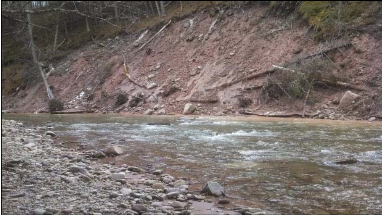
Figure 2. Primary hillslope failure at the West Branch of the Neversink River at Clothes Pool.
