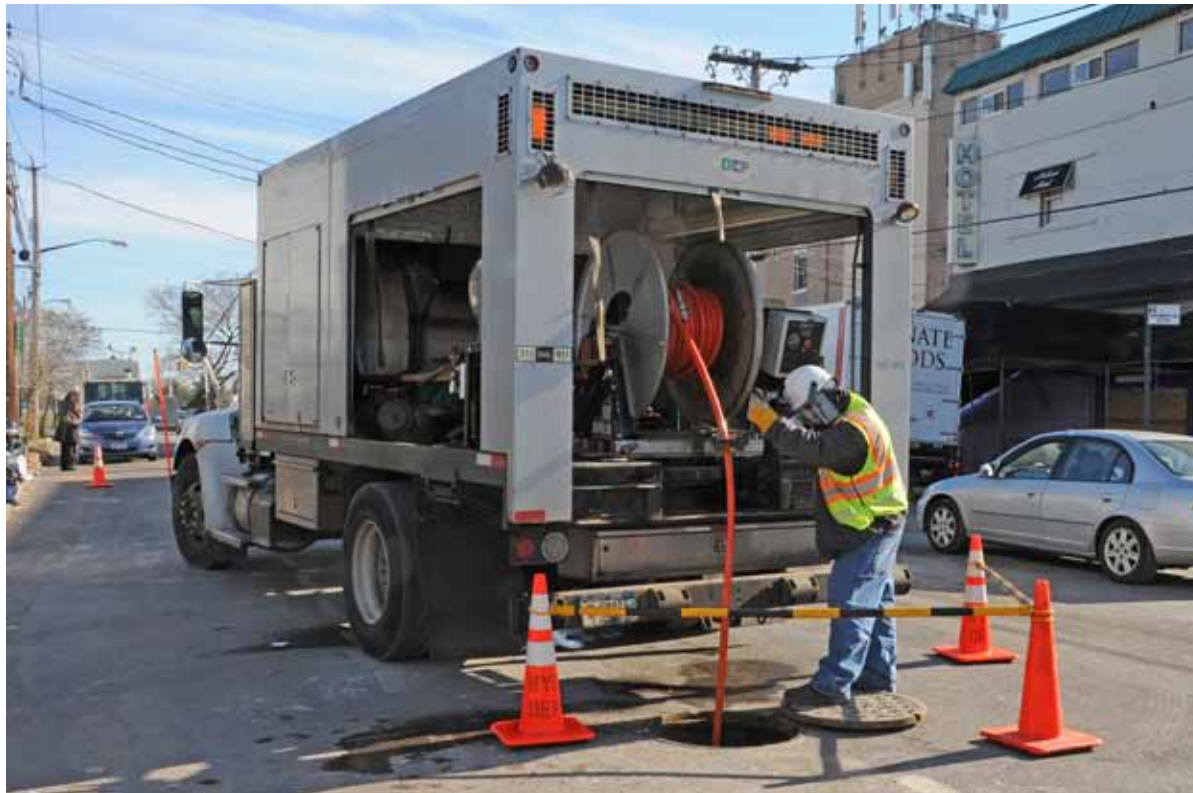
Flushing trucks have large, diesel-powered pumps that force jets of pressurized water into a clogged sewer line, flushing out debris and obstructions. In most cases, when a field crew responds to a sewer backup call, they use these machines to flush the sewer and ensure the line is clean and working properly.
