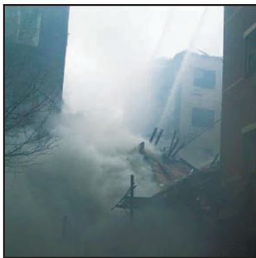
The area of the collapse/debris pile where two victims (the surviving woman is shown above) were found by Rescue 1 members following the March 12, 2014, Manhattan gas explosion/collapse.
