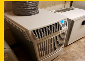
Pace's New HVAC Unit
