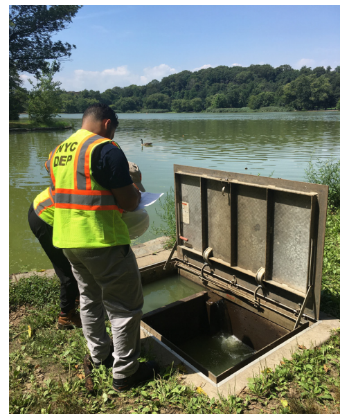
DEP Staff Inspecting Service Line Valve in Prospect Park
