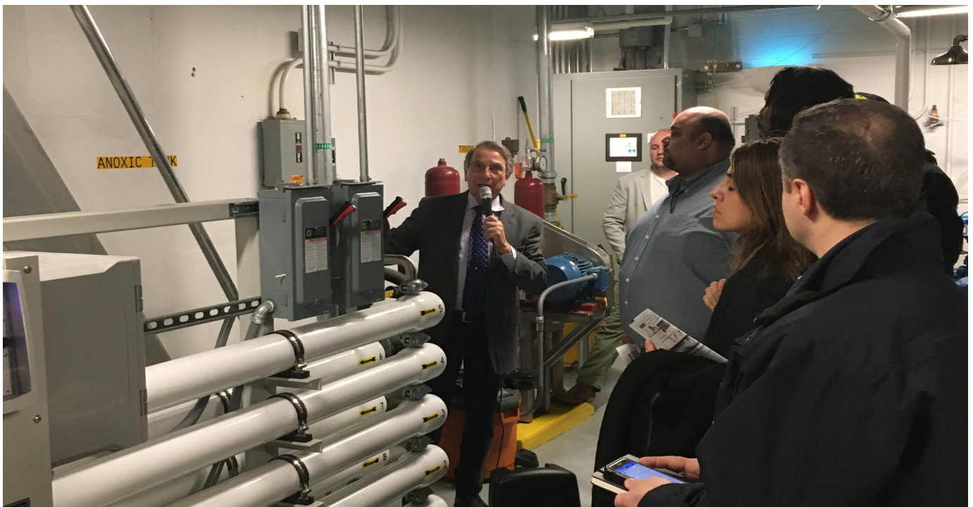
Water Challenge to Universities Workshop, Touring the New School's On-site Water Reuse System
