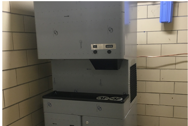
Water Cooled Ice Machines Were Replaced with More Efficient Air-Cooled Models at Harlem Hospital
