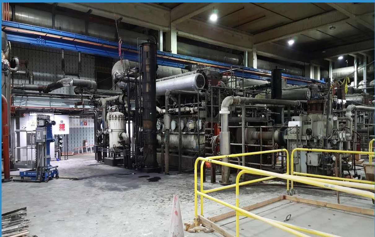
A DEP Wastewater Resource Recovery Facility
