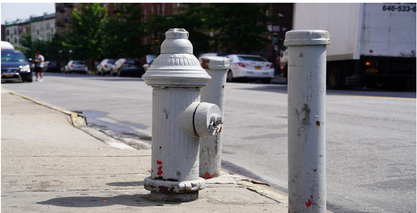
New York City Fire Hydrant
