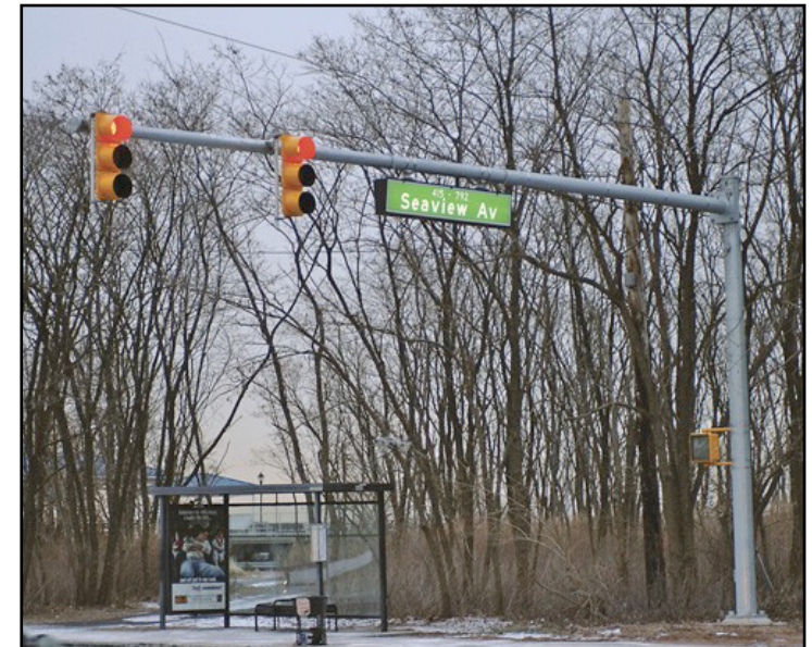
New traffic signal pole with oversized mast arm at Father Capodanno Boulevard and Seaview Ave. In addition, an illuminated street name sign is affixed to the mast arm
