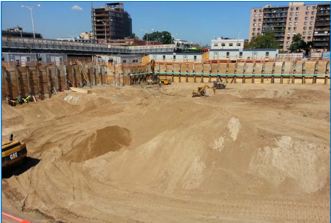
Figure 4: Material made available for reuse through the Clean Soil Bank such as this sandy excavation in Queens has been reviewed by OER and meets the highest remediation standards.
