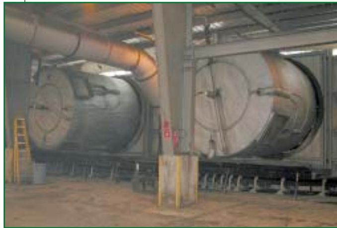
A view inside the building where material is discharged from the composting drum. The conveyor belt under the drum moves the material to a two-inch trommel screen.
