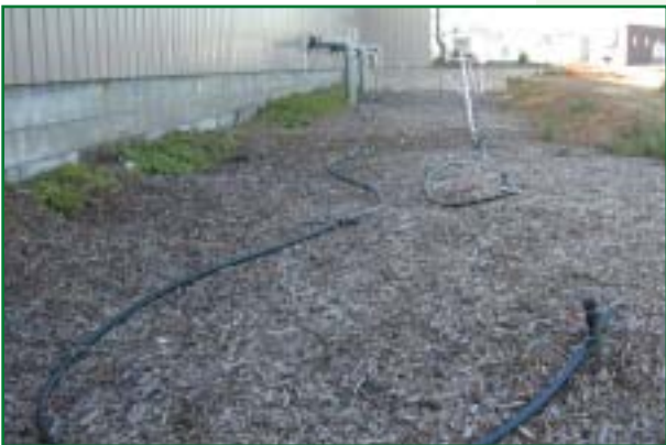
Exhaust air is blown outside the building underground, where it passes up through a biofilter, shown above. Microbes that live in this specially engineered bed of woodchips and compost effectively “scrub” the air of odor-causing compounds. A network of above-ground pipes and sprinklers keeps the biofilter moist.
