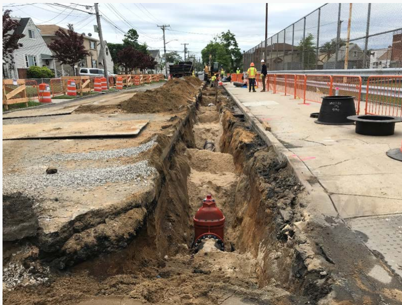
Water main replacement work on 132nd Avenue behind August Martin HS (May 2018)
