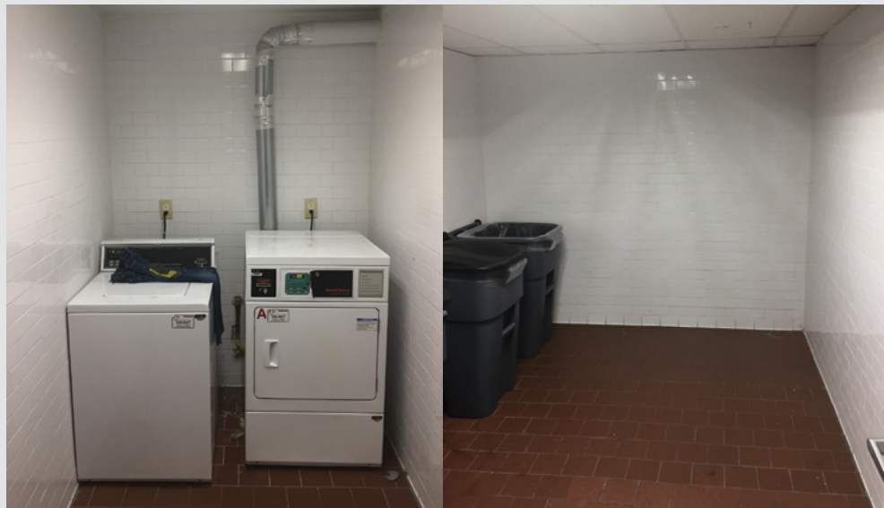
The City’s Shelter Repair Squad retiled the laundry and refuse rooms at the Win Liberty Family Residence.
