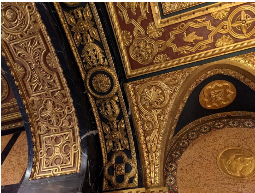
Plaster details Adjacent to East 36th Street steps Matthew A. Postal, November 2021
