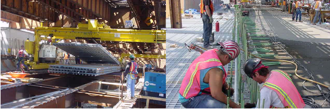
Queens Boulevard - Hoisting a Roadway Grating for Transport & Installing Electrical Conduits in a New Concrete Barrier
