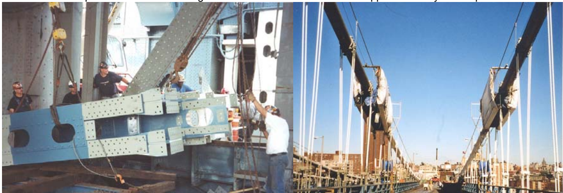
Contract #10 Installing a New End Frame on the Main Span Side of the Brooklyn Tower. Painting Containment Structures on the Cables of the Manhattan Approach Span.
