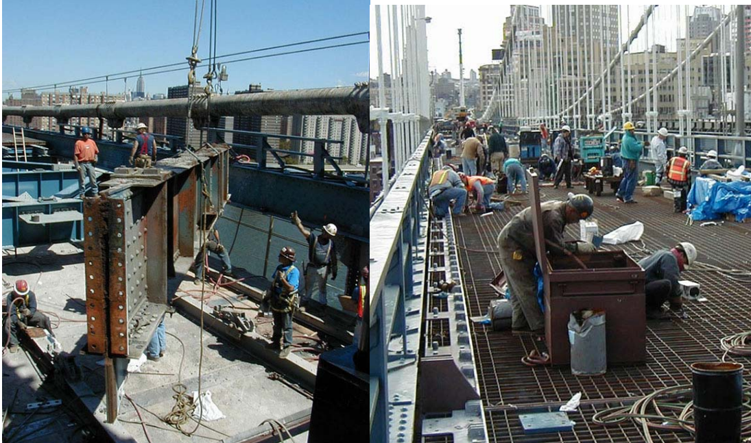
Contract #10 Removing an Existing North Upper Roadway Floorbeam on the Main Span of the Bridge. Installing the New Grid Deck for the North Upper Roadway on the Brooklyn Side Span.
