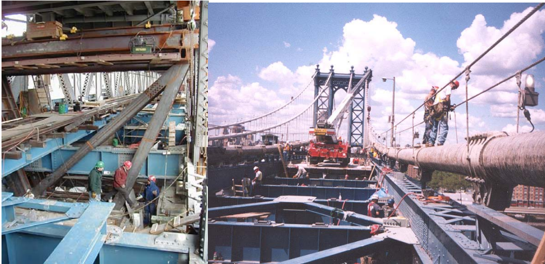
Contract #10 Temporary Truss Jacking Frame Used in the Work to Replace the Existing Truss Bearings. Replacement of Steel Stringers and Floorbeams on the North Upper Roadway Main Span.
