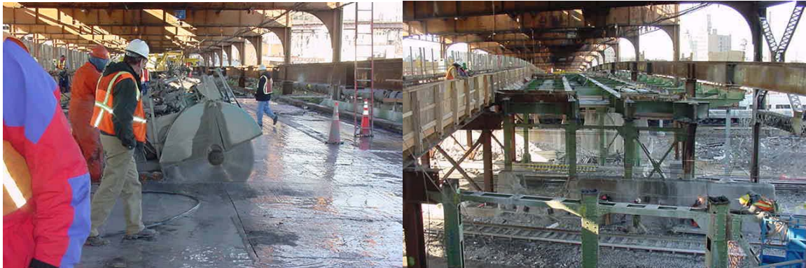
Full Depth Saw Cutting of Queens Boulevard Bridge Deck Slab Panels & Front Steel Demolition
