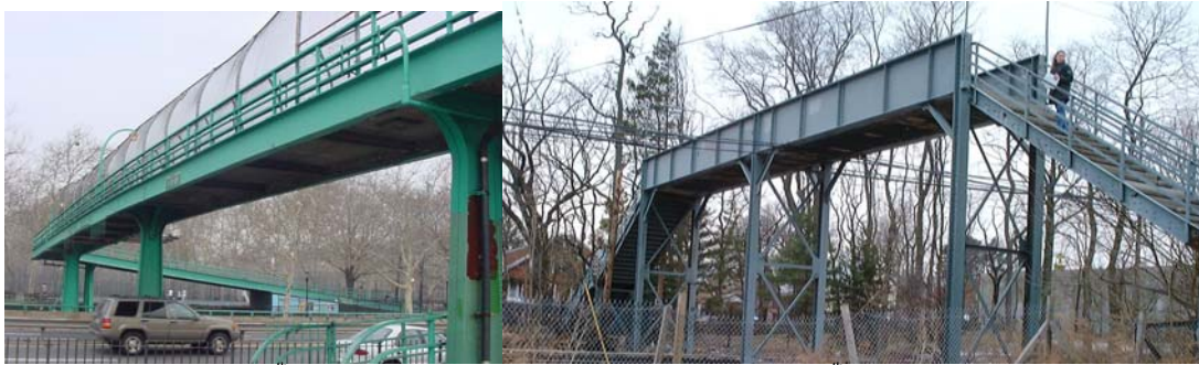
East 111 th Street/FDR Drive (Credit: Andre Celestin) and 216 th Street over LIRR
