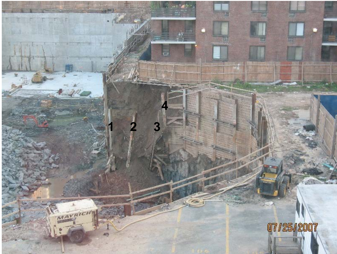
Photo 5 – Collapsed Sheet piling
