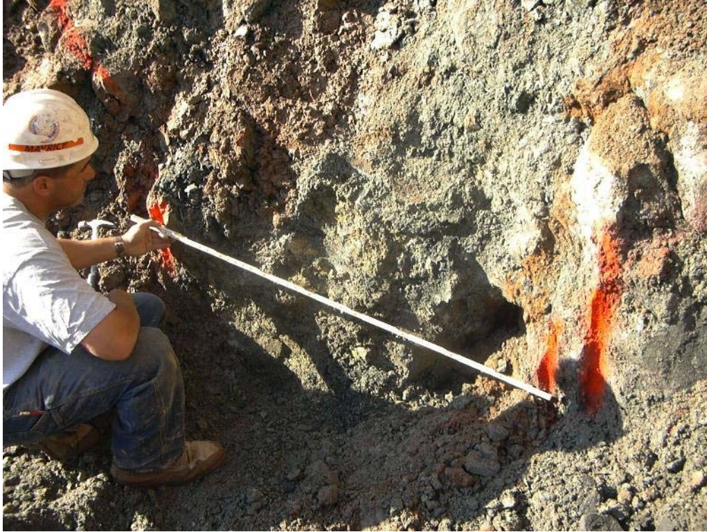
Photo 6 – Weathered Rock Below Sheeting
