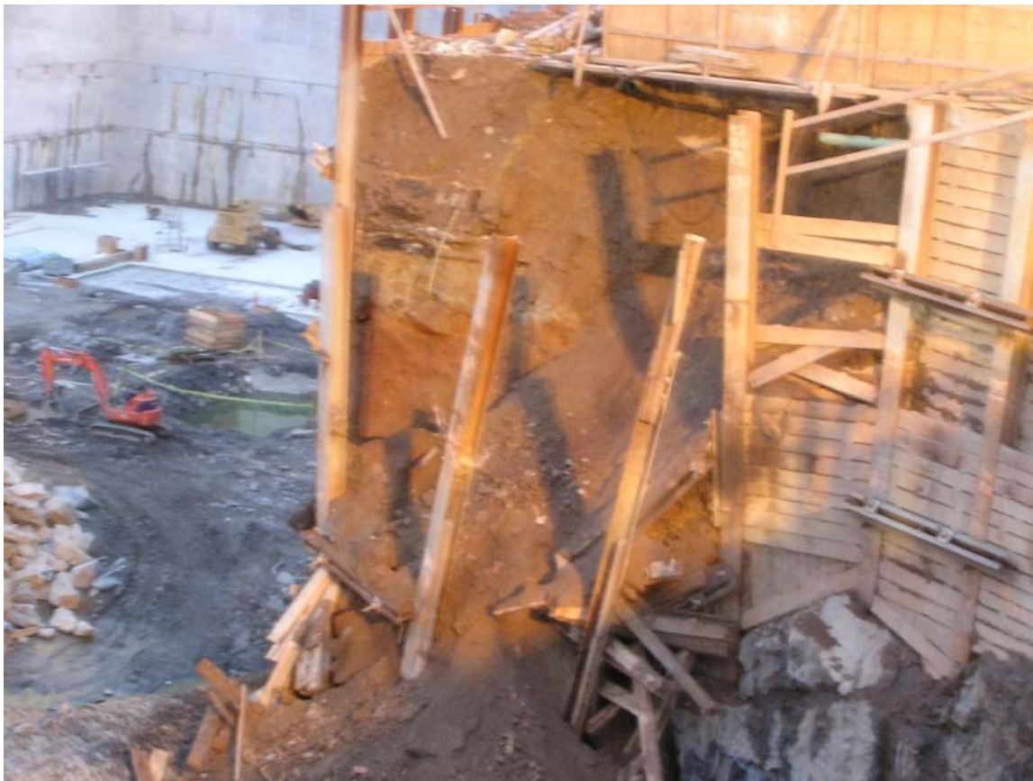
Photo 1 – The Collapsed Sheeting
