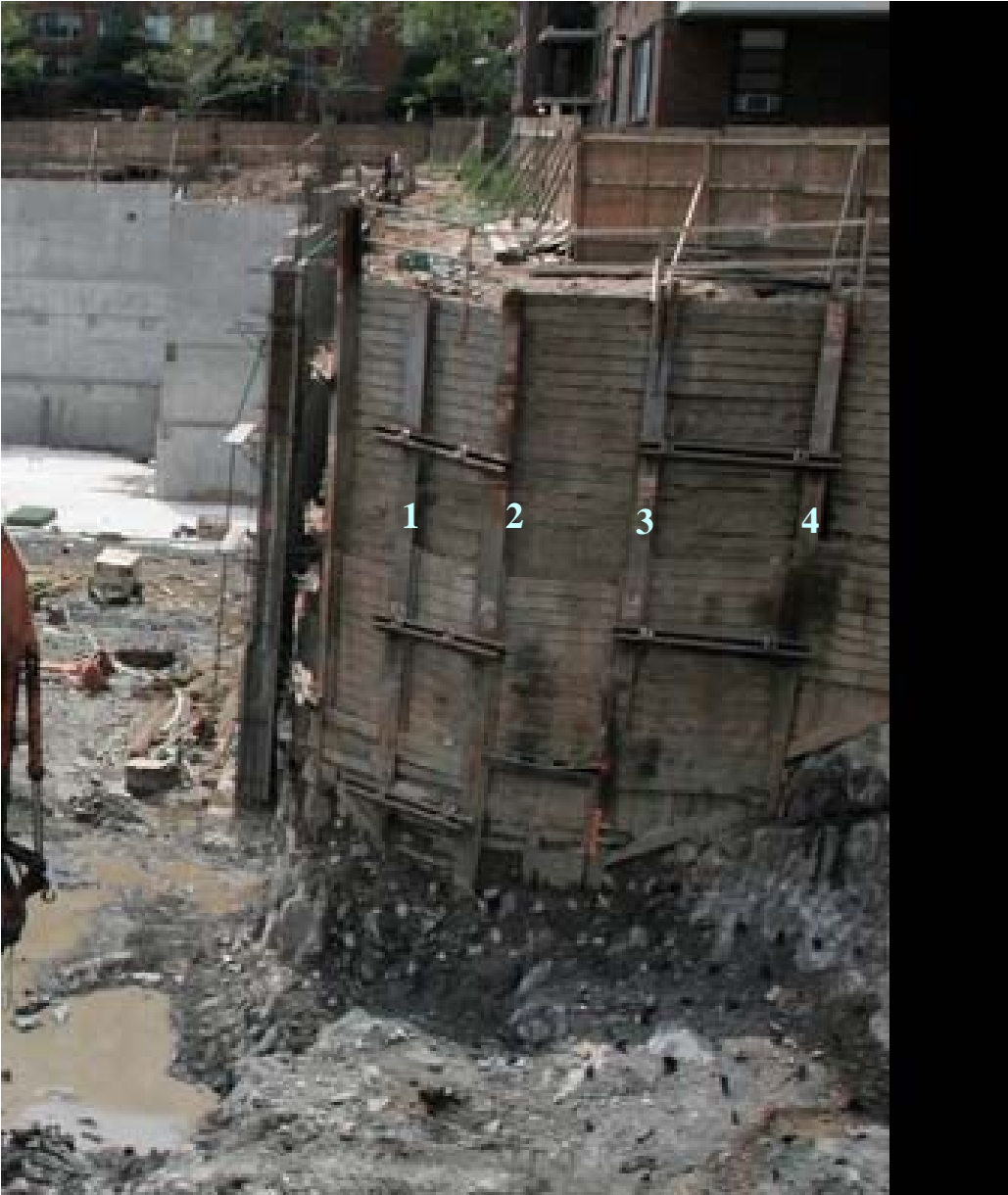
Photo 4 – The Sheet Piling Wall Pre-Collapse –Bernstein photo 7/20/2007
