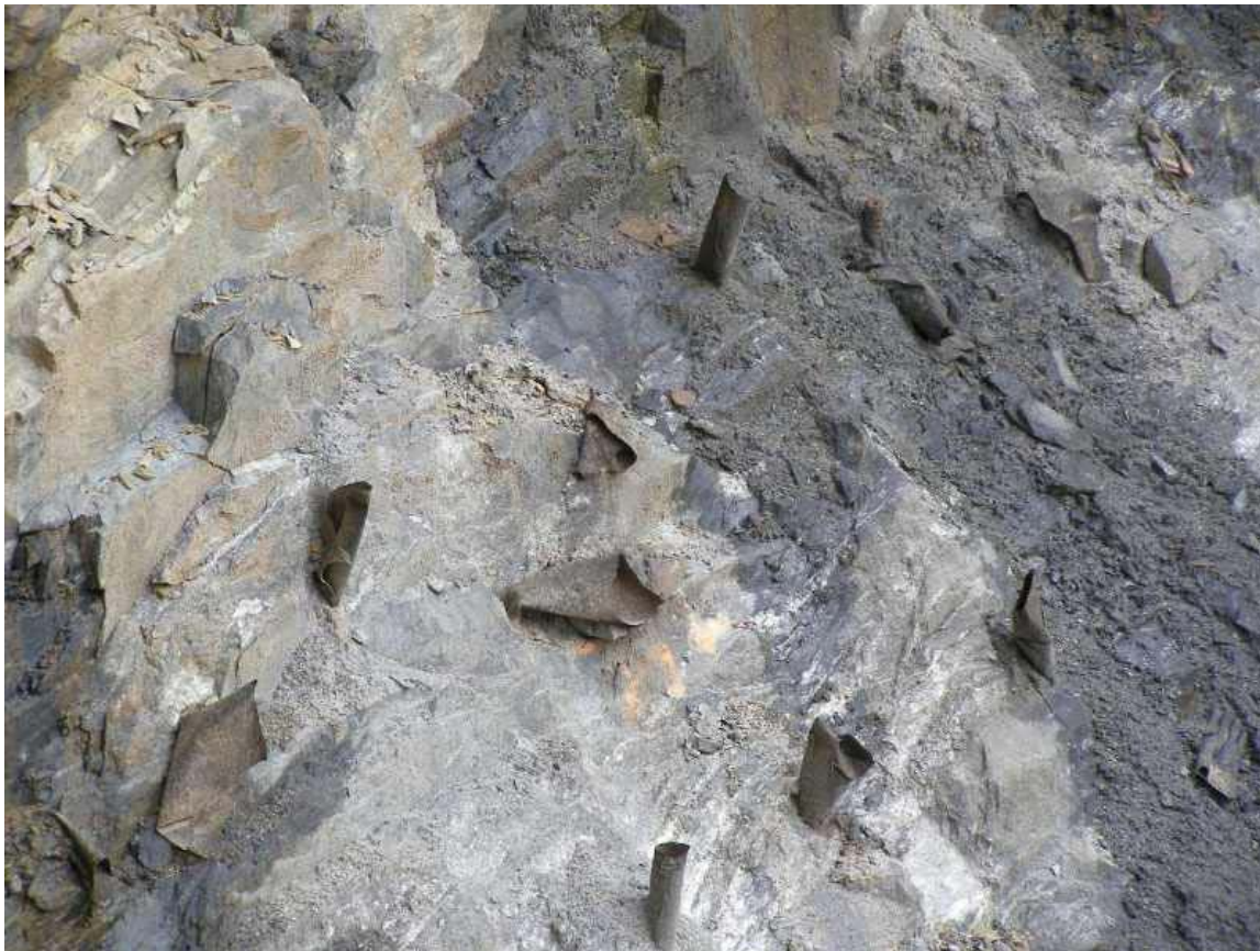
Photo 9 – Marks of Drillings
