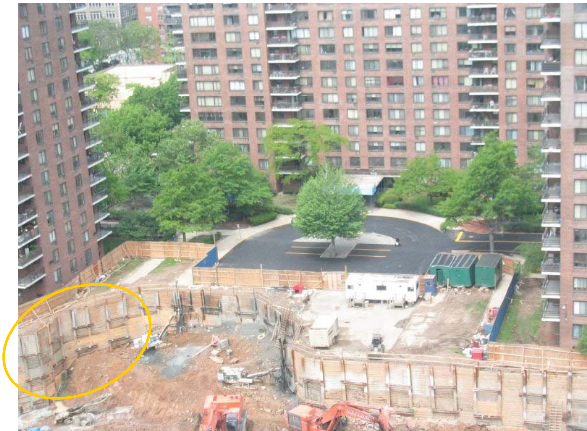
Photo 8 – Area of the Collapse of the Sheet piling Is Marked
