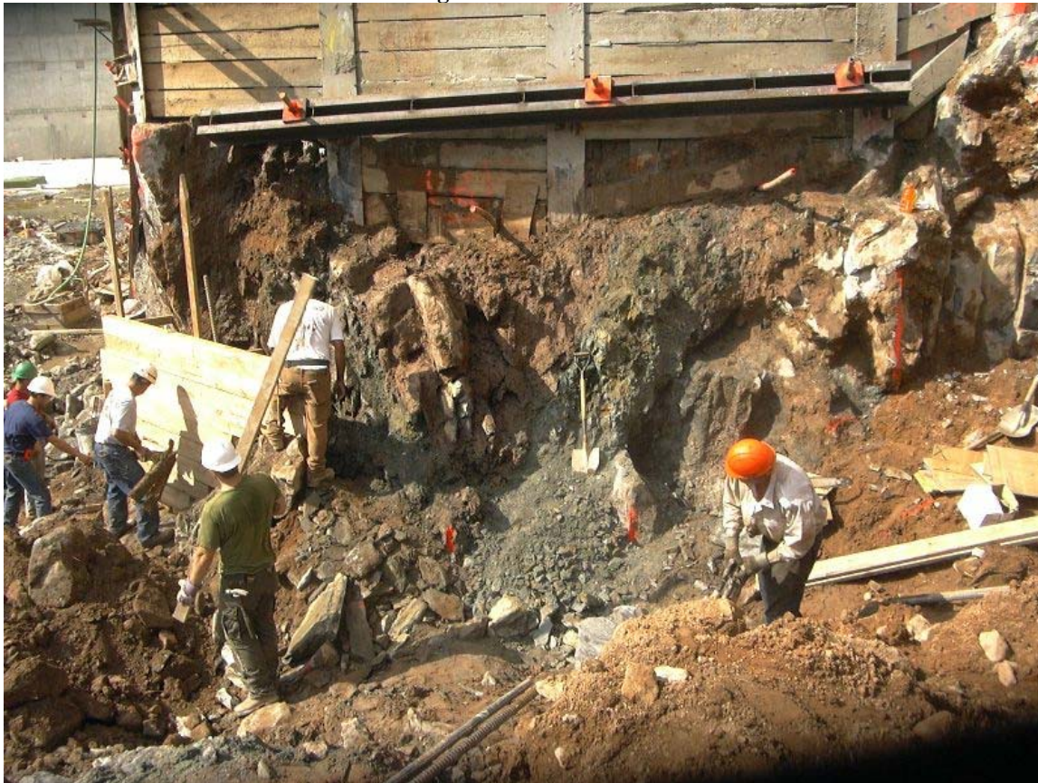
Photo 7 New Sheeting Installed Several Feet Away From Original. Note Weathered Condition of Rock
