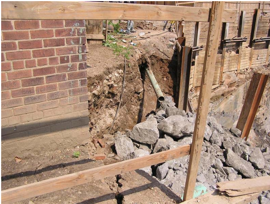
Photo 11 – Broken drainage pipe at collapse area
