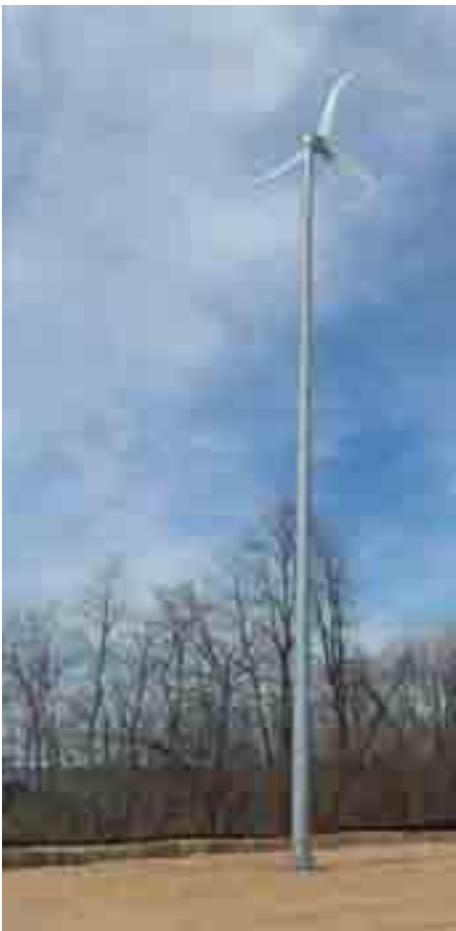
Wind turbine at the Tides at Charleston, Staten Island.
