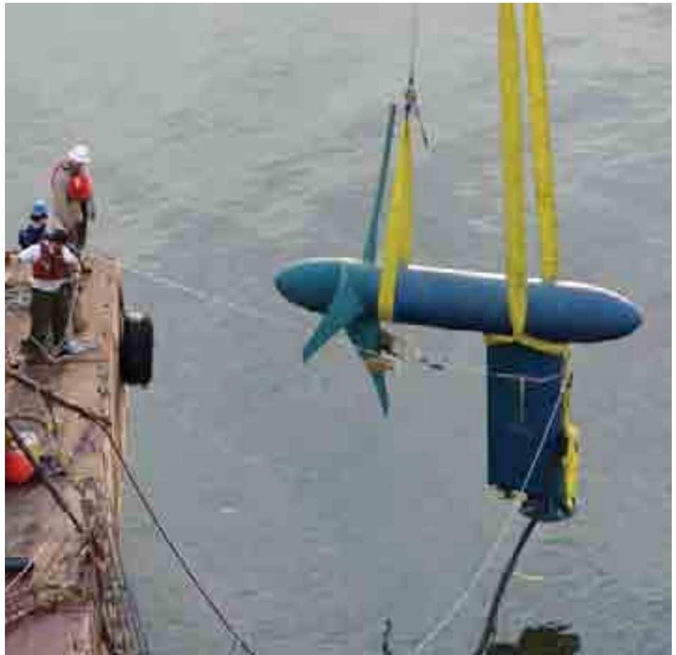
Installation of Verdant Power tidal turbines in the east channel of the East River.
