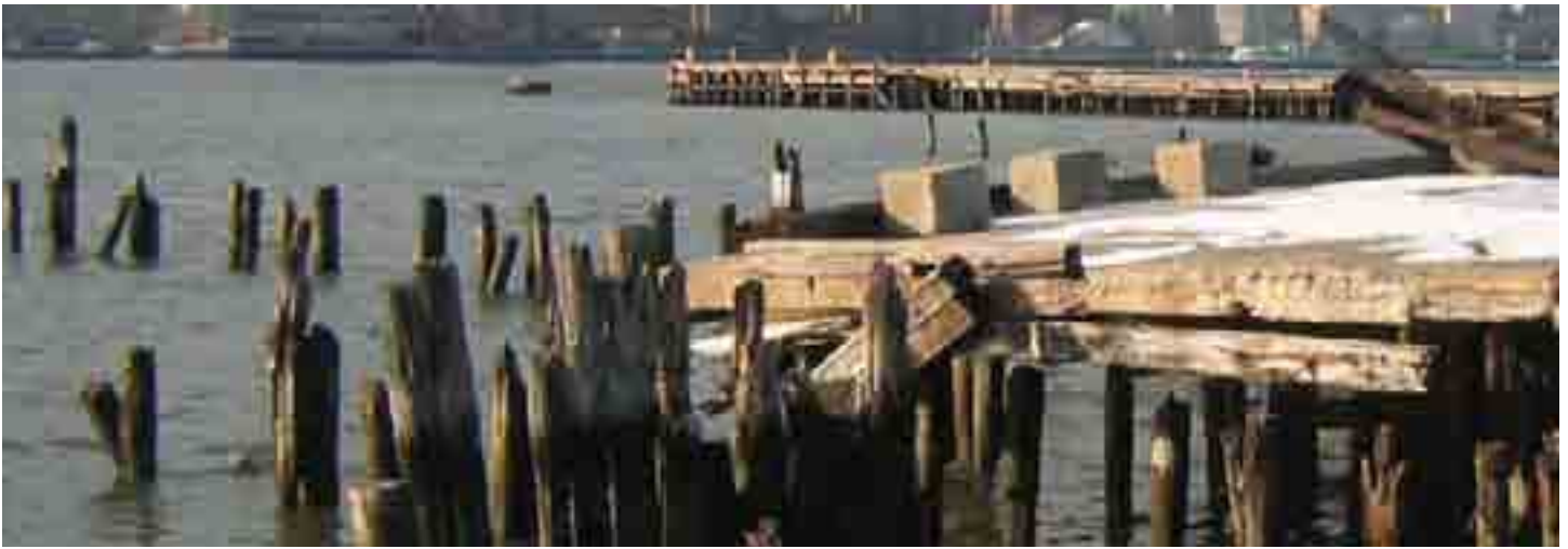
Without regular maintenance, piers will deteriorate until they collapse, as seen with this pier in Greenpoint, Brooklyn. It is difficult to obtain a permit to rebuild.
