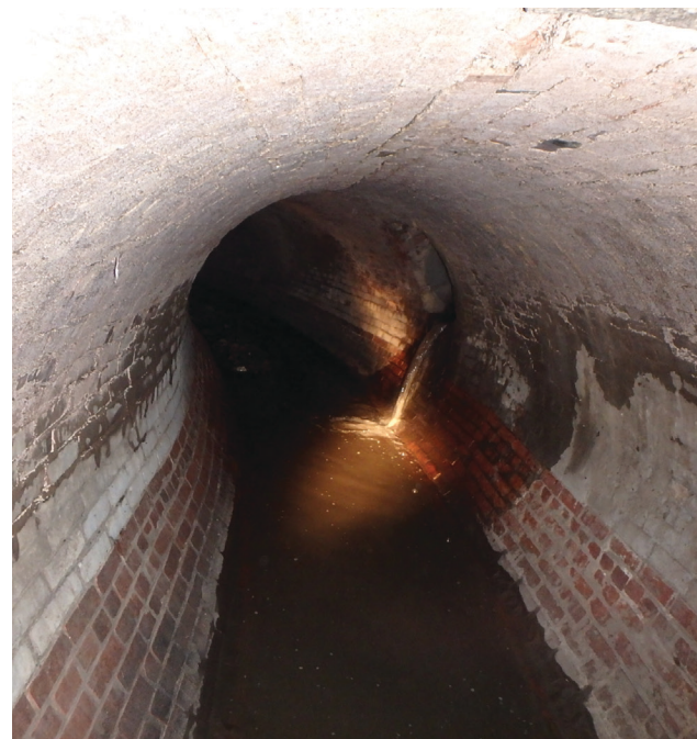
Stormwater discharging through MS4
