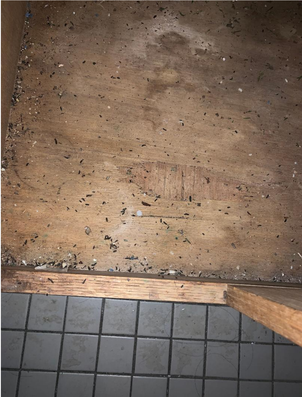
Photo 7 - Kitchen Cabinet Filled with Mouse Droppings
