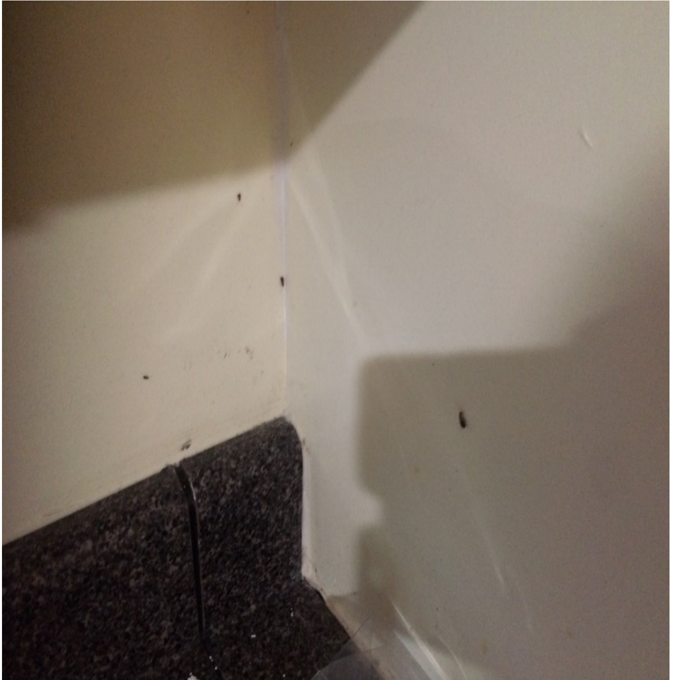
Photo 8 - Roaches Crawling on Kitchen Wall
