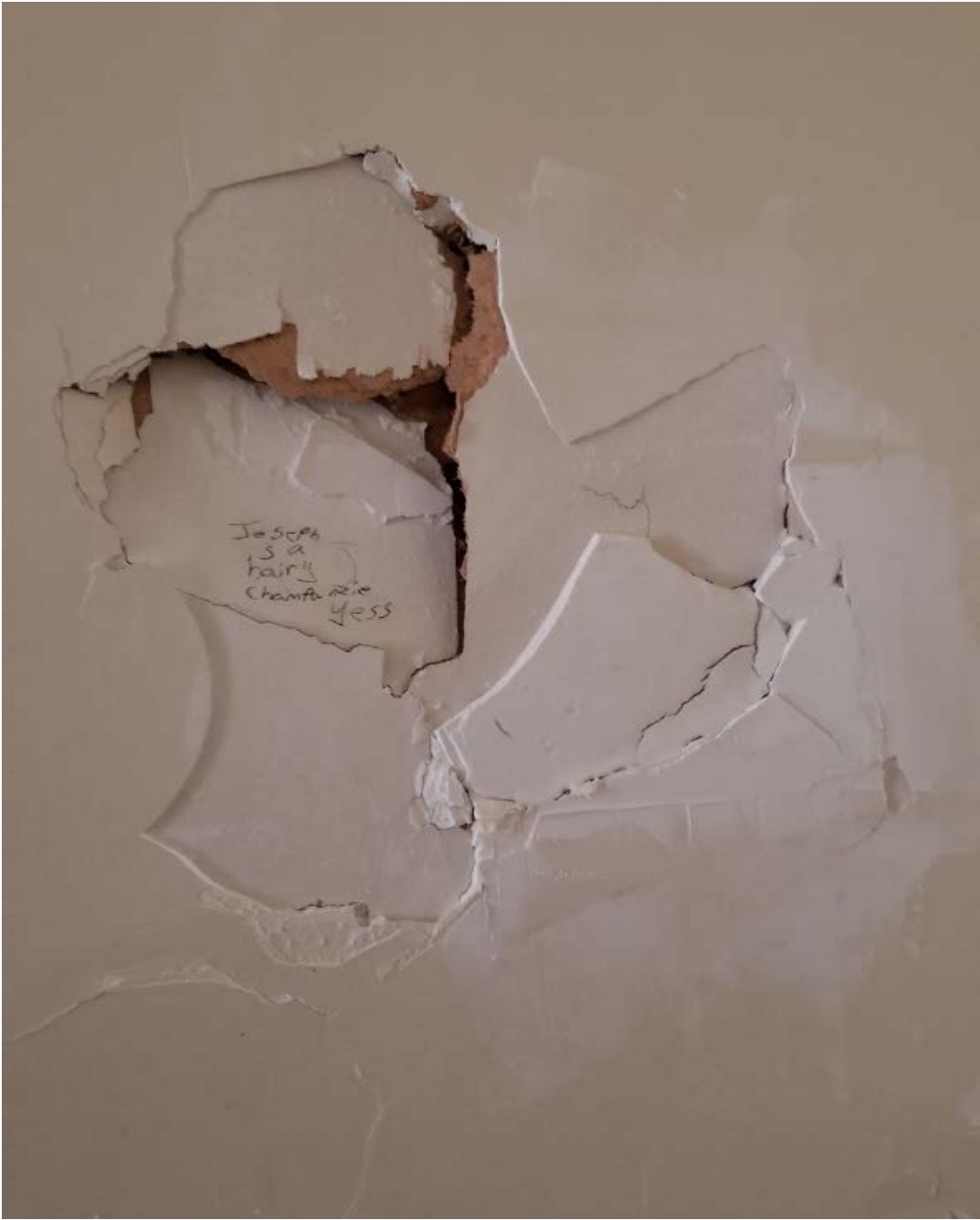
Photo 10 - Hole in Bedroom Door
