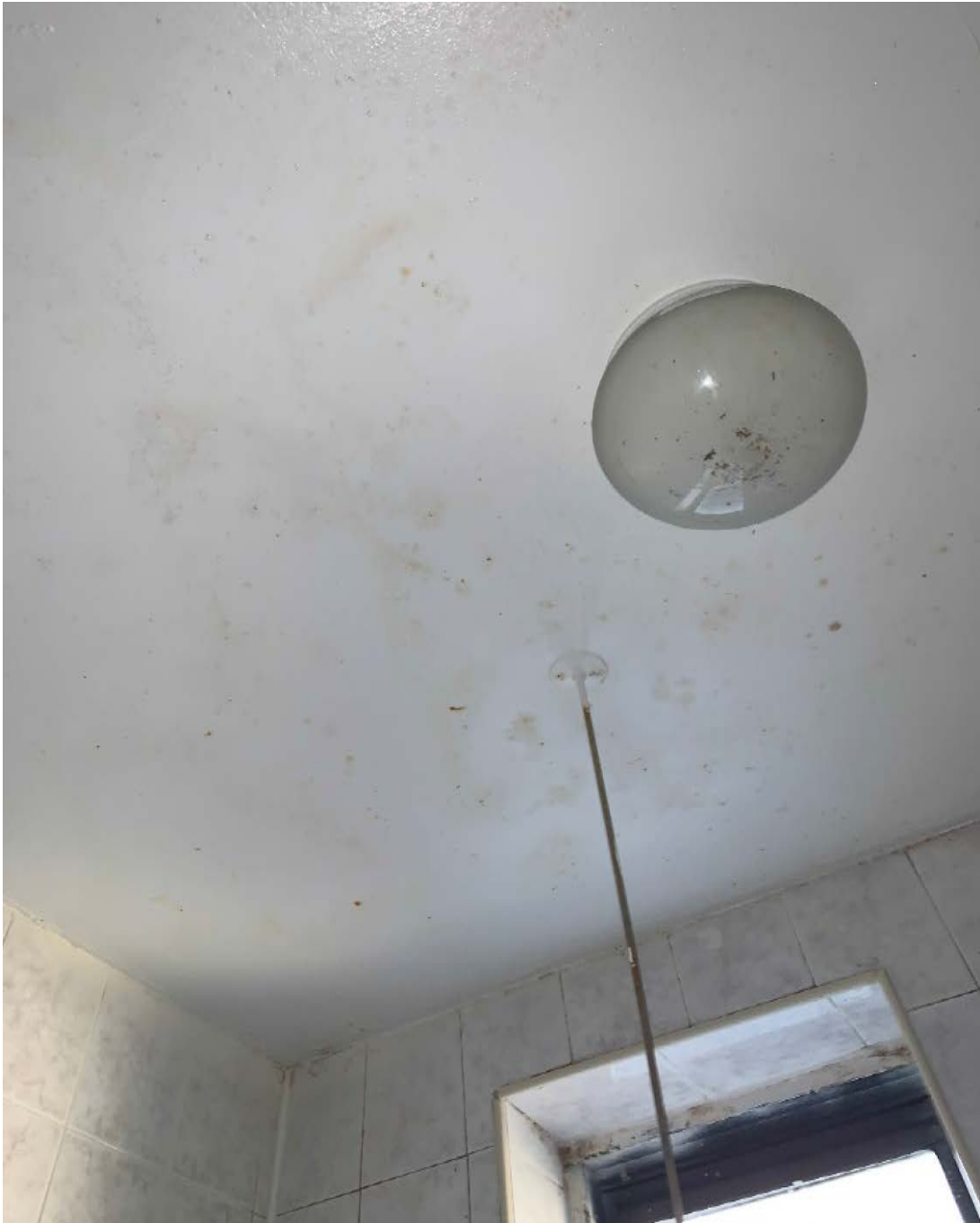
Photo 6 - Mold and Mildew on Ceiling
