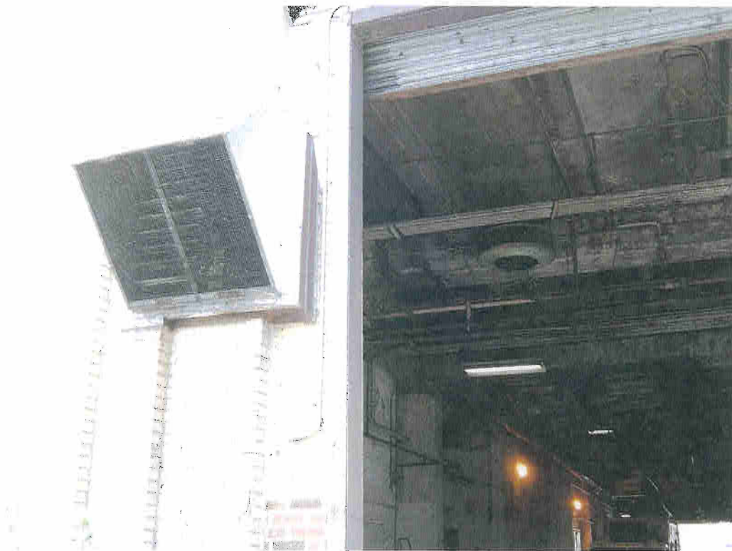
Outside view of exhaust vent
