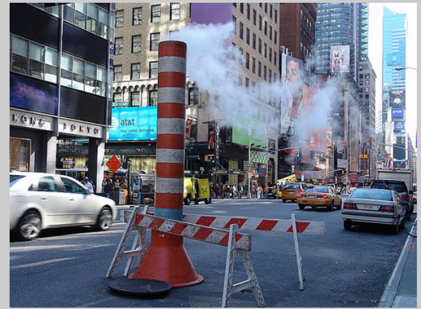
A steam leak on Broadway is contained by Con Edison and blocked off.
