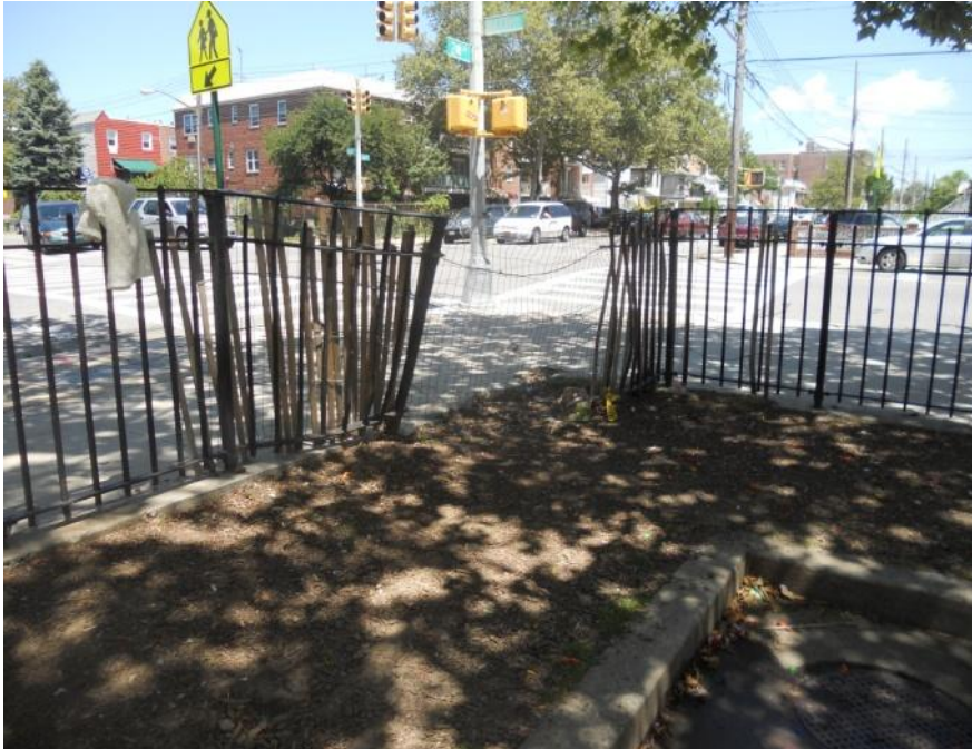
7. Bath Playground Damaged fence
