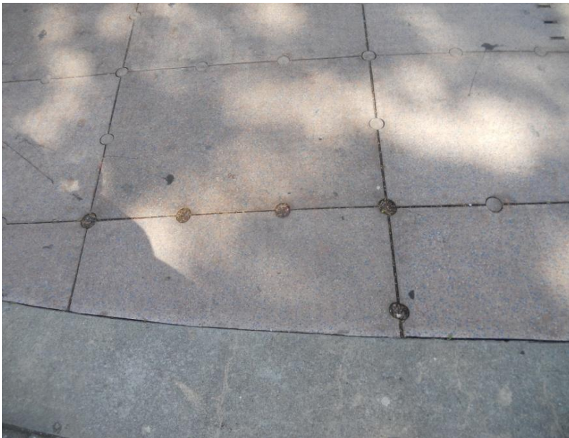
16. Tiger Playground Missing plugs on mats
