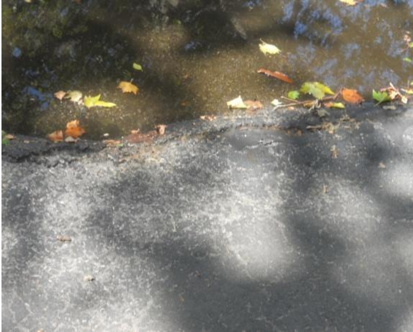
15. Sperandeo Brothers Playground Cracked pavement
