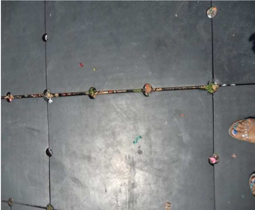
11. Surf Playground Mat area has missing plugs
