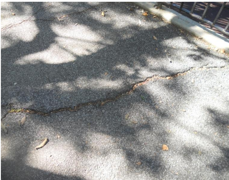
12. Century Playground Cracked pavement
