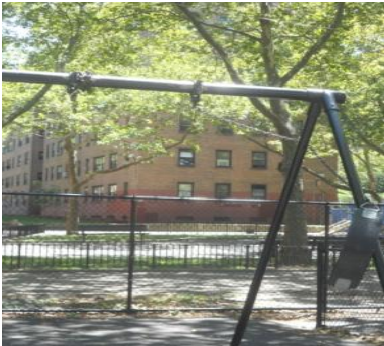
10. Marlboro Playground Broken swing
