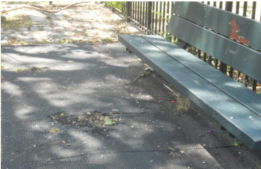
6. Scarangella Playground Peeling paint on benches and weeds on ground
