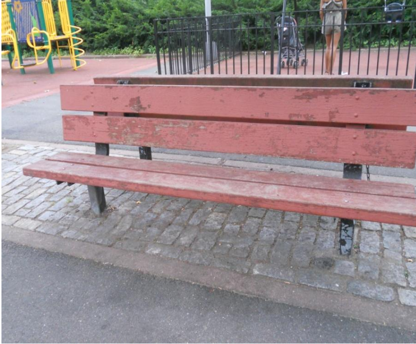
13. Crispus Attucks Playground Peeling paint on benches
