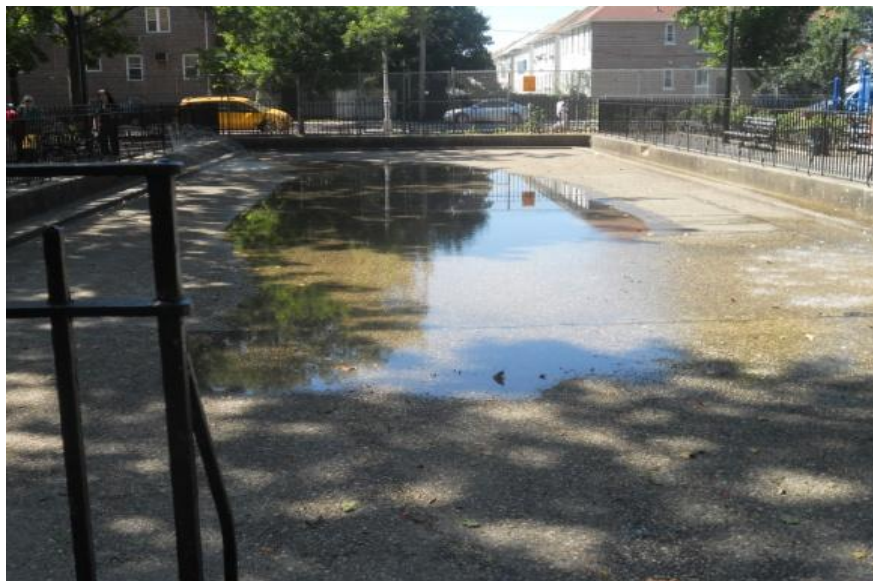
1. Bill Brown Playground Standing water at sprinkler area
