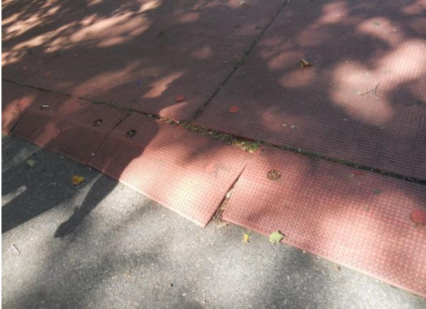
5. Homecrest Playground Broken mats
