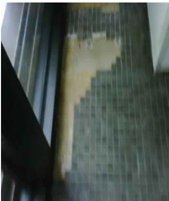
Missing floor tiles
