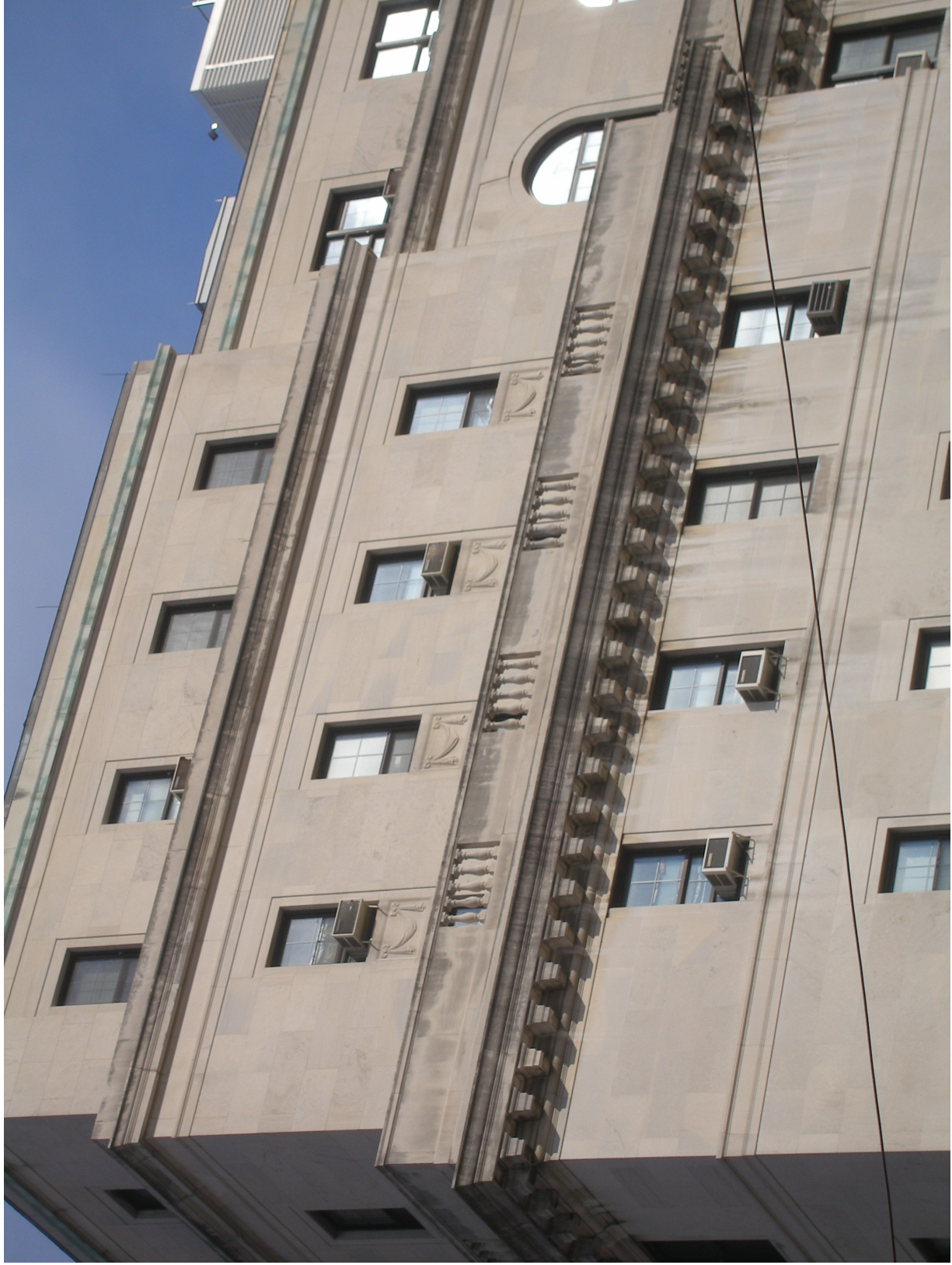
Queens General Court House Detail of the upper stories, Sutherland Avenue facade Photo: Christopher D. Brazeel, January 2007
