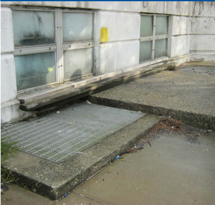
Grate and windows leading to the basement of the Sludge Thickener Building and tunnel system
