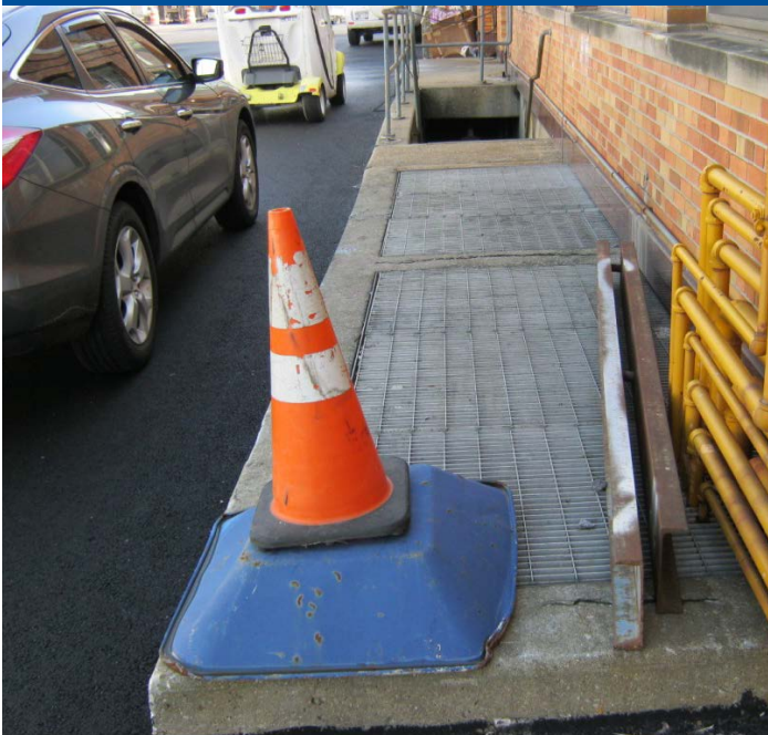
Basement access and floor grates on the perimeter of the Main Building
