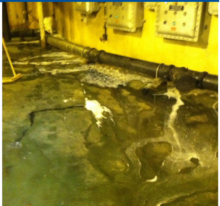
Sinkholes developed near the Sludge Storage Area after Hurricane Sandy. Groundwater may present a flood risk during the next critical flood event
