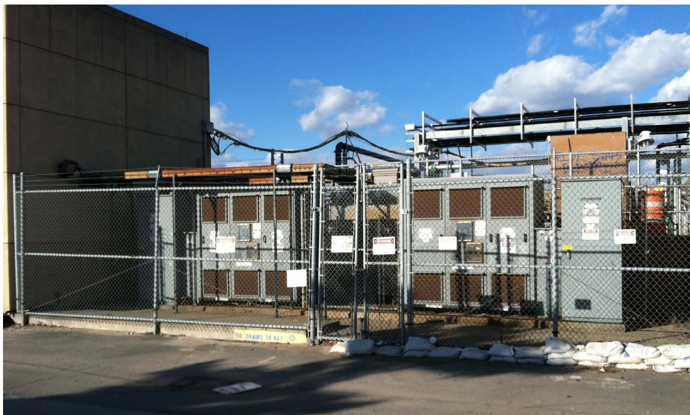
The Unit Substation (USS 1533) is currently protected with sandbags.
