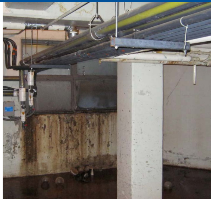
A window at the Sludge Storage Building was one of the main areaways for floodwater to enter during Hurricane Sandy.
