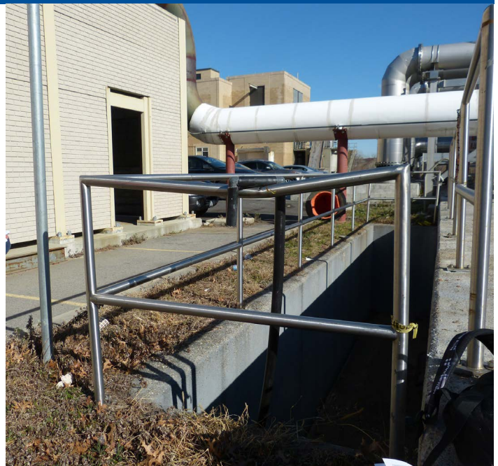
A basement access way leading to the Primary Sludge Gallery would be a flood pathway during the critical flood event.
