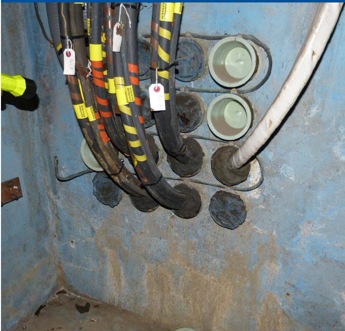
Electrical conduits in the basement of the Main Building provided a pathway for floodwaters during Hurricane Sandy.
