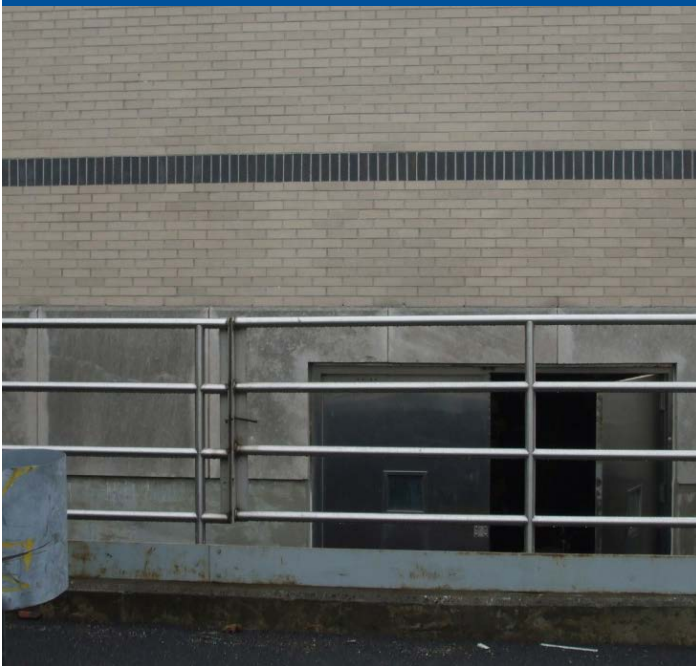
A pathway for flooding is around the perimeter of the Administration Building.
