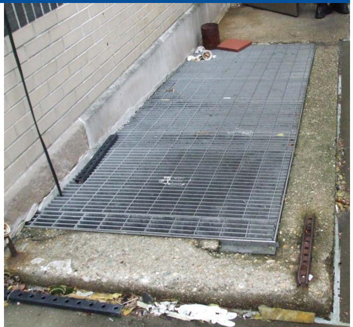
Floor grates near the Generator Room may allow floodwater to enter.
