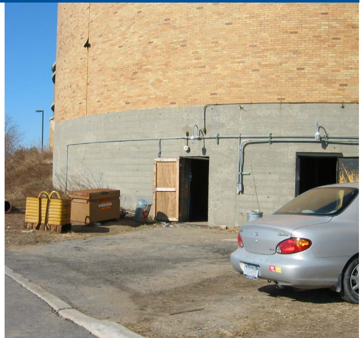
Access doors to the Sludge Storage Tanks next to the East River
