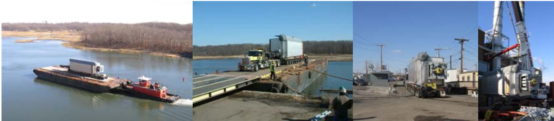
In February 2007, a Permit Was Issued for the Move of a Boiler to Co-op City in the Bronx. The Boiler was Unloaded From a Barge at the Agency Conner Street Facility, and Was Later Delivered by Truck to Its Final Destination. The Total Weight of the Vehicle With the Boiler was Approximately 380,000 Pounds.
