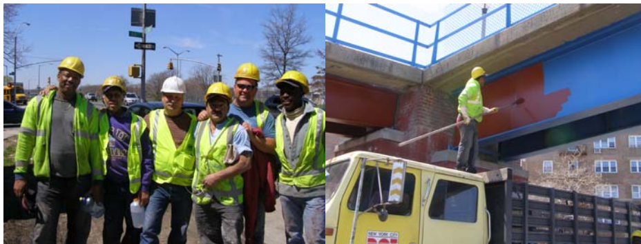
Bridge Painters Reynaldo Grant, Joao Silva, Robert Avellino, Louis Masucci, Brian Kavanagh, and Joao Nascimento at the Whitelaw Pedestrian Bridge. Bridge Painter Reynaldo Grant. (Credit: Earlene Powell)
