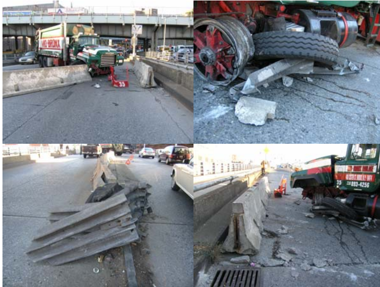
Damaged Truck, Jersey Barriers, And Impact Attenuator.
