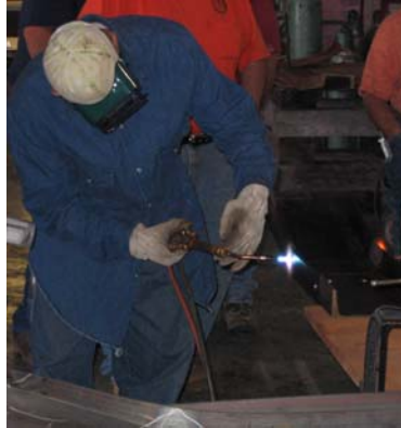
Bridge Repairer and Riveter David Collins Demonstrating Heat Straightening Techniques. (Credit: George Klein)
