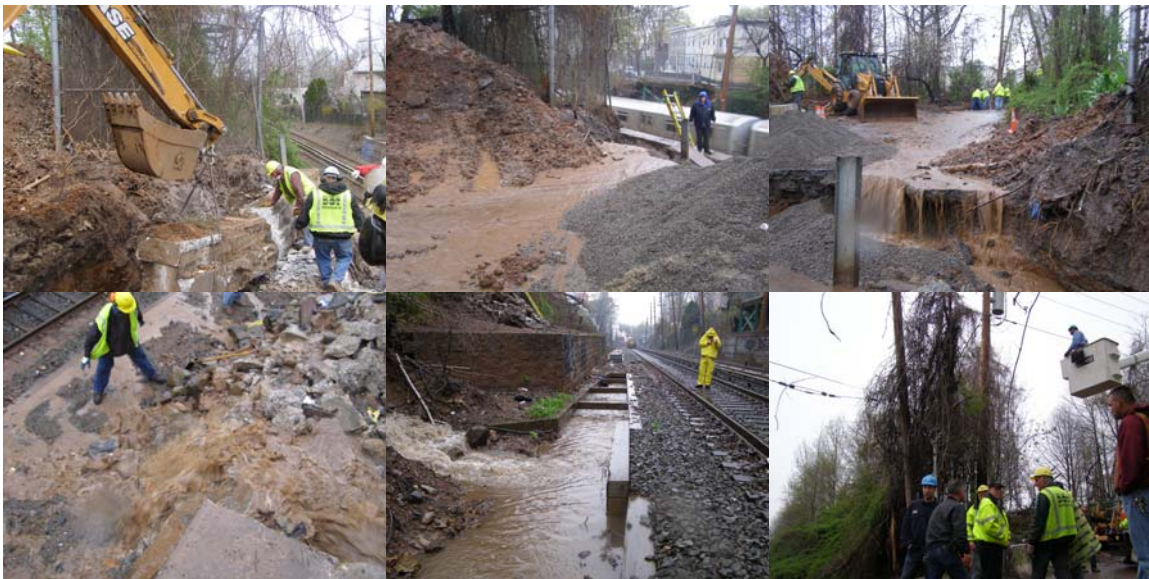
Department and Consolidated Edison Personnel at the Former Bridge Site. Executive Director of Bridge Preventive Maintenance and Repair Thomas Whitehouse (Fourth From Left, in Last Photo.)
