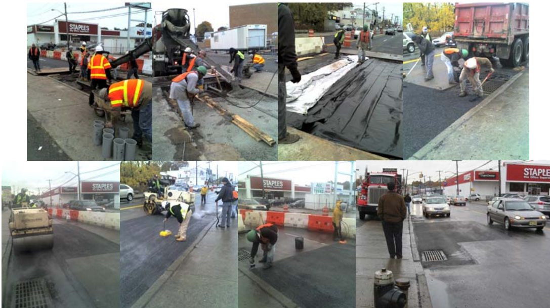
Completing the Forest Avenue Culvert Repairs: Asphalt was Placed in Two Layers; Compacted With a 5-Ton Vibratory Roller; the Asphalt Joints Were Sealed; Nuclear Compaction Tests Were Performed; and All Forms Were Removed From the Underside of the Culvert. Completed Repair.
