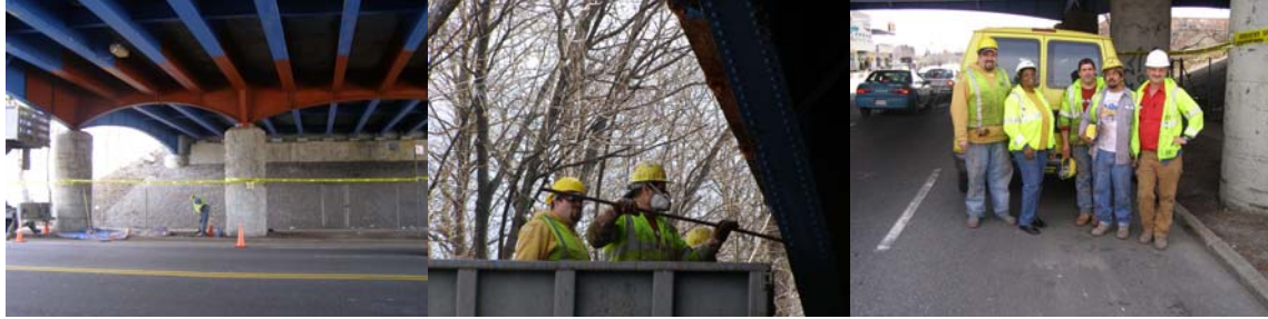
Painting the Belt Parkway Over Ocean Avenue Bridge. (Credit: Earlene Powell) Bridge Painter Brian Casey, Deputy Director of In-House Painting Earlene Powell, Bridge Painters Anthony Attore and Samuel Martinez, and Supervisor Bridge Painter David Yanolatus.
