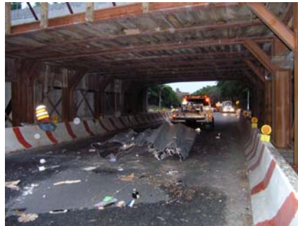
Debris Under the West 252 nd Street Bridge Construction Shield After Accident. (Credit: Mohammad Awal)
