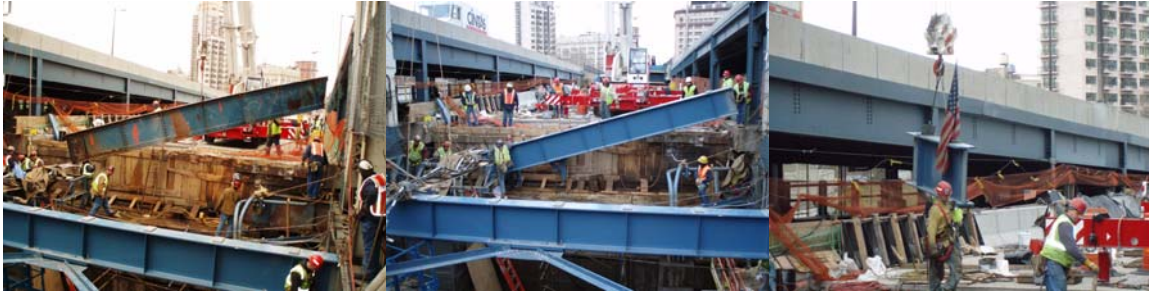
Removal and Replacement of the Final Existing Manhattan Bridge Lower Roadway Floorbeam.
