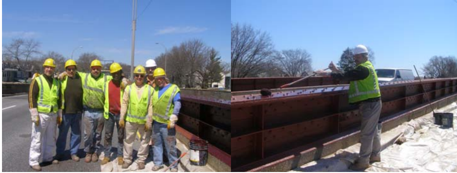
Bridge Painters Frank Hollen, Albert Pappas, Nicholas Krevatas, Henry Bollin, and Branko Grzanic, Supervisor Bridge Painter Georgeios Ploumis, and Bridge Painter Brain Kenny at the Woodhaven Boulevard Bridge. Supervisor Bridge Painter Georgeios Ploumis. (Credit: Earlene Powell)
