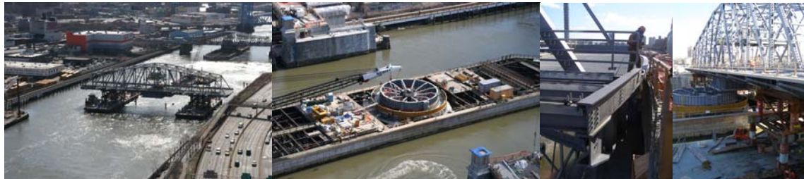
Floating In the New 145th Street Span in February 2007. (Close-up Credit: Bojidar Yanev)
