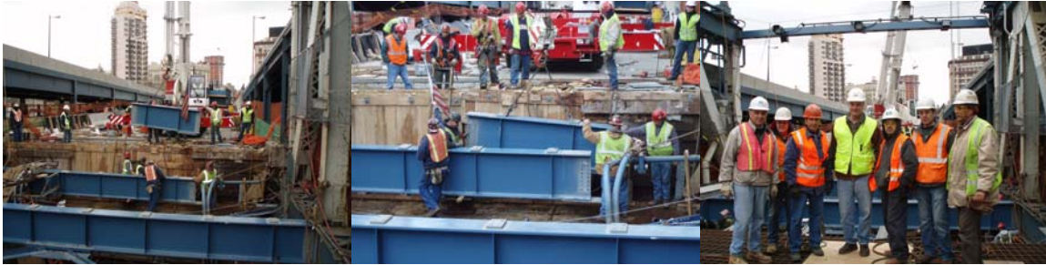
Placing the Final Floorbeam Into Position. Engineer-In-Charge Brian Gill (in Center) and Inspection Staff on the Lower Roadway.
