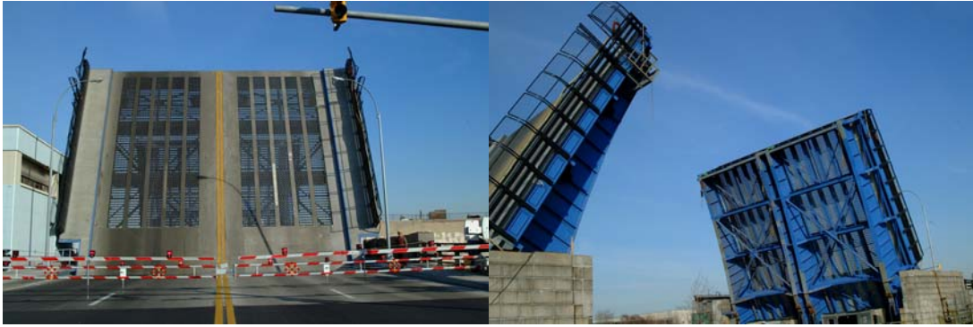
Bridge Opening With New Machinery And New Warning And Safety Gates.
