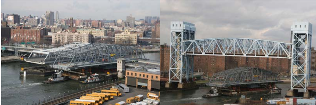
Moving the New 145 th Street Swing Span From South of the Third Avenue Bridge to the Site. Passing Under a Metro-North Railroad Bridge.
