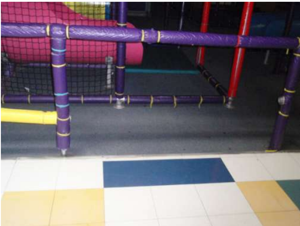
Missing Bar of Indoor Jungle Gym
