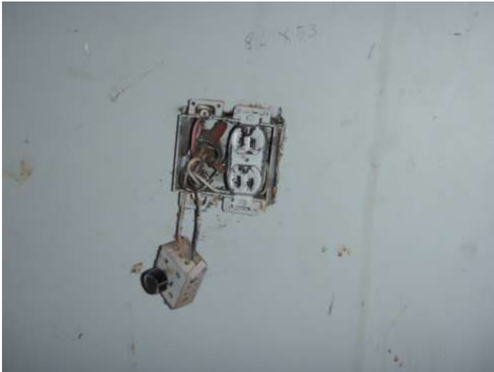
Exposed Electrical Outlet
