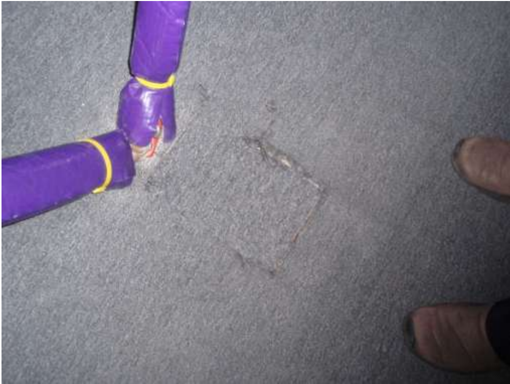
Damaged Carpeting in Gymnastics Area
