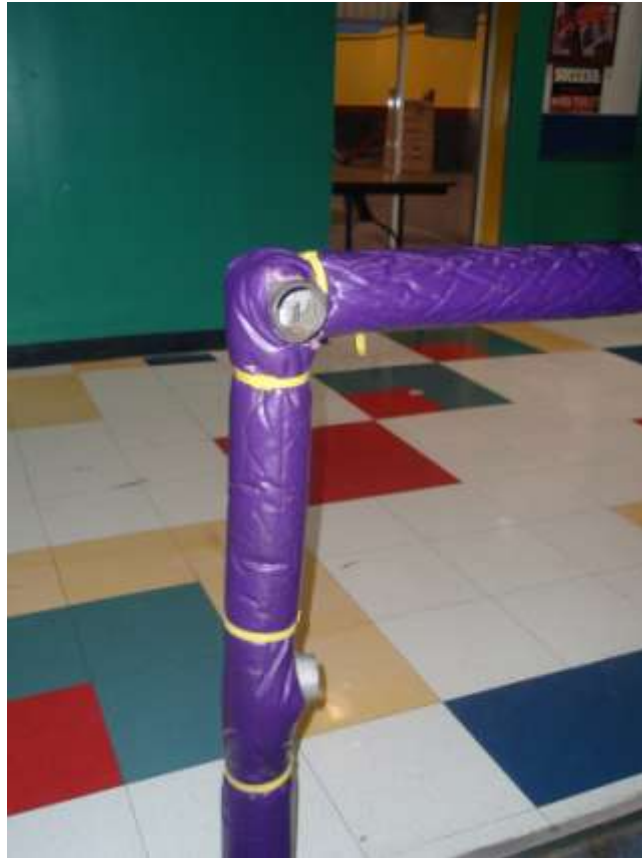
Exposed Metal Edges
