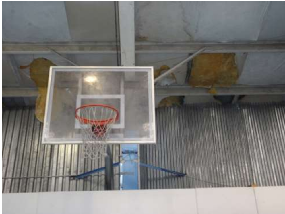
Damaged Ceiling Panels at Basketball Court near Soccer Field
