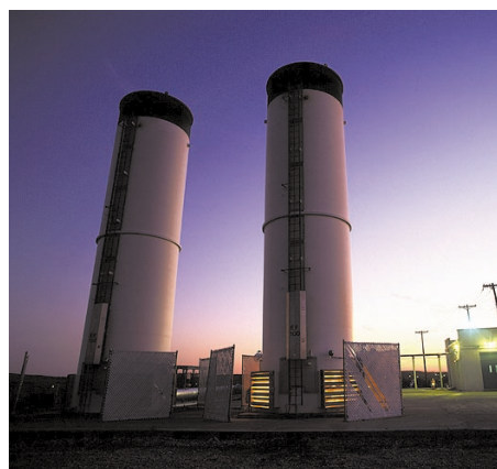
Methane flaring station at sunset.
