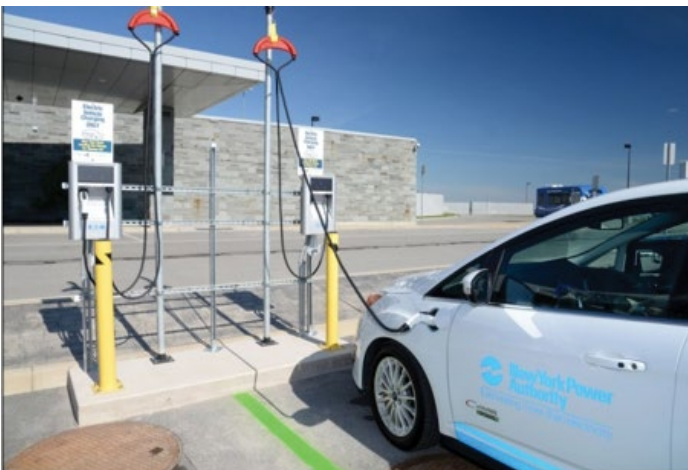
A car charges with a Level 2 Charger.
