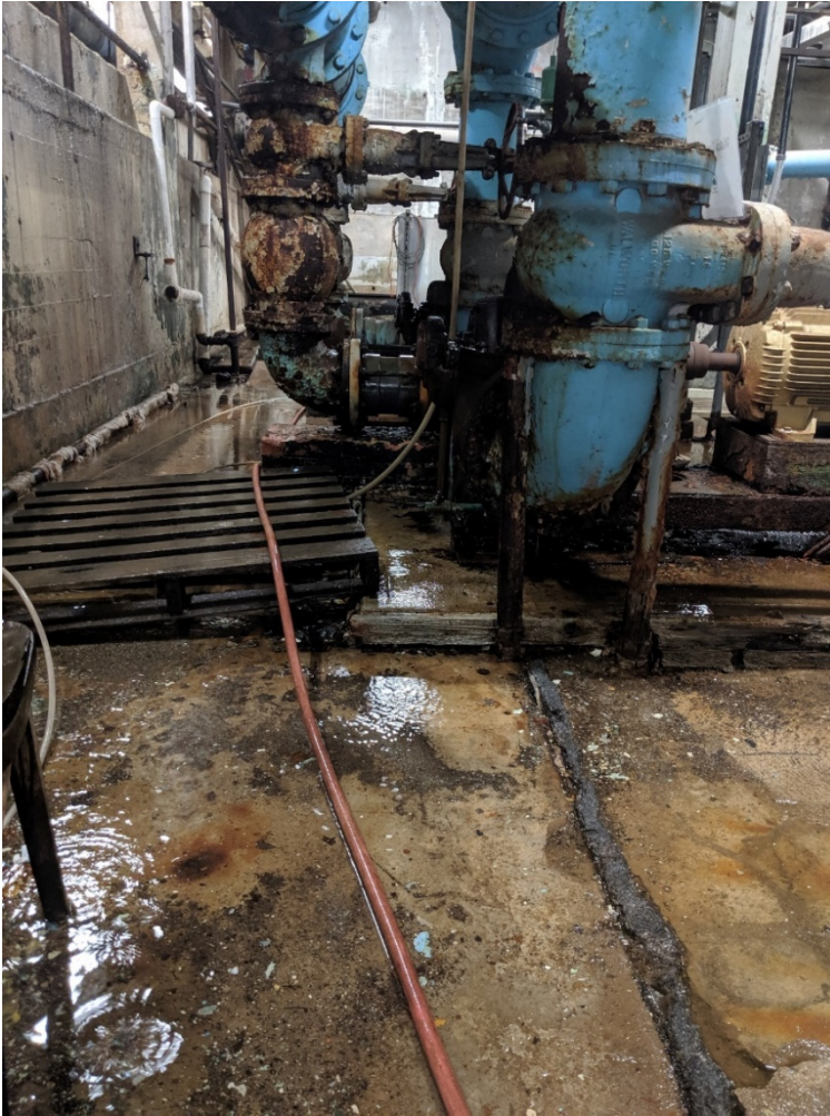
Image 1: Showing extensive flooding in Filter Plant underneath Circulation Pipes.
