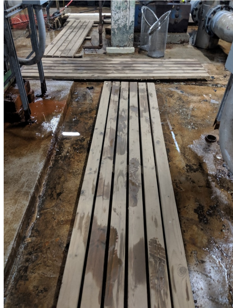
Image 2: Showing makeshift walkway laid on top of flooded areas.
