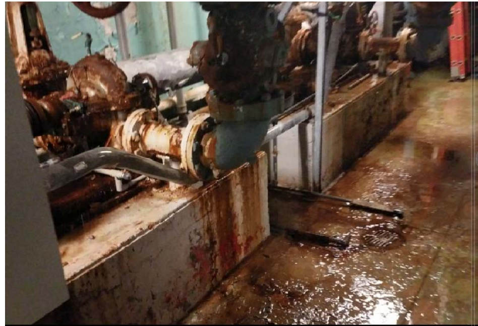
Image 2: Area around recirculation pumps #2 and #1 showing leaks and corrosion on September 5, 2019.
