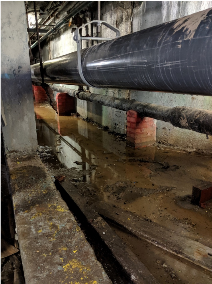
Image 1: Standing water underneath pool area on August 12, 2019.
