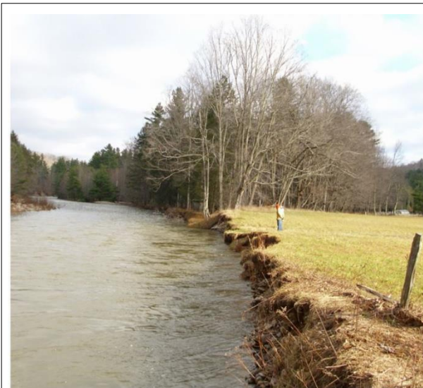
Figure 4.22 Eroding streambank before bioengineering treatment.
