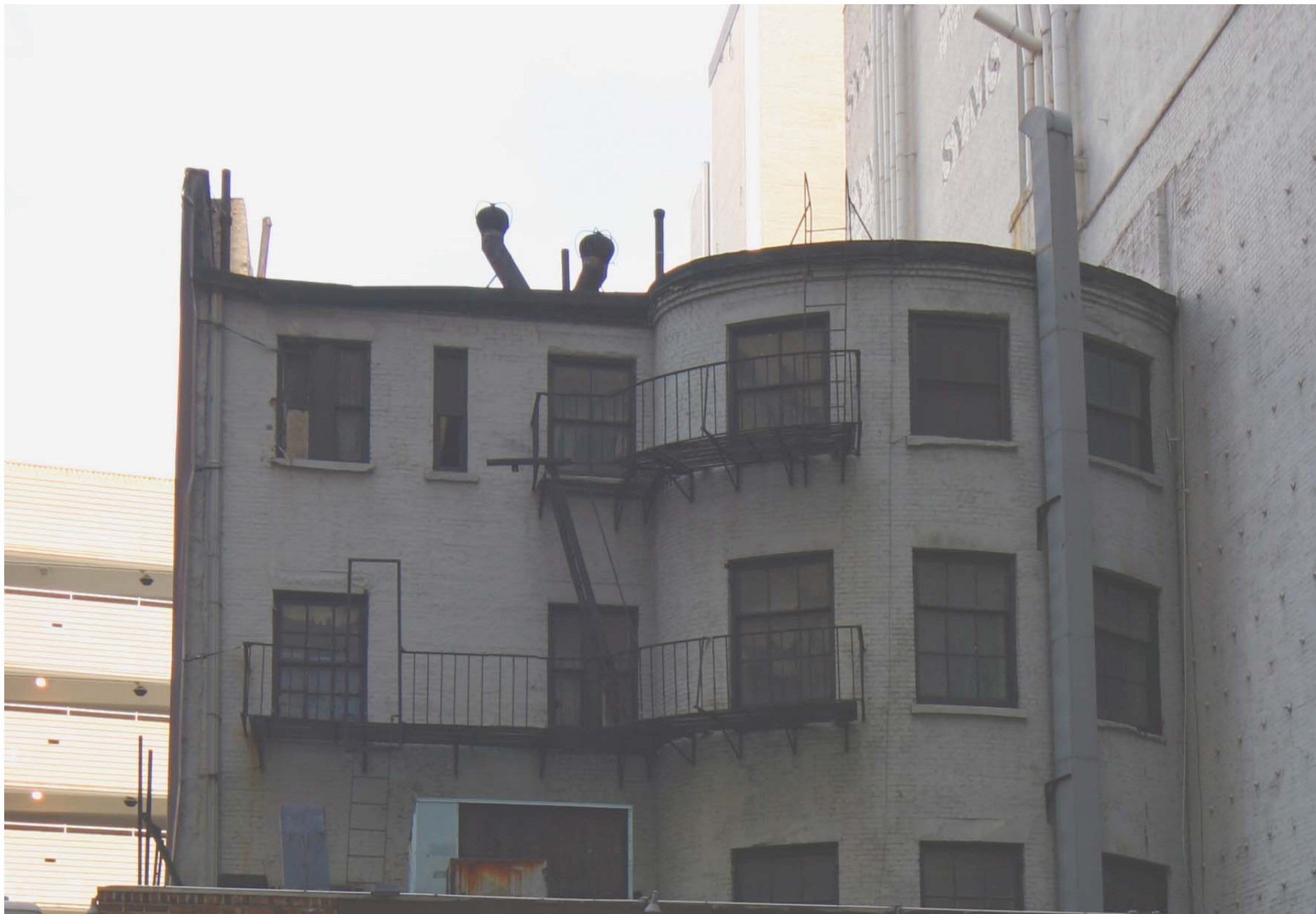
Robert and Anne Dickey House, rear façade upper stories Photo: Jenny Staley, LPC
