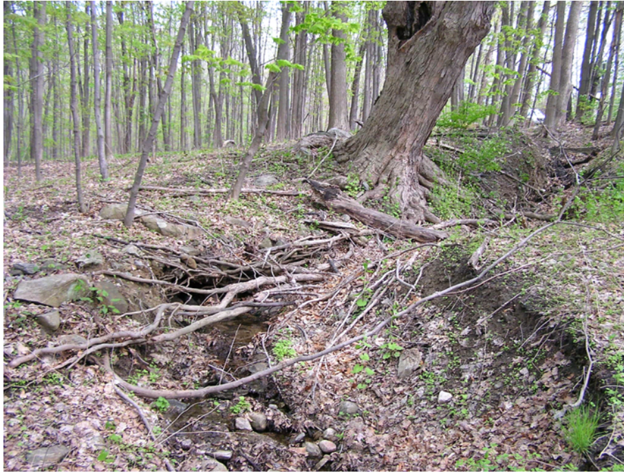
Figure 4.22. Eroded drainage ditch at Hemlock Road.
