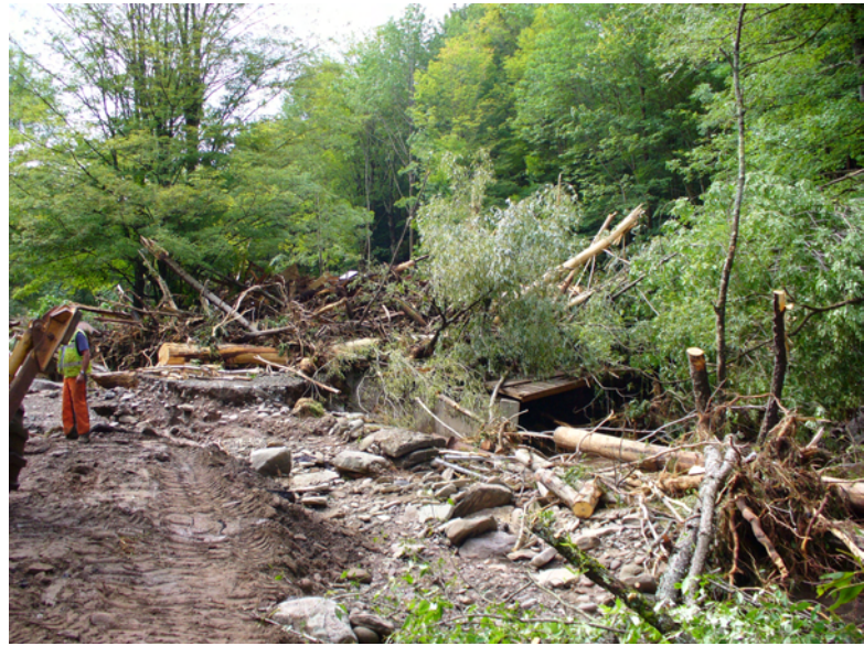
Figure 4.8. Woody debris, house remnants, and sediment jam a private bridge on DEP property along lower Holliday Brook.
