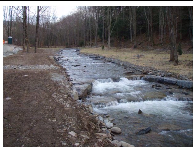
Figure 4.11. Completed cross-vane structure and adjacent grading on Holliday Brook. Roadway is visible at left.
