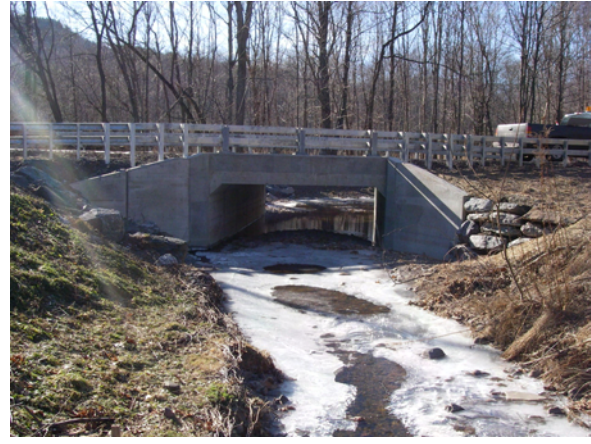
Figure 4.15. County Rte. 13 culvert after replacement. The culvert was upgraded to a 14' x 5' opening with the invert buried 1' and a low flow dish added for fish passage. Two floodplain drains were also installed in the field to the right.
