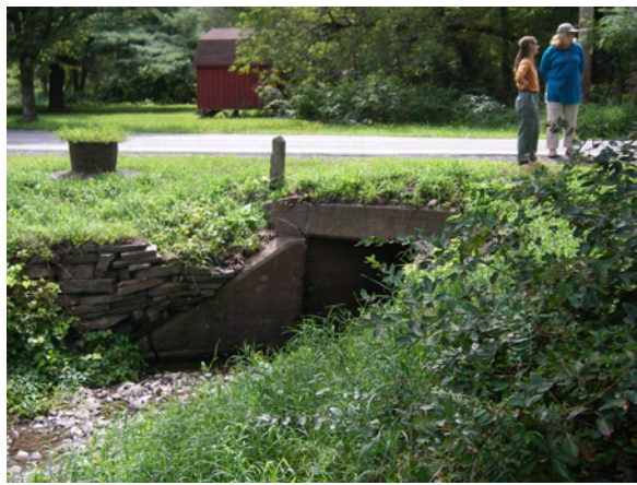
Figure 4.14. County Rte. 13 culvert prior to replacement. The left wing wall was collapsing and the culvert was undersized.
