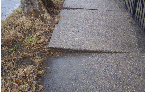
Left: Example of uneven surfaces along a sidewalk. Right: Sidewalk improvements remove obstacles for people with disabilities.
