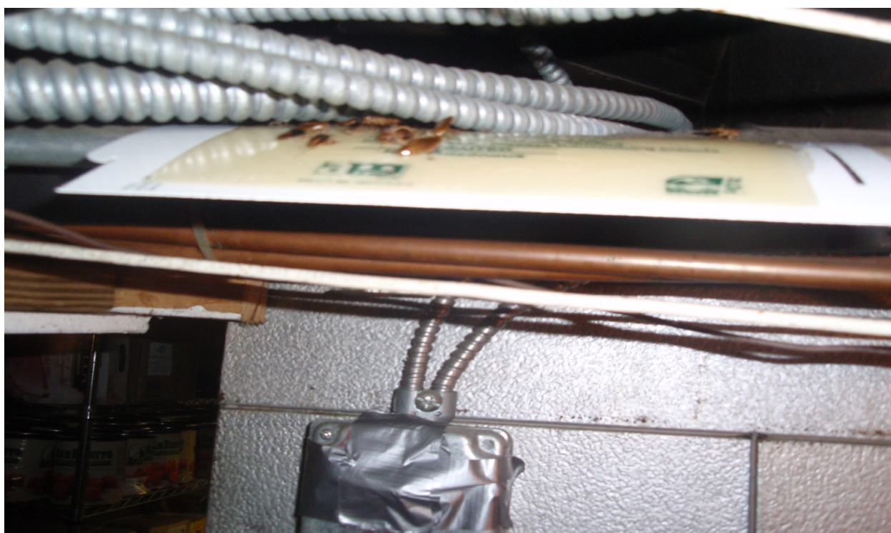
Glue trap with roaches found on top of some pipes near the basement ceiling.
