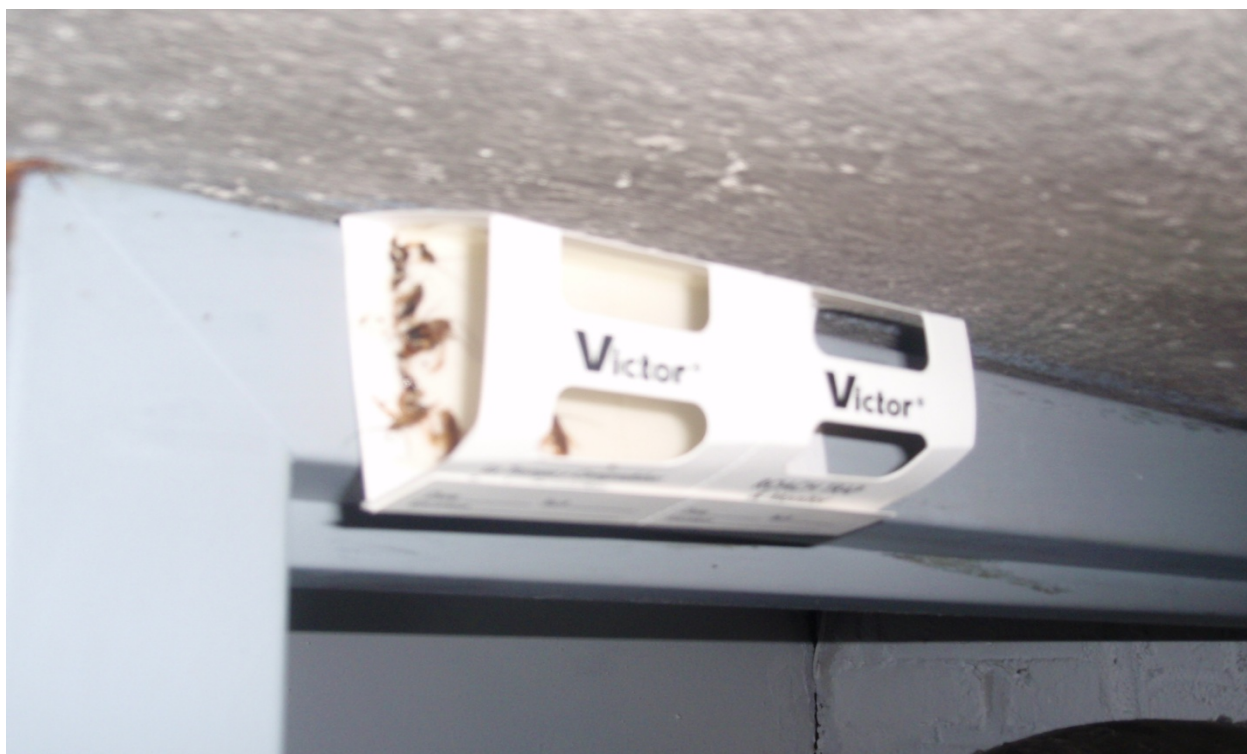
Glue trap with roaches placed on top of the entrance of the furnace room in the basement.
