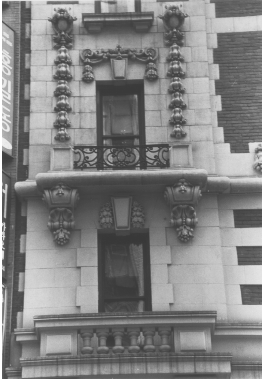
(Former) Aberdeen Hotel (now Best Western Manhattan Hotel), upper facade detail 17-21 West 32 nd Street, Manhattan
