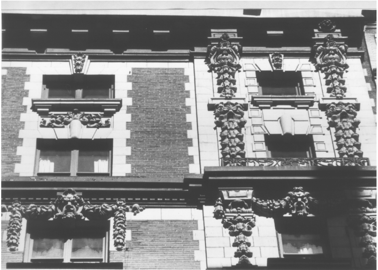
(Former) Aberdeen Hotel (now Best Western Manhattan Hotel), upper facade detail 17-21 West 32 nd Street, Manhattan
