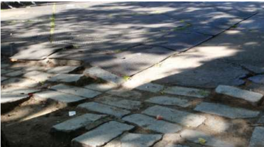
6. Dry Dock Playground Uplifted cobblestones and mats
