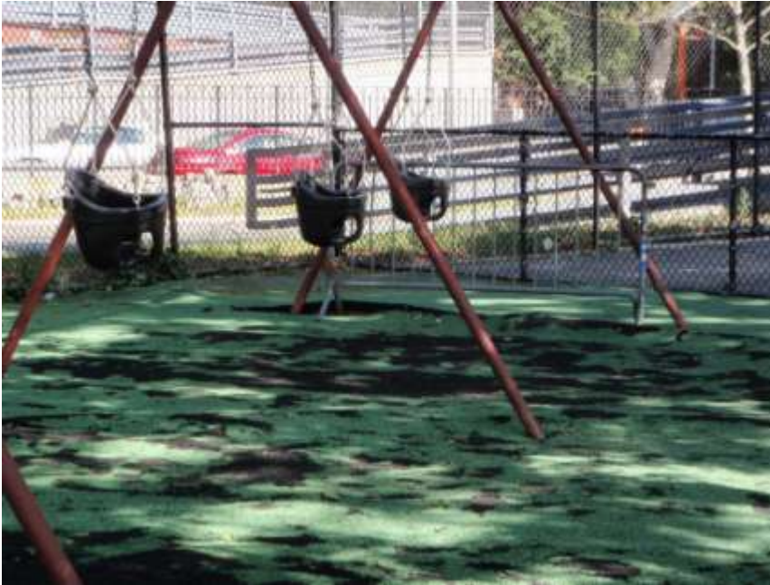
5. East River Playground Deteriorated safety surface at the swing area
