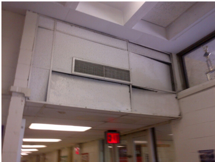
CORE photo of service center documenting loose wall covering
