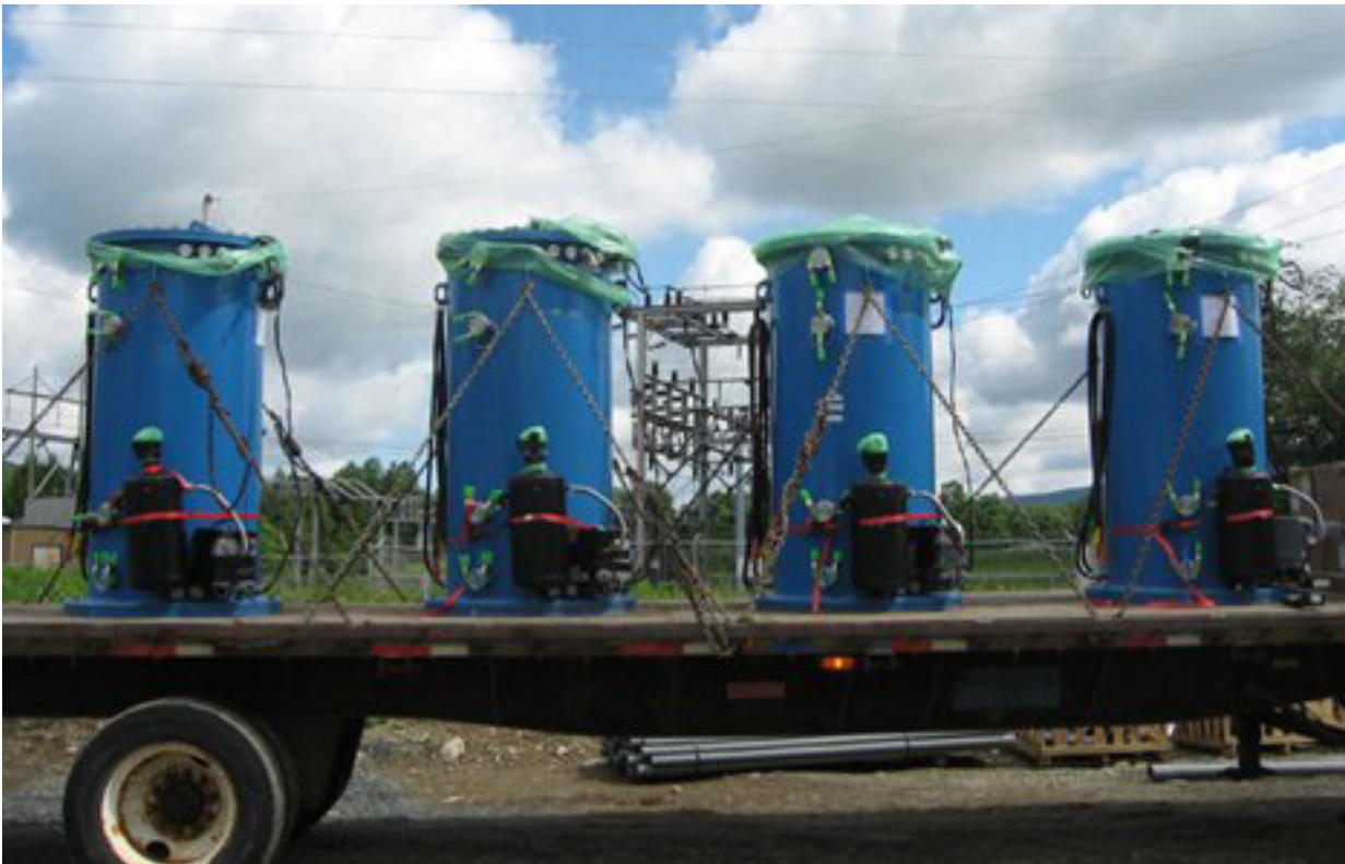
Figure 5: Flywheel Energy Storage Technology 11
