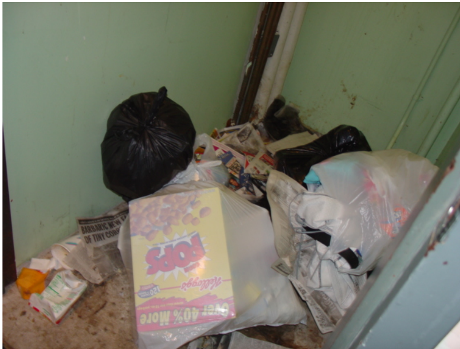
7 th Floor Hallway Trash in Front of Garbage Chute
