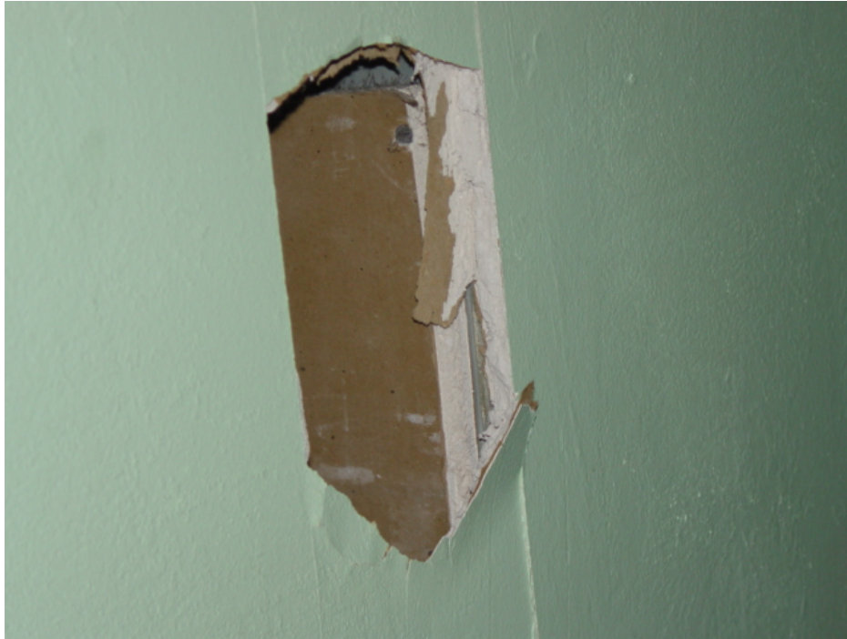
7 th Floor Hallway Hole in Wall
