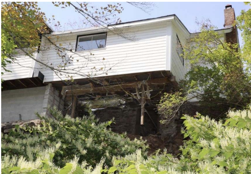
Figure 7: Residential structure in the Town of Jewett hanging over a failed stream slope.
