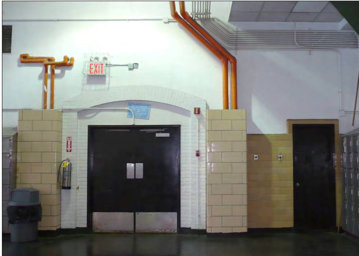
Crotona Play Center: Women's Locker Room Interior, West Wall Door Openings, Photo: Jennifer Most, 2007 Borough of the Bronx
