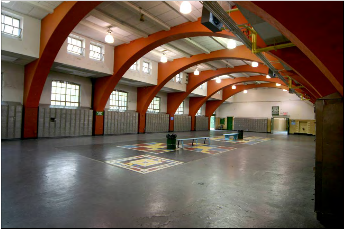
Crotona Play Center: Men's Locker Room Interior, North Wall (view northeast), Borough of the Bronx
