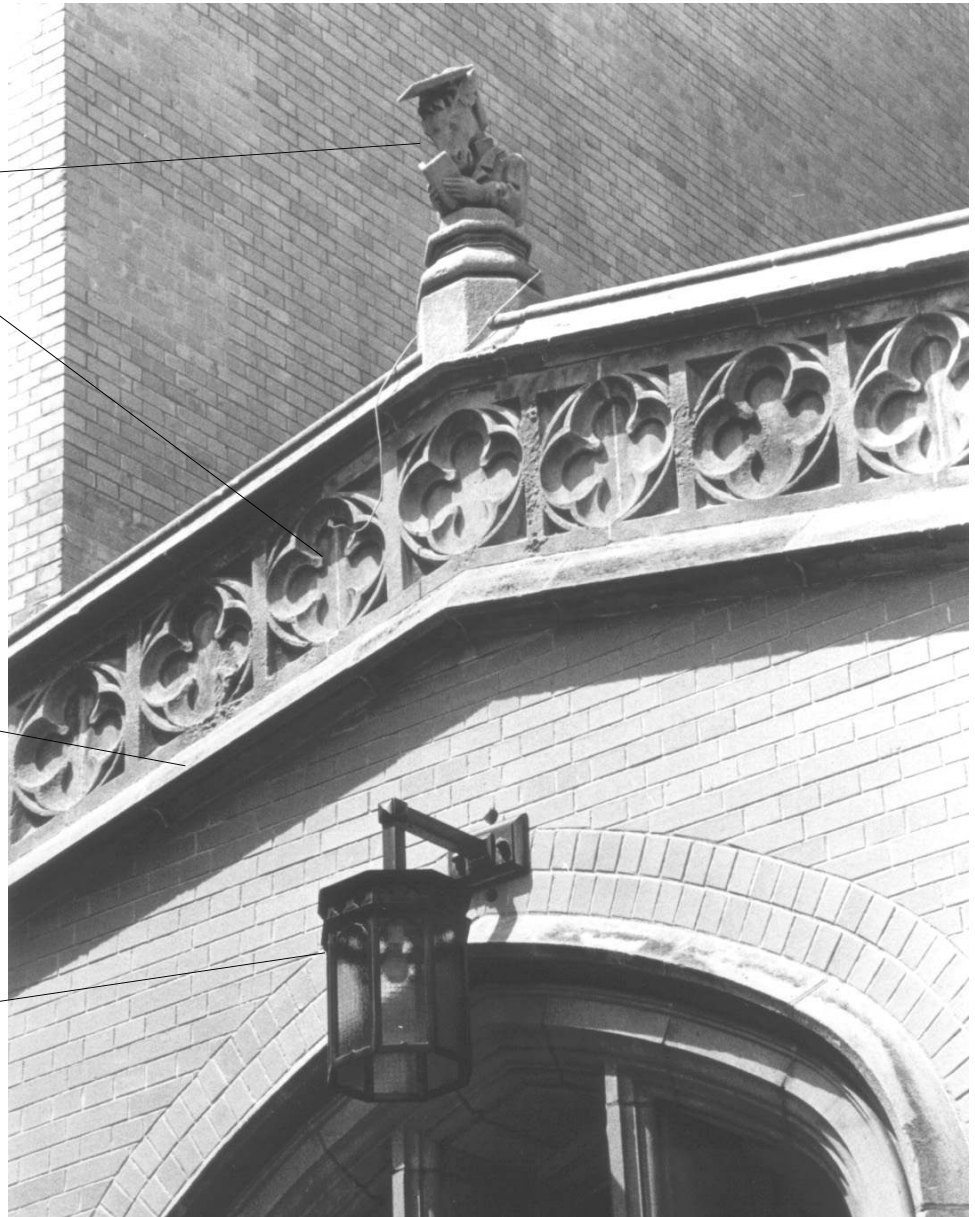
Erasmus Hall High School Entrance between buildings C and D Detail of finial, molding and doorway
