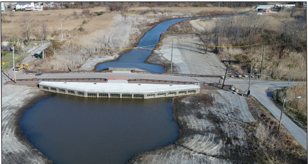
Figure 7 - A DEP bluebelt under construction in Staten Island designed to alleviate chronic flooding. Photo courtesy of JRCRUZ Corp.
