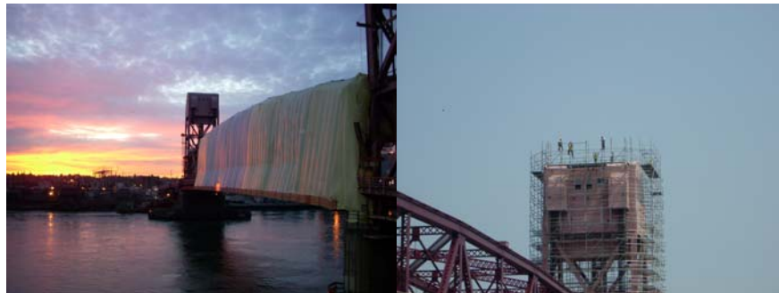
Lead Paint Removal Containment on the Roosevelt Island Bridge Lift Span in January 2008. Scaffolding Erection on the East Tower in July 2008.
