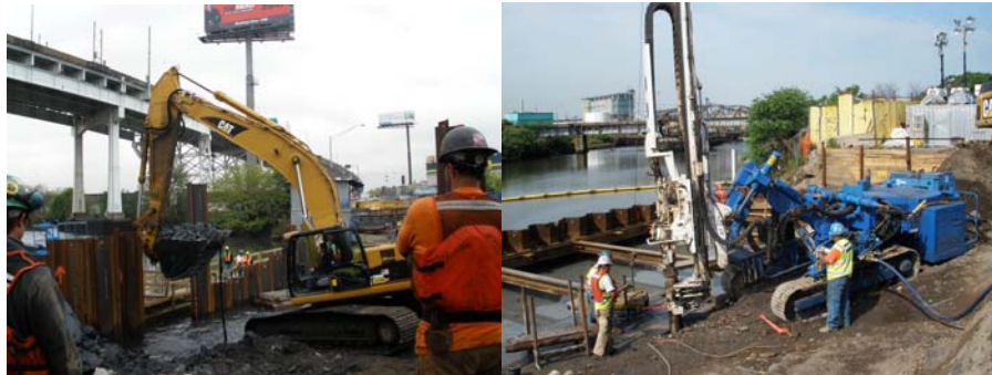
Removal of Obstructions for the Sheeting Operation in May 2009. Deep Well Installation Southwest of the Bridge in June 2009.
