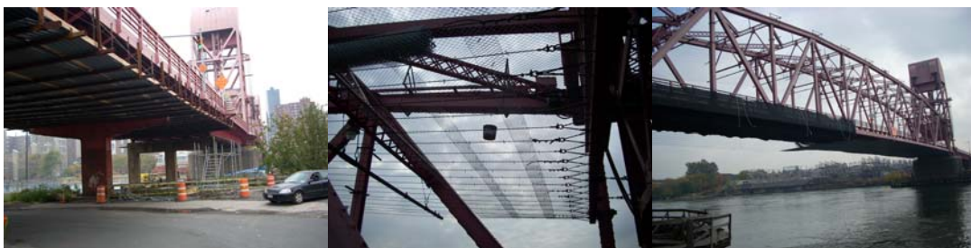
2007: Construction of the Below Deck Shield for the Queens Approach of the Roosevelt Island Bridge. Above Deck Containment on the Lift Span. The Lift Span Shield Looking Northeast.
