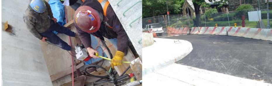
West 252 nd Street Bridge: Transverse Post-Tensioning of the Pre-Cast Concrete Beams in March 2007. Installed Asphalt on Bridge Approach in July 2007.
