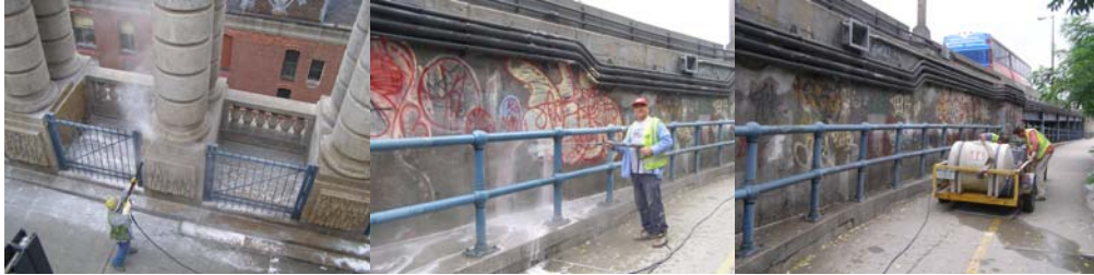
Removing Graffiti From the Manhattan Bridge in September 2009: William Budge at the Railing. (Credit: Earlene Powell)
