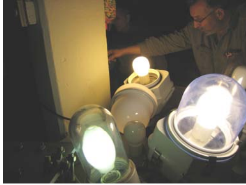
Supervisor Electrician Ben Cipriano in October 2008 With Both Mild and Bright Induction Light Fixtures for Testing. For Comparison Purposes, There is a Mix of Clear and Frosted Globes. (Credit: Russell Holcomb)
