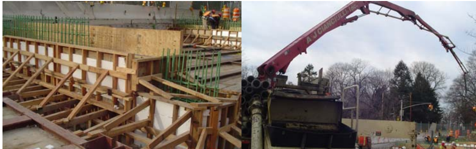
2007: West 252 nd Street Bridge Formwork and Rebar Fabrication at the Pier and West Abutment. Concrete Placement in Progress.
