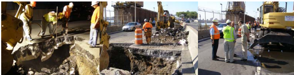
First Emergency Repairs at the FDR Drive in August 2009. Executive Director of Inspections and Bridge Management Dr. Bojidar Yanev (at Right) Visiting the Site.
