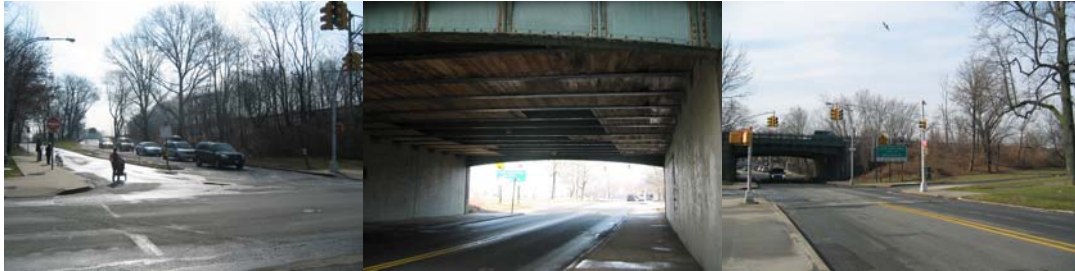
Cross Island Bridge Exit Ramp on the Northeast Side. Bridge Underdeck. South View of the Bridge. (Credit: Tamara Berlyavsky)
