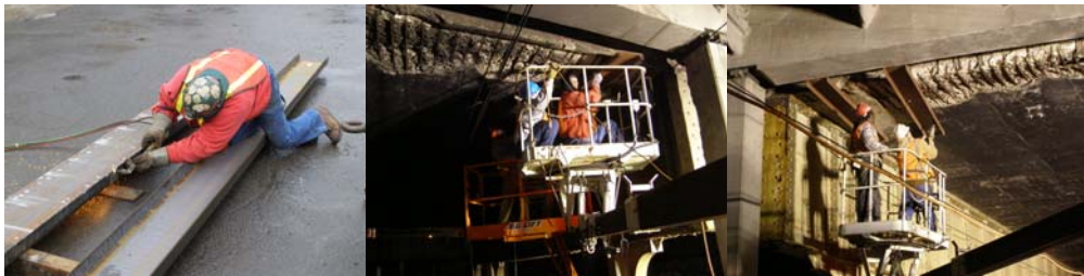
Removing Loose Concrete at the West 39 th Street Bridge over Amtrak 30 th Street Branch in March 2009.
