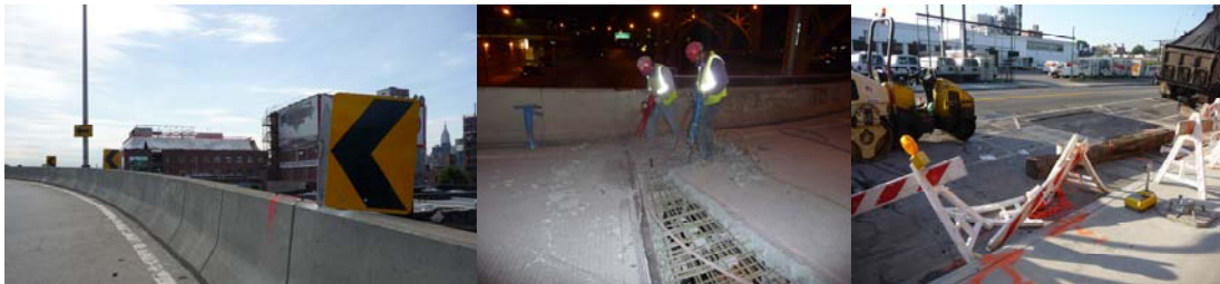
Performing Component Rehabilitation of Ramp G of the Queensboro Bridge in June 2009.
