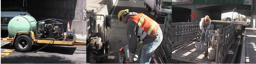
Pressure Washing Machine Used for Graffiti Removal. It is Set to 2500 psi and 212° F. Bridge Painters Frank Duic and Russell Newme Feeding the Spray Pump and Preparing the Paint.
