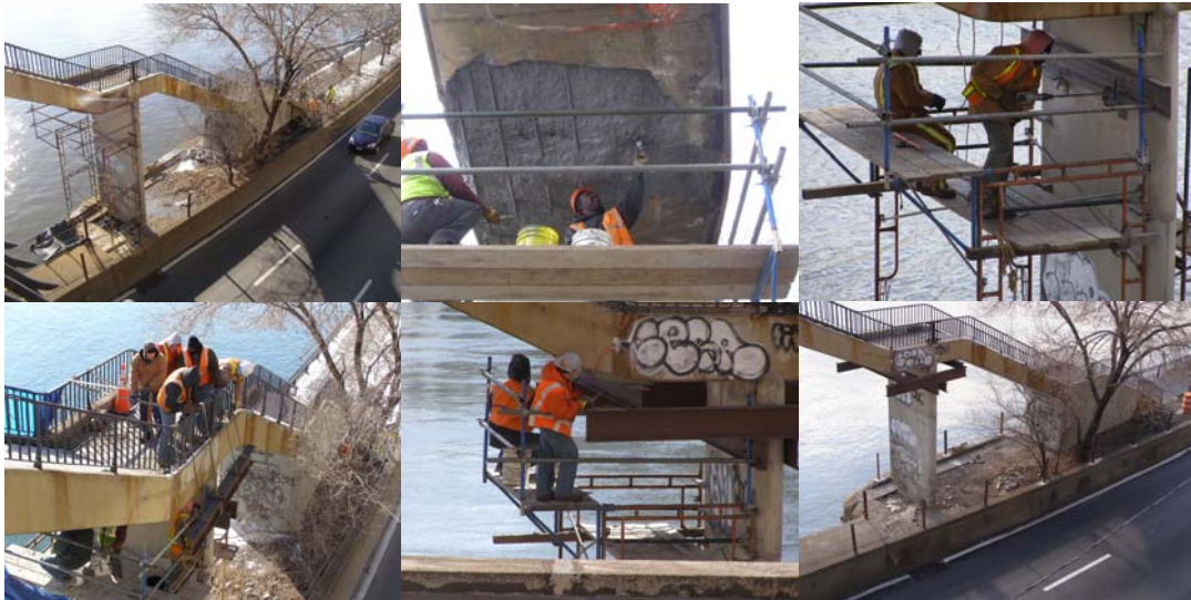
Installing Steel Shoring at the 81 st Street Pedestrian Bridge over FDR Drive in January and February 2009.
