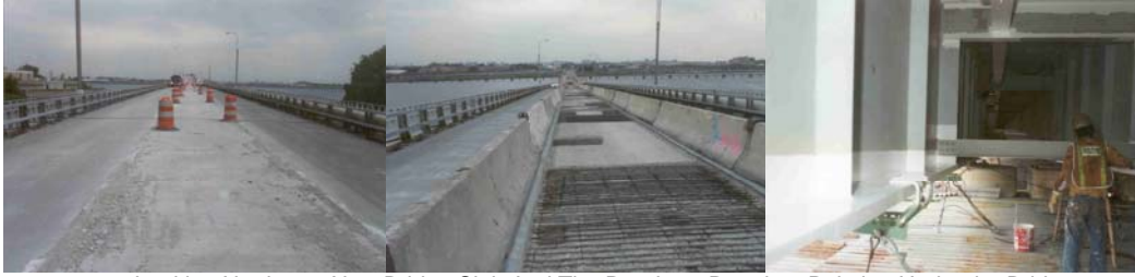
2006: Looking North at a New Bridge Slab And The Roadway Repairs. Painting Under the Bridge.
