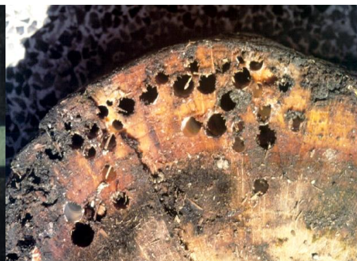
Teredo Damage (holes up to 1/4" diameter)
