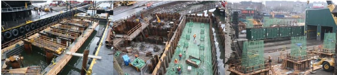
April 2009: Willis Avenue Bridge Pier 5 Precast Footing, Pier 8 Footing, and Pier 9 Rebar Columns.
