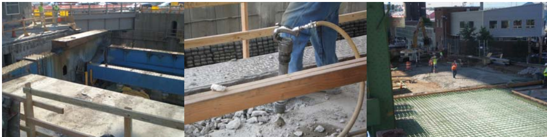
Removing the Existing Hamilton Avenue West Bridge Structural Steel in June 2008. Removing the Existing Southwest Toe Joint and Installing New Reinforcement of the Southwest Approach Slab in July 2008.
