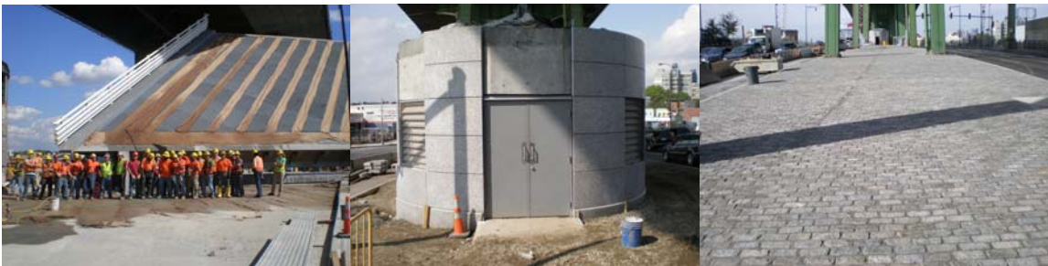
Completion of the New Hamilton Avenue West Bridge Installation in August 2008. Construction of the New Back Up Generator Building in September 2008. New Granite Pavers at the South Median Area in October 2008.
