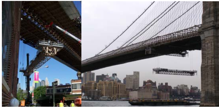
Lifting Traveler #4 in June 2008. Lifting the New Manhattan Main Span Traveler to the Underside of the Bridge on November. 20, 2008. (Main Span Credit: Bojidar Yanev)
