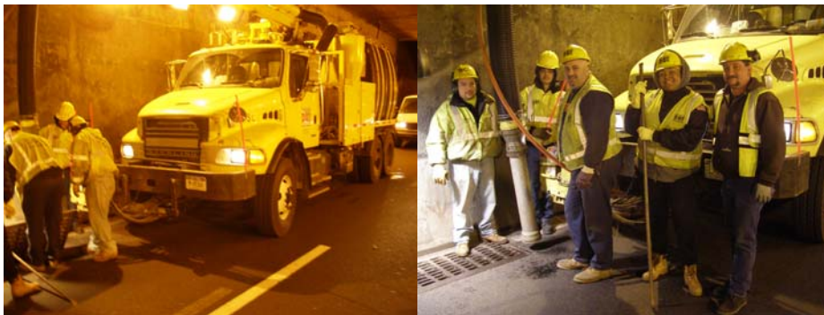
Cleaning a Drain: Supervisor Highway Repairer Michael Parise, Highway Repairer Anthony Irizarry, and Assistant City Highway Repairer Danny Alvarado. Darin Crew: Assistant City Highway Repairer Danny Alvarado, Highway Repairer Anthony Irizarry, Supervisor Highway Repairer Michael Parise, Assistant City Highway Repairer Claudia Wilkinson, and Highway Repairer Michael Cunningham. (Credit: James Campbell)
