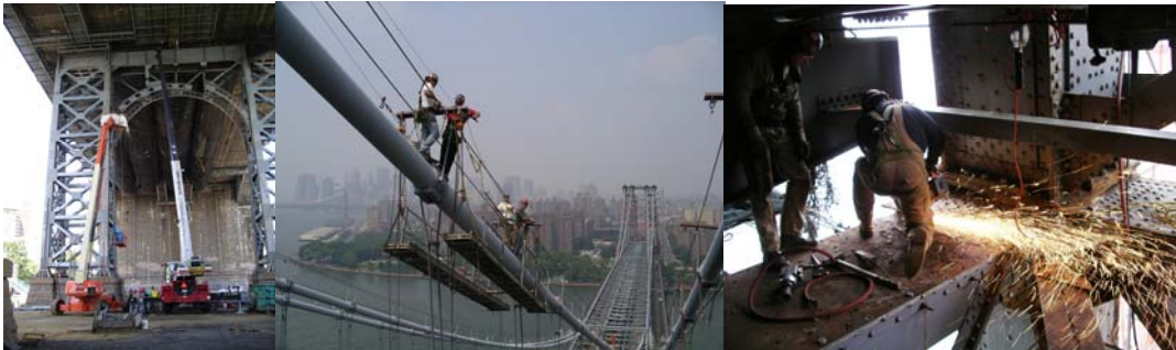
2004: Steel Arch Replacement. Cable Band Bolt Retensioning. 2005: Rehabilitation of the Brooklyn Main Tower Steel.
