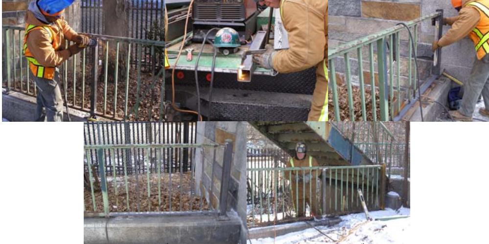
Fixing the Railing at the West 148 th Street Pedestrian Bridge over Amtrak 30 th Street Branch in January 2009.
