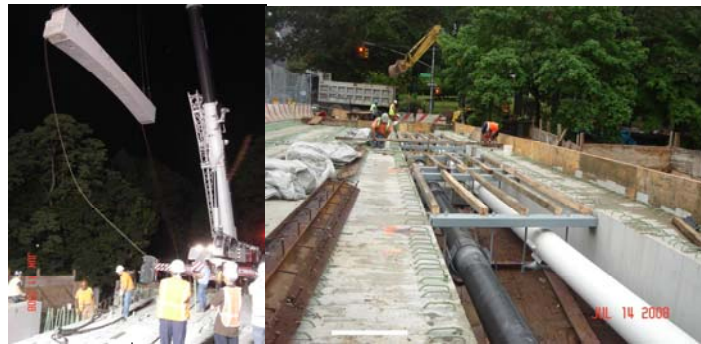
West 252 nd Street Bridge: Placing New Precast Prestressed Concrete Box Beam on the Bridge Deck in June 2008. Installation of Water and Gas Mains in July 2008.
