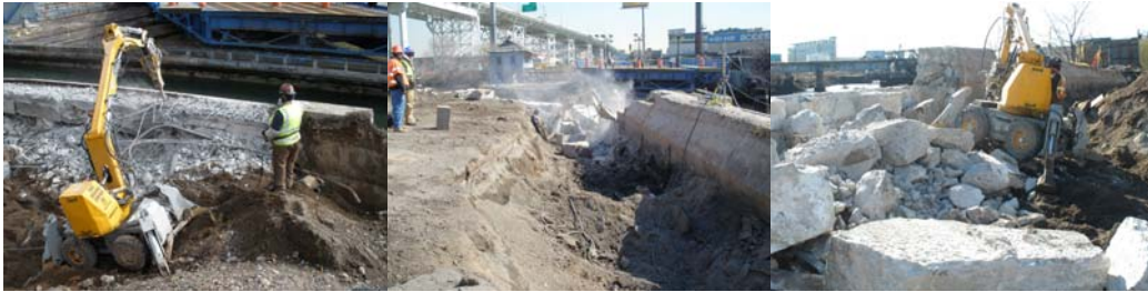
Demolition of the West Abutment and Wingwall in February 2009. (Third View Credit: Reza Lotfi)
