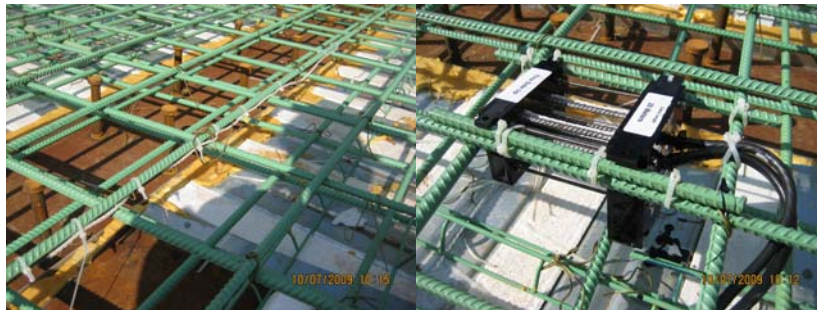
The Corrosion Monitoring Probe Sensor Measures the Electrical Potential Between the Rebar and the Electrode. The Corrosion Penetration Monitoring Probe Sensor Measures Corrosion Caused by Chlorine Containing Moisture.
