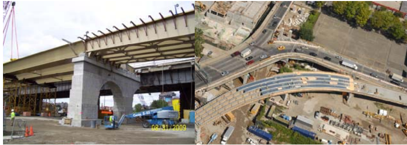
Willis Avenue Bridge August 2009: Installation of Tub Girders on Temporary Supports. September 2009: Existing and New Ramps to Bruckner Boulevard.
