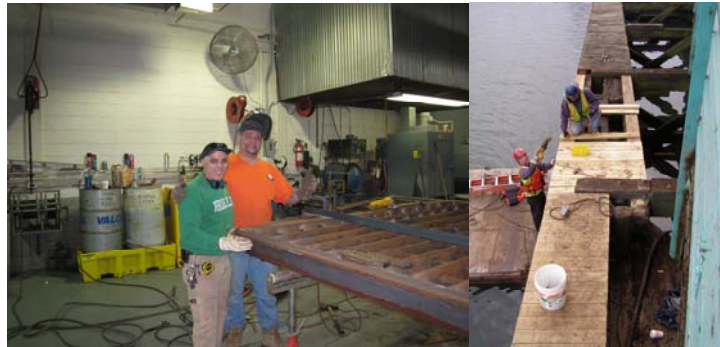
Bridge Repairer and Riveters Ignazio Trapani and Christopher Sabbagh Fabricating a New Grizzly for the Agency Asphalt Plant. (Credit: Russell Holcomb) Bridge Repairer and Riveters Michael Greenwood and Damian Venezia Replacing Deteriorated Planks on the Grand Street Bridge in October 2009.
