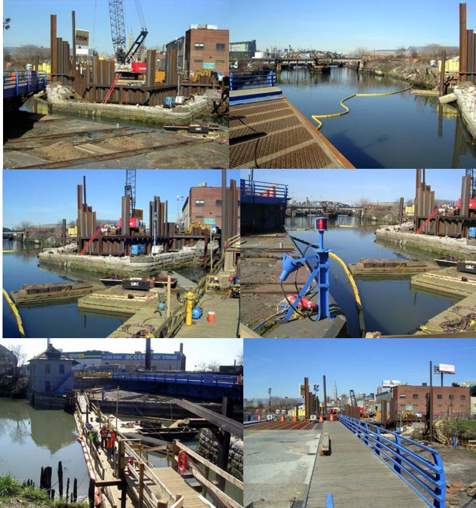
Reconstruction of West Abutment of the Borden Avenue Bridge in April 2009. (Credit: Bernard Ente)
