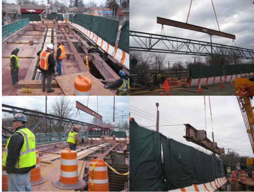
Annadale Road Bridge: Stage I Construction in February 2009. Saw Cutting the Diaphragms, Removing the Stringers, And Placing a Temporary Truss to Support Utility Conduits.
