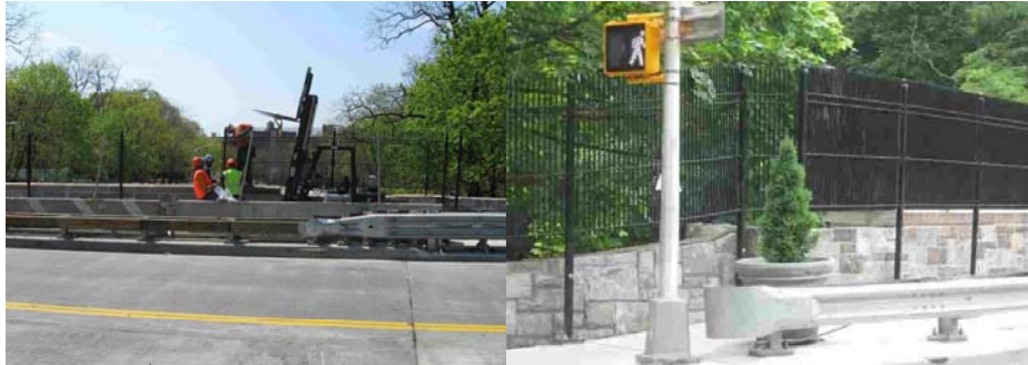
West 252 nd Street Bridge: Installing the Protective Steel Picket Fence. View of the Sidewalk After Reconstruction.
