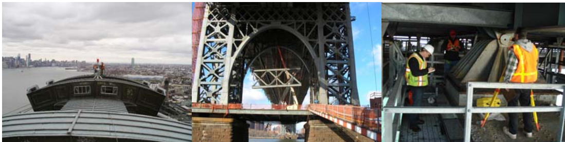
2005: Installing Brooklyn Main Tower Aviation Lights. 2006: Truss A Removal, Brooklyn Tower. Bearing Survey.
