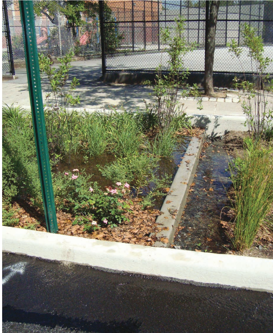
Check dams can separate different levels of a planting area to allow for greater control of slopes and to increase detention: Westbourne Avenue at Bay 25th Street, Queens (Credit: DPR)
