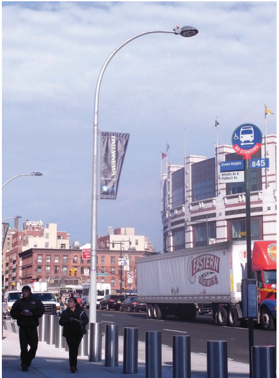
Helm luminaire on Davit pole: Flatbush Avenue, Brooklyn
