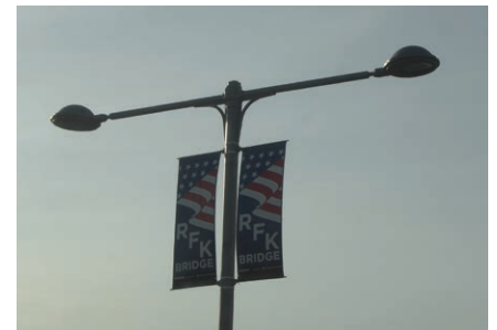
Stad luminaires on TBTA pole: Robert F. Kennedy Bridge, Manhattan
