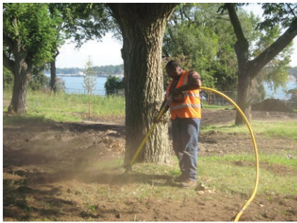
RIGHT: Removing soil from around a tree's roots through pneumatic excavation allows for work to be done without damaging the tree: LEFT - Fort Totten Park, Queens (Credit: DPR); RIGHT - 235th Street and 119th Avenue, Queens (Credit: Lisa Montana)
