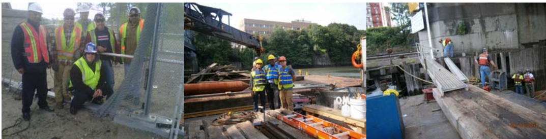
Bridge Maintenance Personnel Building a New Prototype Pedestrian Fence in April 2012. Standing: Director of Bridge Repair Pinakin Patel, Bridge Repairer and Riveter Charlie Zhao, Acting Director of Bridge Preventive Maintenance Paul Schwartz, and Bridge Repairer and Riveters Ignazio Trapani and James Philip. Foreground: Executive Director of Bridge Preventive Maintenance and Repair Thomas Whitehouse. Broadway Bridge Fender System Rehabilitation Work in August 2012: Administrative Engineer Sunil Desai, Assistant Civil Engineer Li Yi, and Civil Engineer Antoine Aubourg.
