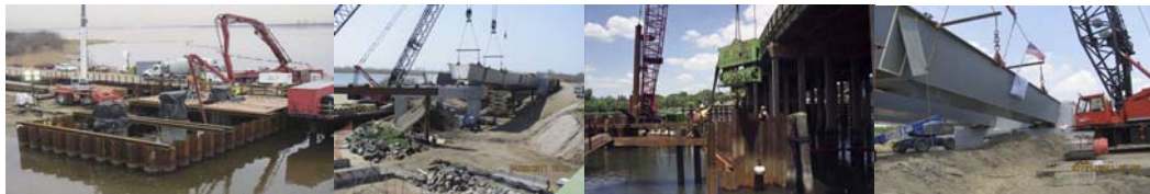
February 2011: Pumping Concrete at Paerdegat Basin Cofferdam for Pier No.3. April 2011: Setting Tub Girder Sections at Eastbound Bridge Between West Abutment and Pier No. 1. June 2011: Hammer Being Positioned to Drive Steel Sheet Piling for Cofferdam at Westbound Bridge – Pier # 2. July 2011: Setting Final Tub Girder Section at East Abutment.
