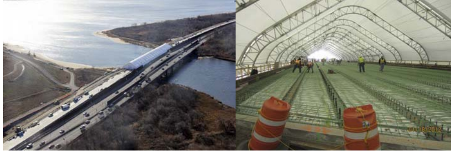
Fresh Creek Bridge: Winter Tent Enclosure for Stage IIB Concrete Bridge Deck Placement.
