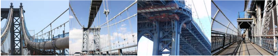
September 2012: Main Cable Work Platforms. New Suspenders Along Truss B. September 2012: Jacking Struts and Work Platforms. November 2012: Sidewalk Protection Sheds.
