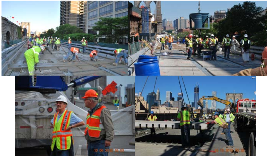
First Full Roadway Closure in October 2012: Manhattan Approach, Ramp A Concrete Placement. Chief Bridge Officer Henry D. Perahia and Deputy Chief Engineer Robert Collyer at the Site. Second Full Roadway Closure: Brooklyn Approach, Brooklyn Bound Roadway Super Slab installation - Installing Super Slab.
