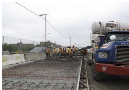
Placing and Finishing On-Grade Concrete Pavement for Westbound Roadway on West Side of the Rockaway Parkway Bridge.
