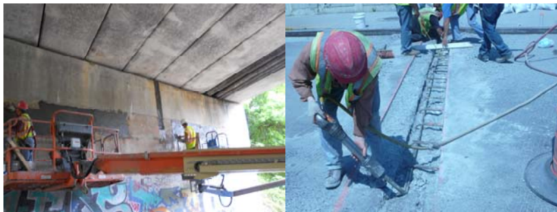
15 th Avenue Bridge - Vertical Patch Repair on the Abutment Wall. Joint Repair Work.
