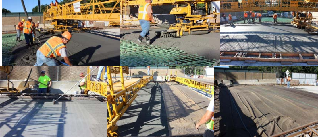
Following Behind the Finishing Machine Along the Deck, the Concrete was Textured and Wet-Burlaped Within the Prescribed Time Limits. Texturing was Performed in the Longitudinal Direction. Continuous Wet Curing was Set up With Hoses Over the Burlap.
