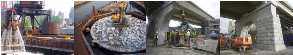
June 2011 River Work: Picking Up Waste With a Clamshell Bucket. July 2011: Demolition of Old Pier 9. March 2011: Stage III Caisson Concrete Placement at Caisson #2 at Pier 11. Setting Granite Stone Facing at Pier 11. Finished Stage VB Removal of Steel Girder at South Bay at Existing Span 15.
