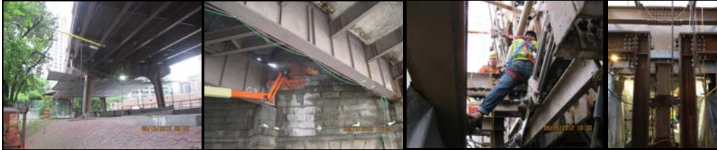
June 2012: Platform Removal at Ramp D. Granite Removal at Main Street Structure. Structural Steel and Flag Repairs.
