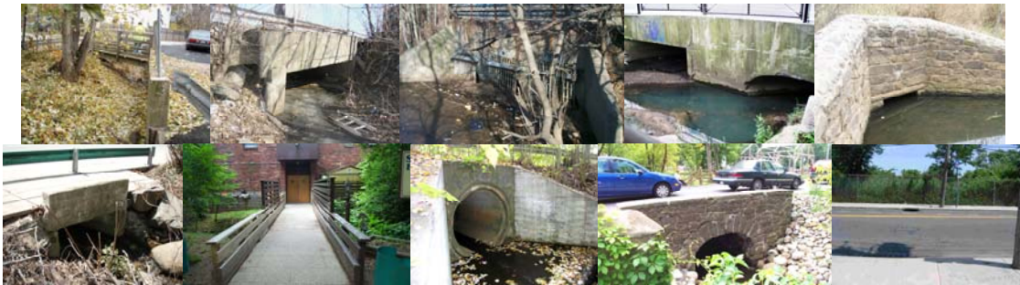
Galloway Avenue over Marianne Street, Forest Avenue over Crystal Avenue. Naughton Avenue over Patterson Avenue, Midland Avenue over Hylan Boulevard. Rockland Avenue over Brielle Avenue, Forest Avenue over Randall Avenue. Gregg Place over Randall Avenue, Arthur Kill Road over Muldoon Avenue. Richmond Hill Road over Richmond Road, Arthur Kill Road over Ridgewood Avenue.
