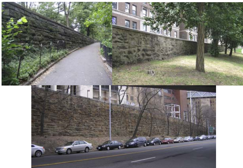
Riverside Drive Retaining Walls: Riverside Drive Between West 99 th Street and 104 th Street, and Riverside Drive Between West 158 th Street and West 165 th Street. Riverside Drive Retaining Walls: Left Side of Riverside Drive Northbound, Holds Ramp to George Washington Bridge.
