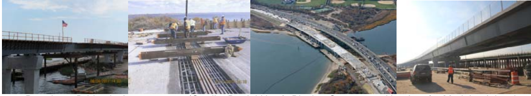
Paerdegat Bridge in August 2011. (Credit: Daniel Hom) Placing Concrete at Headers for Modular Joints in November 2011. November Aerial View. December 2011: New Eastbound Bridge.
