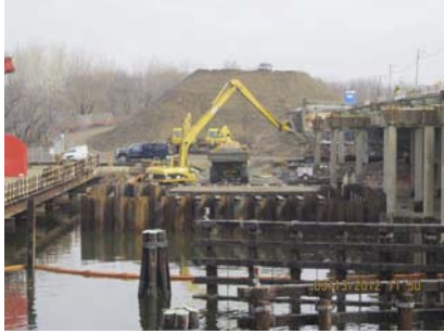
Paerdegat Basin Waterway with Partially Demolished Bridge, Temporary Work Platform, and Pier 2 Cofferdam. Embankment for Future Westbound Bridge in Background.
