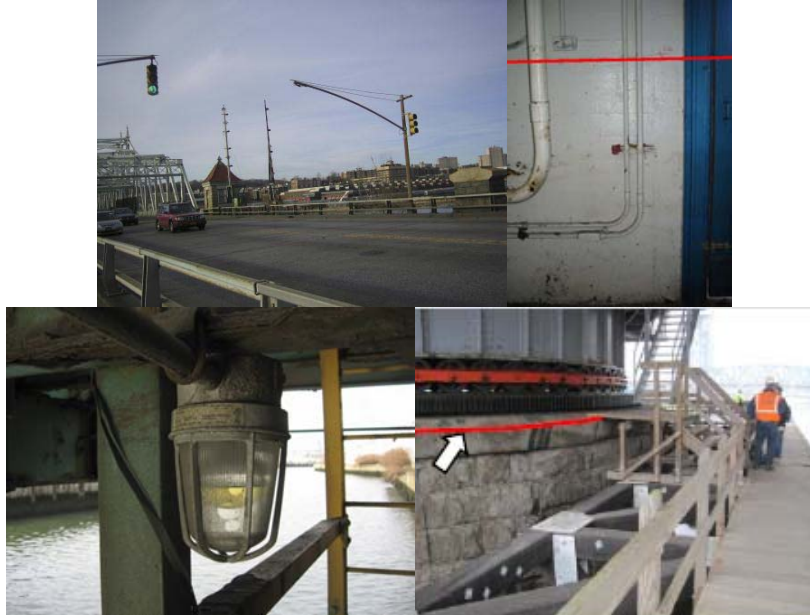
East End of the West 207 th Street Bridge - Missing Traffic Signal was Knocked Down by the Hurricane Winds. Borden Avenue Bridge Operator's House Basement Level – Depicted Flood Line was Approximately 5 Feet Above the Floor. Grand Street Bridge – Standing Water in the Access Light Fixture at the East Wedge Walkway. Madison Avenue Bridge - General View of Fender and Center Pier—the Red Line Depicts the Approximate Water Level.
