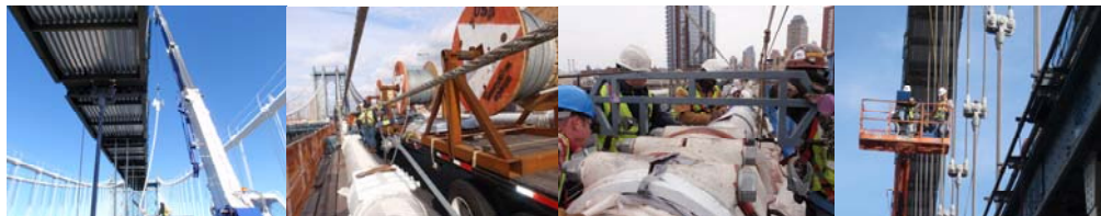
March 2011: Removal of Existing Suspender, 'C' Truss. April 2011: Installation of New Hand Ropes for 'C' Cable. April 2011: Checking Bolt Tension in New Cable Band Bolts. August 2011: Checking Suspender Loads With an Accelerometer.
