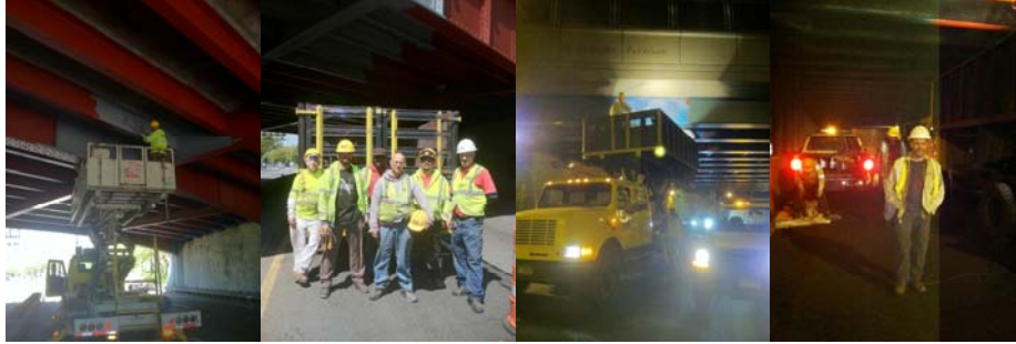
April 2012: Bridge Painter Juscelino Andrade at Knapp Street Bridge over Belt Parkway. Bridge Painters Andrew Law, Juscelino Andrade, Henry Bollin, Julio Perez, and Samuel Martinez, and Supervisor Bridge Painter David Yanolatos. Woodside Avenue Bridge over Brooklyn-Queens Expressway. Supervisor Bridge Painter Hughie Flood at the 69 th Street Bridge over Brooklyn-Queens Expressway. (Credit: Earlene Powell)
