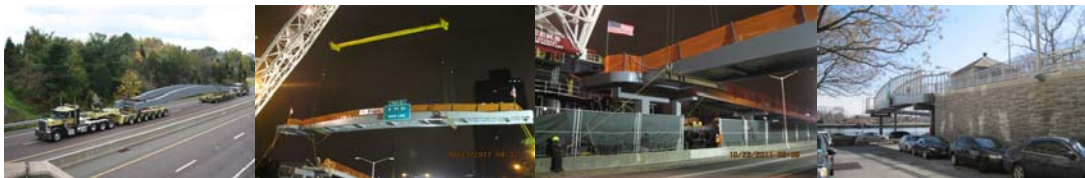
The New Bridge Span in Transit from Just North of Philadelphia to Jersey City. It was Then Loaded on the Barge and Brought up the East River to the Site. The Span Size was 26' x 135' and Weighed Approximately 80 Tons. New Main Span Steel Erection in October 2011. New West Ramp Masonry Wall.
