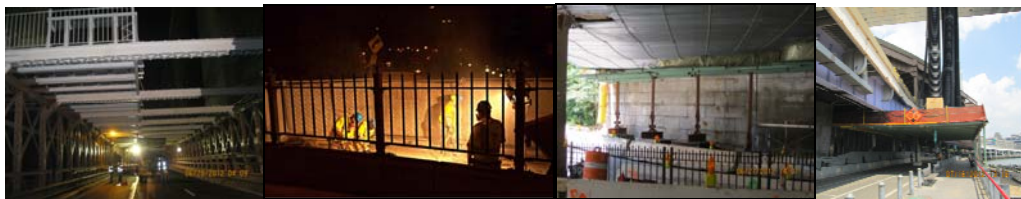
June 2012: Night Shift - Brooklyn Bound Brooklyn Tower Top Struts Primer-Intermediate Coat in Progress. Super Slab Installation on the Brooklyn Approach Brooklyn-Bound Lanes. Temporary Supports at the Park Row West Abutment. Duct Hose Platform Over Esplanade.
