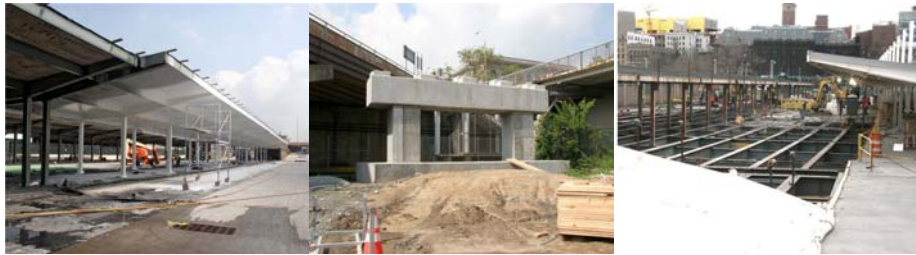
August 2011: Bus Ramp A Canopy. North Ramp Center Pier. December 2011: Bus Ramp D.
