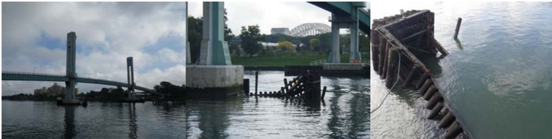
Emergency Inspection on Wards Island Bridge Revealed that the Southwest Fender System Collapsed and Required Repairs.
