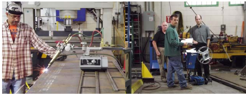
In September 2012, Bridge Maintenance Personnel Fabricated a Mock-Up Overheight Protection Beam for the Westchester Avenue Bridge over Hutchinson River Parkway. This Enabled the In-House Design Engineers to Prepare the Final Shop Drawings. Bridge Repairer and Riveter James Philip Using a Track-Mounted Torch to Bevel the Edge of the Steel Plate. Electrician Patrick Fitzgerald, Supervisor Bridge Repairer and Riveter John Jones, and Acting Director of Bridge Preventive Maintenance Paul Schwartz Discussing the Next Step in Setting up the Sub-Arc Welder for Fabrication of the Beam.
