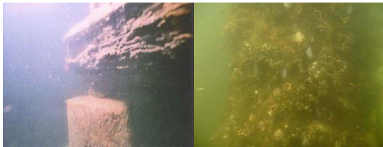
Severe Marine Borer Infestation in Timber Cribbing of Carroll Street Bridge and Moderate Marine Growth Below Waterline on the Ocean Avenue Pedestrian Bridge in 2009. (Credit: NYSDOT)
