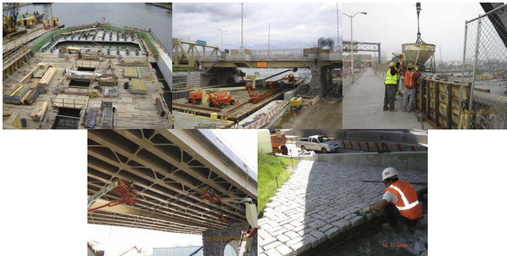
May 2012: Pier 6 North Fender. Touch-up Paint Operations at the Underside of Span 5. Finished Span 10 Parapet Wall Concrete Placement. Girder Touch-up Painting at Span 12. Preparing and Installing Granite Stone Pavers at Ramp-C End Abutment.
