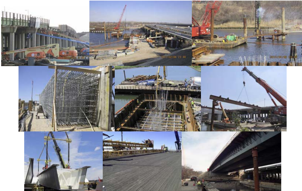
Paerdegat Basin Bridge in January 2012: Removal of Existing Westbound Lanes. February 2012: North Side Cofferdam and Pier for New Westbound Bridge. Driving Piles for Temporary Work Trestles on the North Side for the Future Westbound Bridge. April 2012: Galvanized Steel Rebars for Westbound Pier 1 Cap Beam. May 2012: Pumping Concrete for Footing of Westbound Bridge Pier 2 Cofferdam. Galvanized Rebars for Footing and Piers Shown. June 2012: Erecting Steel Falsework Temporary Supports for the Westbound Paerdegat Tub Girders. Unloading Tub Girder Section for Westbound Paerdegat Basin Bridge at Contractor's Storage Yard. October 2012: Finished Concrete Deck on Westbound Paerdegat Basin Bridge. Finishing Machine and Mason's Bridge at Left. November 2012.
