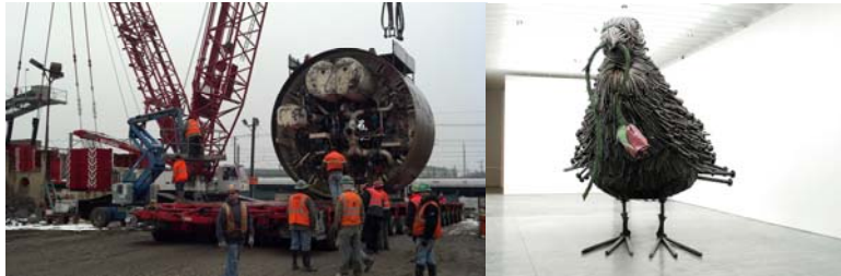
In January 2012, the Section Coordinated a Series of Supersized Moves with Bay Crane to Move a 435,000 Pound Tunnel Boring Machine Head and a Smaller Machine Head Weighing 150,000 Pounds, as Part of the Ongoing Eastern Access Project. The Vehicle was 27'-10" high, 22'-5" Wide, and 94'-2" Long, With a Gross Weight of 689,800 Pounds. In February 2012, the Section Issued a Permit for the Move of the Sculpture "Bird" by Will Ryman. The 12 Feet High, 16 feet Wide, 2 Ton Sculpture was Exhibited From February 16 Until March 24, 2012. (Credit: Will Ryman and Paul Kasmin Gallery)
