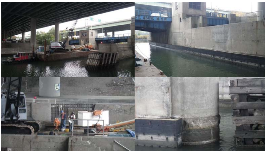
Unionport Bridge – Rebuilt the West Wall Fender System to Stop Barges From Hitting the Side of the Bridge. Safety Flags on the Concrete East Parapet Wall Were Also Completed. (Credit: Thomas Leung)
