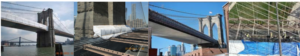
August 2012: Manhattan Side Span Containment at Manhattan Tower. Brooklyn Side Span Protective Shield. Brooklyn Side Span Suspender Ropes Painting.
