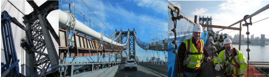
April and September 2012: Manhattan Bridge Suspender Replacement. (Credit: Bojidar Yanev) December 2012: Manhattan Bridge Engineer-in-Charge Brian Gill and Deputy Chief Engineer Russell Holcomb on the Bridge.
