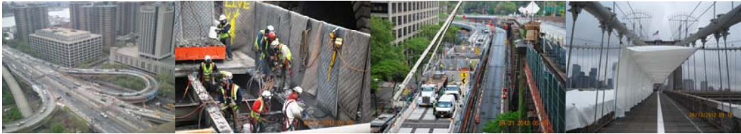
April 2012: Overview. (Credit: Maria Mikolajczyk) Manhattan Approach, Ramp A Existing Deck Demolition. June 2012: Brooklyn Side Span Netting Protection for Main Cable and Suspender Rope Painting.
