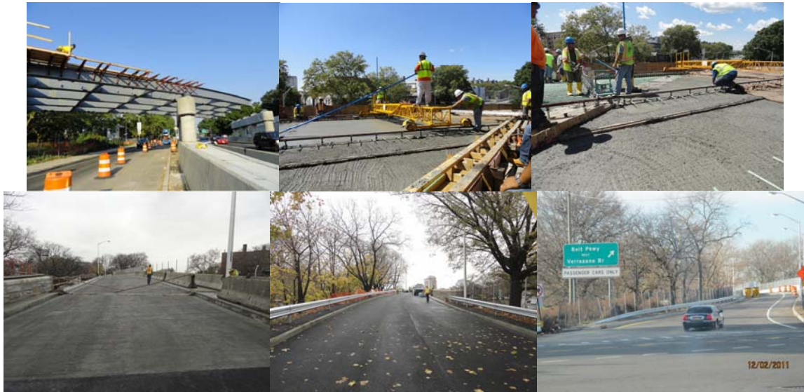
2011: Installation of Steel Girders over the South Service Road and Eastbound Belt Parkway. August 2011: Concrete Deck Placement. November 2011: Completed North and South Approach Roadways. December 2, 2011: Bridge Open to Traffic.
