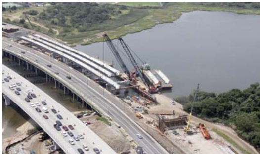
Paerdegat Basin- Eastbound Belt Parkway Traffic on New Eastbound Bridge Shown at Left. Westbound Belt Parkway Traffic on Old Paerdegat Basin Bridge at Center. Tub Girder Erection in Progress at Right Side by Crane on a Temporary Work Platform at Future Westbound Bridge.
