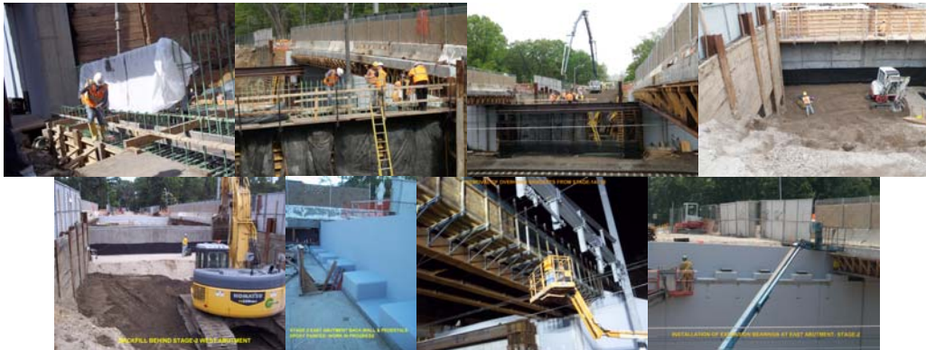
Shore Road Circle Bridge in April 2012: Placing Concrete for Stage 2 West Abutment Footing. May 2012: Stage 2 Backfill Behind East Abutment. East Abutment Backwall Rebar Installation. June 2012: Backfill Behind Stage 2 West Abutment. Painting of East Abutment Back Wall and Pedestals. June 2012: Removing Brackets from Stage 1A/1B. Installing Expansion Bearings at East Abutment in Stage 2.
