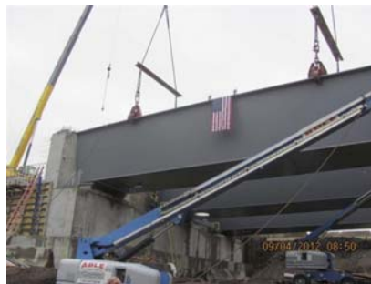
Setting the Last Tub Girder Section for the Westbound Bridge at the East Abutment.
