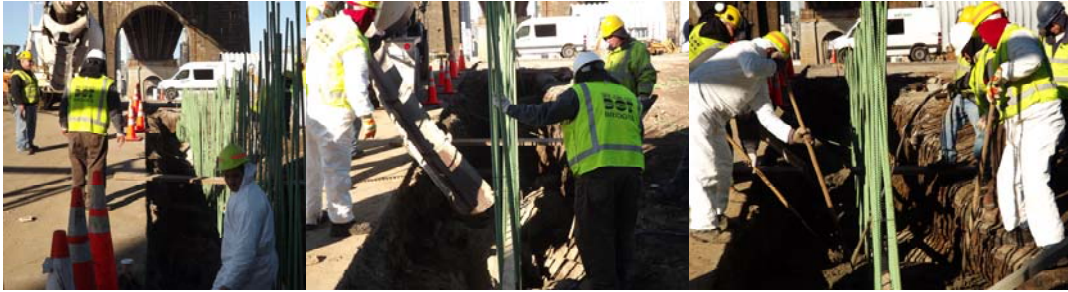
December 2012: Preparing a Footing for a Concrete Pad That Will Hold Office Trailers and Storage Containers in the Vernon Boulevard Yard Under the Ed Koch - Queensboro Bridge. (Credit: Thomas Whitehouse)
