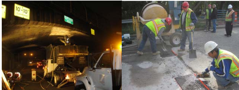
Sandblasting the Underdeck Concrete and Rebar on the Superior Road Bridge. Placing Rapid Hardening Polymer Concrete.
