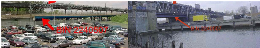
Roosevelt Avenue Bridge (#2240507) in 2002 and 2004. (Credit: NYSDOT)
