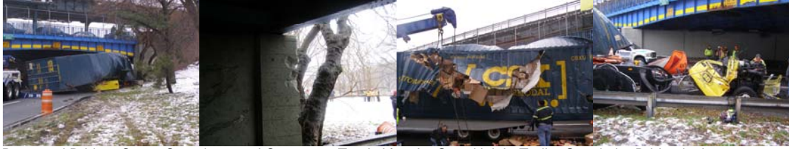
Damaged Bridge, Cargo Container, and Contractor Truck After An Over-Height Trailer Struck the Bridge in January 2012.
