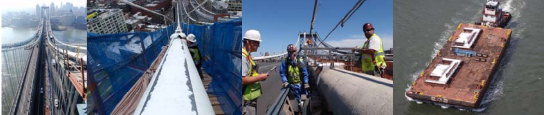
March 2012: View of Bridge From Tower Top. April 2012: Application of Anti-Skid Walking Surface on Main Cable. June 2012: Measuring New Cable Band Bolts. August 2012: Barge Carrying Temporary Work Platforms and Jacking Steel.
