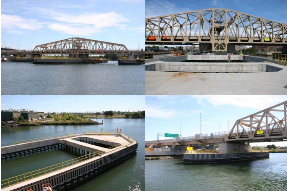
September 2012: Bridge Fender North Elevation Looking South. Bridge South Elevation Looking North. Pier 6 South Fender Looking South. Pier 7 West Face Looking East.
