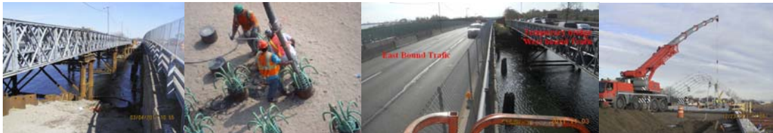
Fresh Creek Bridge March 2011: Westbound Temporary Bridge at Left, Existing Bridge at Right. July 2011: Concrete Pouring in Piles. November 2011: The Remaining Bridge Carrying East Bound Traffic and Temporary Bridge Carrying West Bound Traffic. (Credit: NYSDOT) December 2011: Commenced Installation of Winter Tent Enclosure for Stage IIB Concrete Bridge Deck Placement. (Tent Credit: Daniel Horn)
