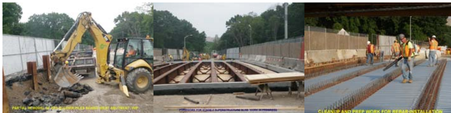
June 2012: Removing Soldier Piles Behind the West Abutment. June 2012: Formwork for Stage 2 Superstructure Slab. July 2012: Formwork for Stage 2 Deck.
