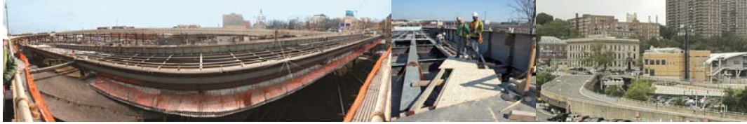
January 2011: Panoramic View. March 2011: Ramp D South Side Fascia Repair. Existing North Ramp (Foreground) and New North Ramp (Background).
