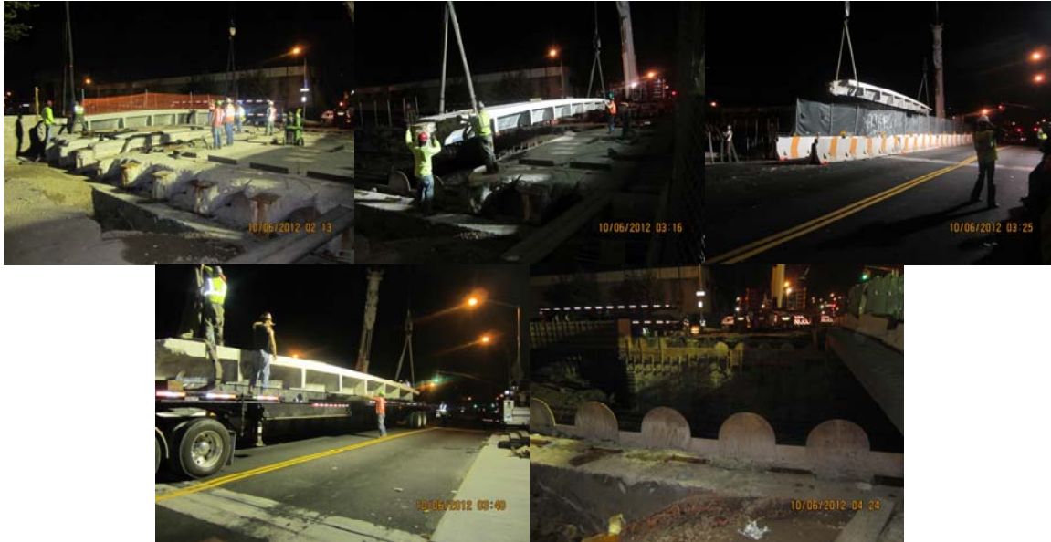
October 2012: Second Stage Demolition: Removal of the Remaining Portion (10 Concrete-Encased Steel Girders) of the Existing Bridge Superstructure.
