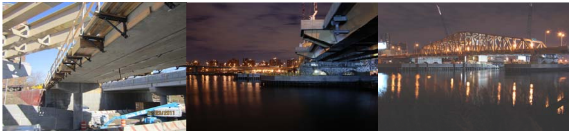
February 2011: Pedestrian/Bicycle Bridge and Ramp to Major Deegan Expressway. September 2011: Granite Installation for Approach to Connector Ramp. Bridge in November 2011. (November Credit: Hardesty and Hanover)
