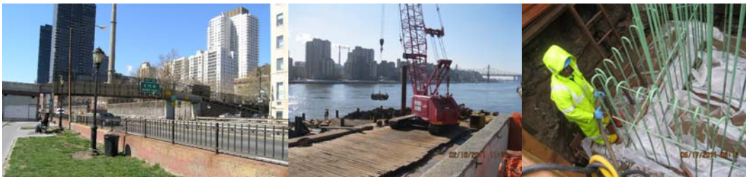
Old East 78 th Street Bridge. February 2011 at the East Ramp Area: Installing Interim Steel Sheeting on East Side, at Pier Footings # 10 and 11. May 2011.
