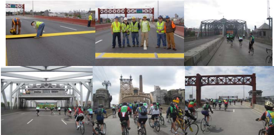
Preparing the Pulaski Bridge for the Bike Tour by Installing Plywood Covers Over the Finger Joints. Blowing Out Debris, Placing the Plywood Board, and Taping into Place: Carpenters Mark Pavia, Michael Short III, and Patrick Burns. Completed Job: Carpenter Patrick Burns, Supervisor Carpenter John Motylewski, and Carpenters John Green, Andrew Myjer, Michael Short III, and Mark Pavia. (Credit: Paul Schwartz) Cyclists on the Madison Avenue, Third Avenue, Ed Koch Queensboro, and Pulaski Bridges. (Credit: Mark Feinman)
