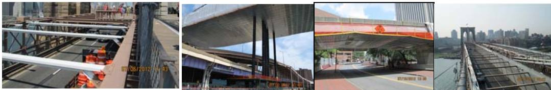
July 2012: Painting Brooklyn-Bound Top Struts. Manhattan Side Span Blasting in Progress. Platform Installation at Ramp E. August 2012: Manhattan Main Span Vertical Wall.
