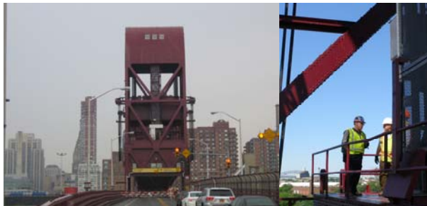
Roosevelt Island Bridge Preparing to Open. (Credit: Kevin Hillery) Executive Director of Bridge Preventive Maintenance and Repair Thomas Whitehouse Inspecting the Bridge. (Credit: Bojidar Yanev)
