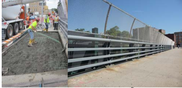
Placing Concrete for Northeast Sidewalk on the 37 th Street Bridge. New Fence and Railing.
