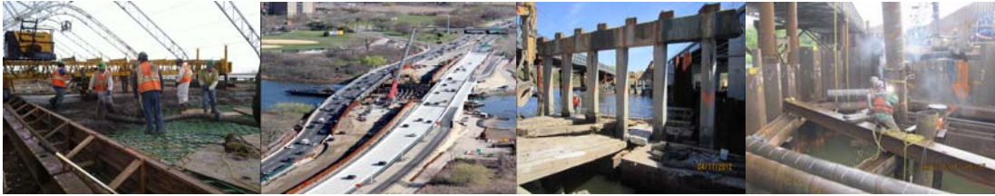
Fresh Creek Bridge in February 2012: Concrete Placement. Fresh Creek Bridge in April 2012: Facing East. New Eastbound Approach Roadways, Bridge Deck, Bicycle/Pedestrian Walkway on Right. Temporary Bridge for Westbound Traffic at Left. Old Bridge Demolition at Center. Fresh Creek Facing East. Stage 3 Demolition of Piers of Old Fresh Creek Westbound Bridge. Workers Cutting off Excess Steel Pipe Casing for Cast-in-Place Concrete Piles at Future Westbound Bridge. Temporary Bridge at Left.
