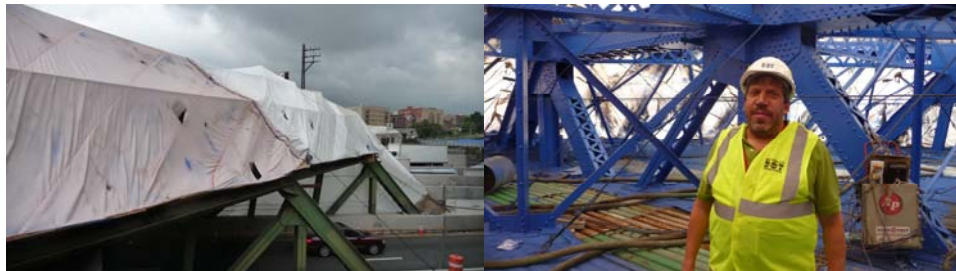
Painting of the Southbound Bridge Truss in September 2012. (Credit: Richard Solomon). Associate Project Manager Richard Solomon Inspecting Inside the Containment.
