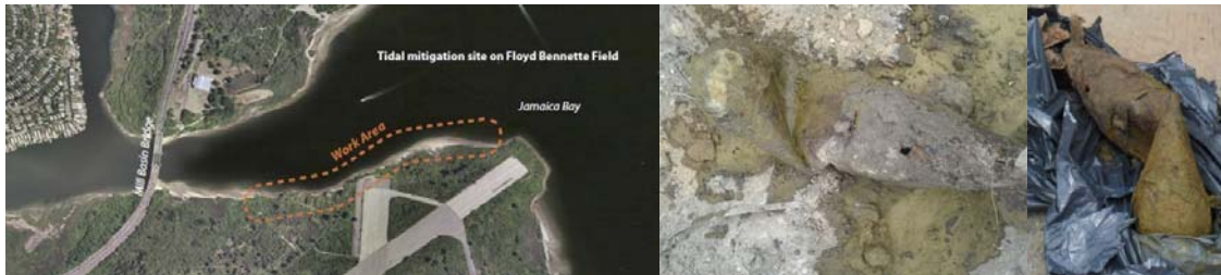
Tidal Wetland Mitigation Site. On June 16, 2011, Work Stopped When Ordnance was Found During Excavation at the Mitigation Site, Floyd Bennett Field. The Bomb Squad was On-Site to Inspect and Remove the Items, Which Were Determined to be Inert World War II Era Torpedoes That Were Buried at the Site.
