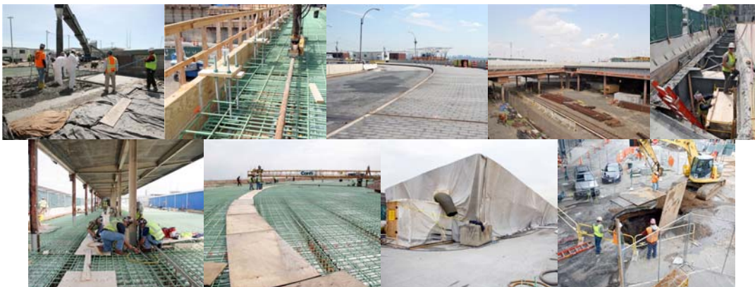
April 2012: BSN Overlay, Towards South. North Ramp, East Approach. June 2012: Ramp B, Looking East. September 2012: BSS West. Old Viaduct West. BSS, Span 2 East. Ramp B Span 19 Southwest. November 2012: BSS Ramp C Containment. Bay Landing Drainage Work.
