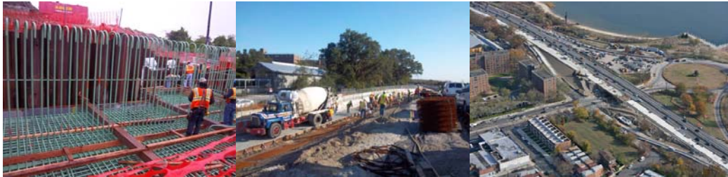
May 2011: Preparing Rebar for Northeast Abutment Footing. October 2011: Pouring Concrete for Northeast Approach. Aerial View in November 2011.
