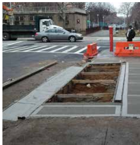
The sidewalk and curb that were removed for the installation are replaced in kind. The new curb has one or two curb cuts that allow water to flow in and out of the bioswale.
