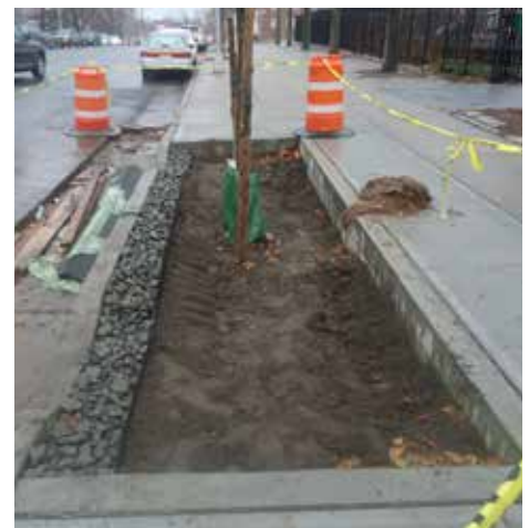
The engineered soil contains sand, which allows for quick infiltration. The soil is graded to allow water to pond at the center of the bioswale during a rainstorm.
