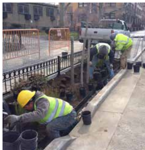
All bioswales feature water- and drought-tolerant perennials that can survive in city streets. Bioswales include trees wherever possible.
