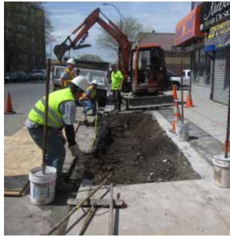
The sidewalk and curb are removed and the material underneath is excavated to a depth of five feet.
