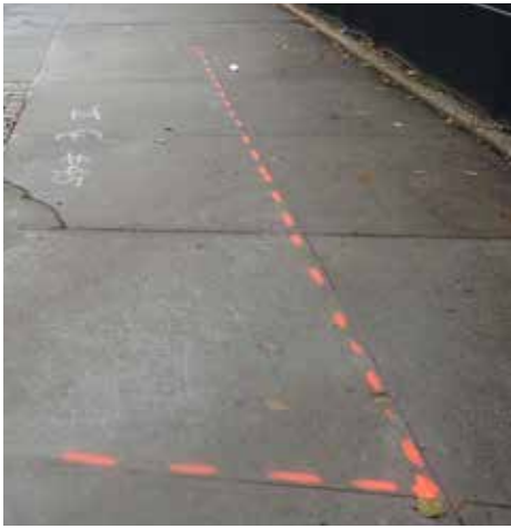
The contractor spray paints the length and width of the bioswale on the sidewalk. These borders are then cut with a saw.
