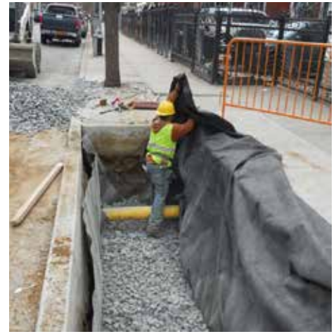
The excavated bioswale is backfilled with broken stone, which is wrapped with geotextile fabric to prevent the next layer of soil from clogging void spaces in the stone layer.
