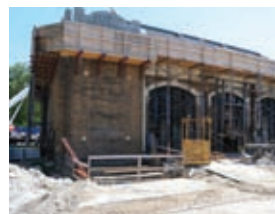
Avenue V Pumping Station
