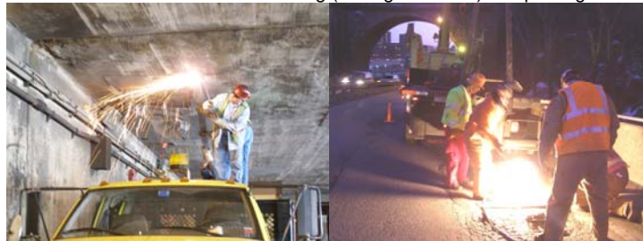
PIA Flag (Truck Wedged Under the FDR Drive at Span 41): Removing the Debris. (Credit: Victor Sandoval) PIA Flag Repair (Through Hole) on Harlem River Drive Ramp. (Credit: Bojidar Yanev)
