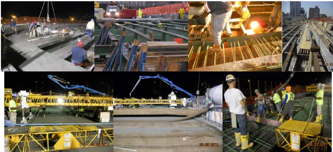
11 th Avenue Viaduct Construction in February 2011. April 2011: New Bridge Deck Formwork. May 2011: Installation of Bridge Deck Formwork for Spans 5, 6, 7 & 8 in Stage 2. June 2011.
