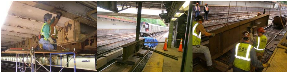
Flag Repairs on the Beverly Road Bridge. Bridge Repairer and Riveters Neil Dalton, Brook Budd, and Daniel Jerderlinic. (Credit: Hany Soliman)
