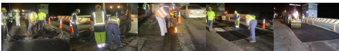
Resurfacing the Belt Parkway Bridge over Mill Basin on August 3, 2009. The Crew Completed a 13'x29' Cut in the Eastbound Center Lane, West Approach Spans. The Area Exhibited Rutting, Cracking and Excessive Patching. Breakout and Removal of Deteriorated Wearing Surface. Ironworker Assisting the Crew. Installation of New Asphalt. (Credit: Yousef Demis) Compacting the Asphalt With the Assistance of a Gasoline Roller Engineer From the Roadway Repair and Maintenance Division. (Credit: Ali Mozaffari)
