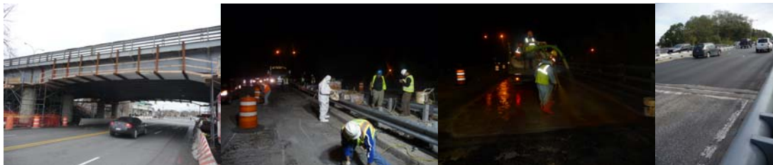
Repairing the Belt Parkway Bridge over Ocean Avenue. The Bridge on October 18, 2011.
