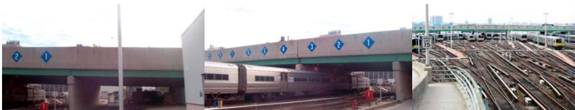
11 th Avenue Viaduct Site (West 30 th Street to West 33 rd Street) in 2006. (Credit: NYSDOT)
