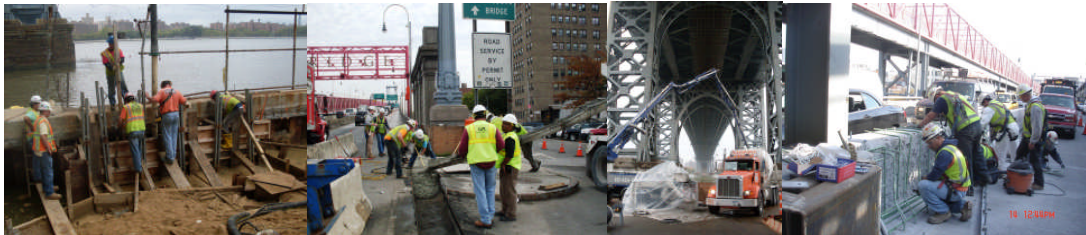
September 2011: Looking West at the Class GG Tremie Concrete Placement for the Kent Avenue Bulkhead Vertical Wall. October 2011: Looking East at the Placement of Concrete Footing for the New Lane 8 Precast Barrier at the Manhattan Plaza. October 2011: Looking West at the Concrete Placement for the Kent Avenue Yard Bulkhead Rehabilitation. November 2011: Looking East at the Rebar Installation for the Cast-in-Place Transition Barrier on the Brooklyn Approach.
