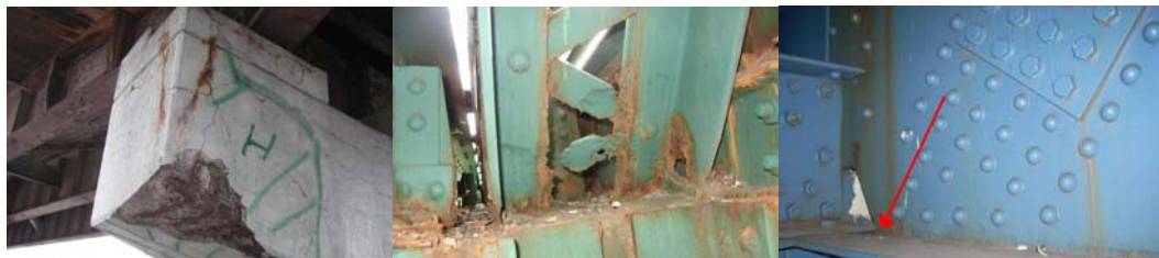
February 2008: Yellow Structural Flag Due to the Deteriorated Cap Beam. October 2008: Corrosion of Steel Secondary Member. November 2008: Crack in Steel Girder.
