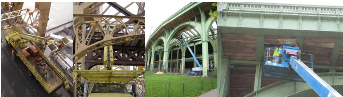
Emergency Inspection of the Queensboro Bridge in February 2011. (Credit: Bojidar Yanev) Inspecting Miller Highway Shielding at 72 nd Street in April 2011. (Credit: Russell Holcomb)
