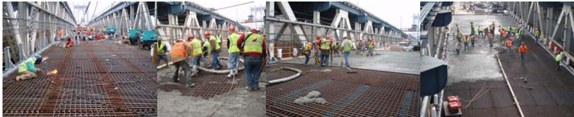
Installation of Full Width Grid Deck Panels on the Manhattan Bridge Lower Roadway in 2006. Pouring the Concrete.
