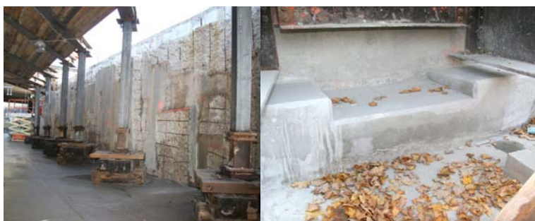
Temporary Shoring of Stringers at Ramp D East Abutment for Steel Repair Work. November 2010: New Bridge Seat and Pedestals Installed at Ramp D West Abutment.
