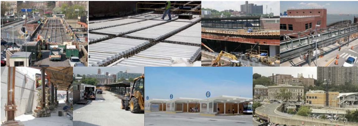
April 2011: Steel Replacement and Rivet Bursting at Ramp D. May 2011: Stay-in-Place Forms and Studs. Overhang Brackets. View of Pedestrian Breezeway Facing East. Ramp D East Abutment. Old Bus Gate. The Refurbished Bus Gates A and B Will Include Enhancements for Pedestrian Safety and Comfort, as Seen in this Rendering. Existing North Ramp (Foreground) and New North Ramp (Background).
