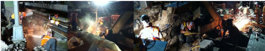
Southbound Bridge Existing Deck Demolition and Deck Panel Installation. August 2011: Stage 2 Assembling and Welding Steel Packs for Southbound Bridge.
