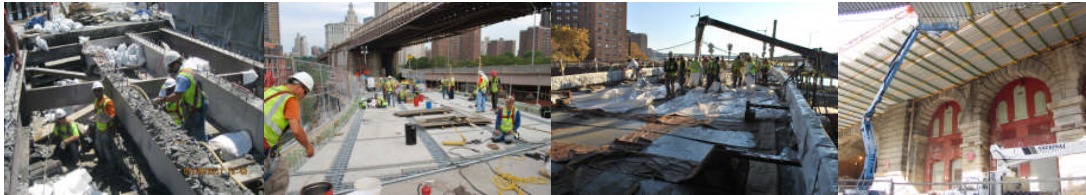
Summer 2011: Manhattan Approach - Ramps A and C Deck Replacement. November 2011: Ramp A and Working Near Arch. (Arch Credit: Jagtar Khinda)
