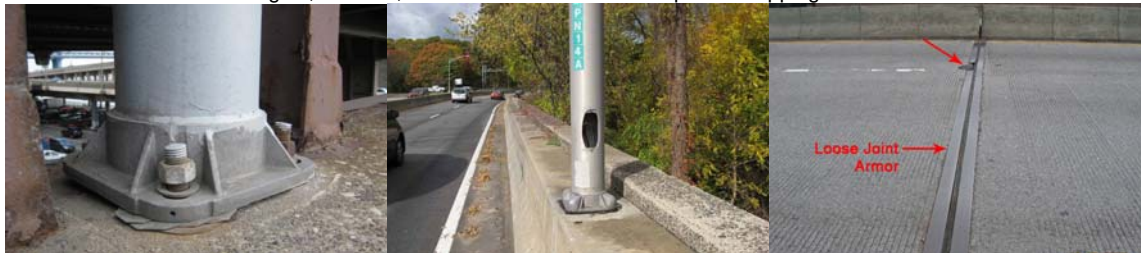
February 2008: Loose Bolts at the Lighting Base. October 2008: Electrical Hazard, and Loose Joint.
