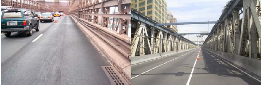
Brooklyn Bridge Wearing Surface. Manhattan Bridge Wearing Surface and Safety-Shaped Barriers. (Credit: NYSDOT)
