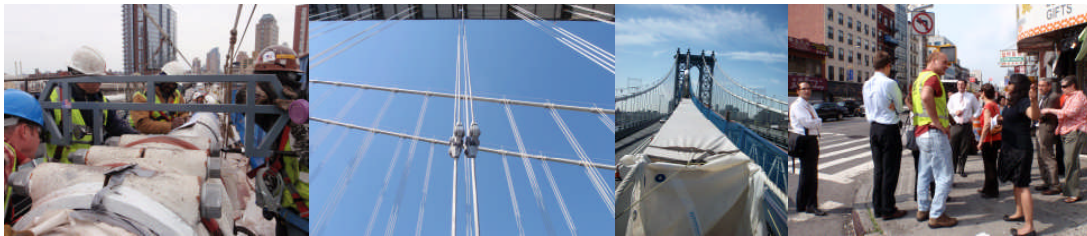
April 2011: Checking Bolt Tension in New Cable Band Bolts. New Suspender Assembly on 'C' Truss. May 2011: Painting Main Band Cables. June 2011: Reviewing the Bikeway Detour – Assistant Commissioner of Traffic Management Ryan Russo, Director of Bicycle and Pedestrian Programs Joshua Benson (Back Turned), Manhattan Bridge Engineer-in-Charge Brian Gill, Bicycle Program Coordinator Hayes Lord, First Deputy Commissioner Lori Arditto (Orange Top), Deputy Commissioner Gerard Soffian, and Chief Staff Manager/Executive Director of Community Affairs Joannene Kidder (at Right).
