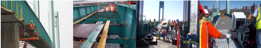
January 2011: Under-Deck Shield Installation for Manhattan Approach Span 6. April 2011: Removing Concrete Decking Material. June 2011: Pouring Concrete Decking at Span 7.
