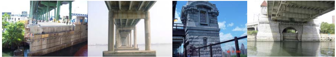
Pier 1 of Hamilton Avenue Bridge. Pier 17 of Rikers Island Bridge. Pier 1 of Hunters Point Avenue Bridge. Ed Koch Queensboro Bridge Pier. Pier 35 of Macombs Dam Bridge. (Credit: NYSDOT)
