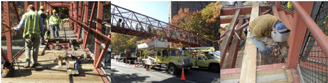
Repairing the PS-5 Bridge: Carpenters Adam Muhleisen and John Horgan, and Assistant Civil Engineers Fouad Althaibani and Sohrab Hossain. Supervisor Highway Repairer Joseph Flood and Interim Director of Bridge Preventive Maintenance Paul Schwartz (at Left). Bridge Repairer and Riveter John McAllister. (Credit: Thomas Whitehouse)
