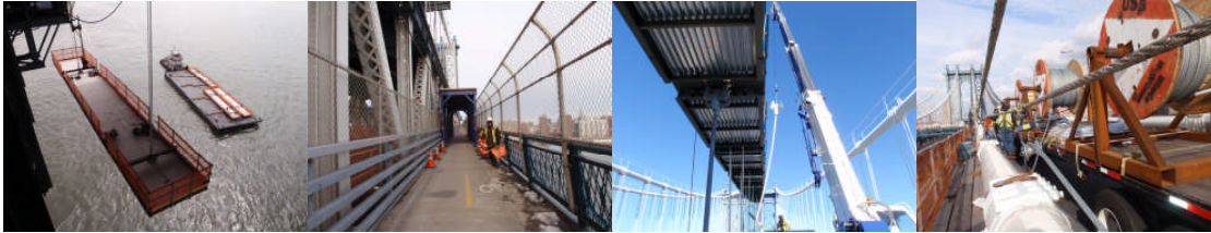
July 2010: Installation of Under Deck Work Platform at Manhattan Tower. January 2011: Bikeway Protection Shed on North Path. March 2011: Removal of Existing Suspender, 'C' Truss. April 2011: Installation of New Hand Ropes for 'C' Cable.
