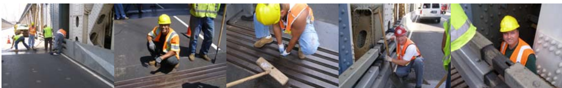
Manhattan Bridge Expansion Joint Cleaning in 2008: Supervisor Highway Repairer Thomas Cruz, Assistant City Highway Repairer Antonio Asaro, Highway Repairer Louie Dumeng, and Oiler Stanley Karolewicz. Assistant City Highway Repairers Jonathan Adorno and Antonio Asaro, Oilers Stanley Karolewicz and Ronald Grady. (Credit: Thomas Whitehouse)
