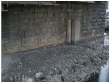
Eroded Riprap Pier Protection at Pier 11 of Old Willis Avenue Bridge in 2008. (Credit: NYSDOT)
