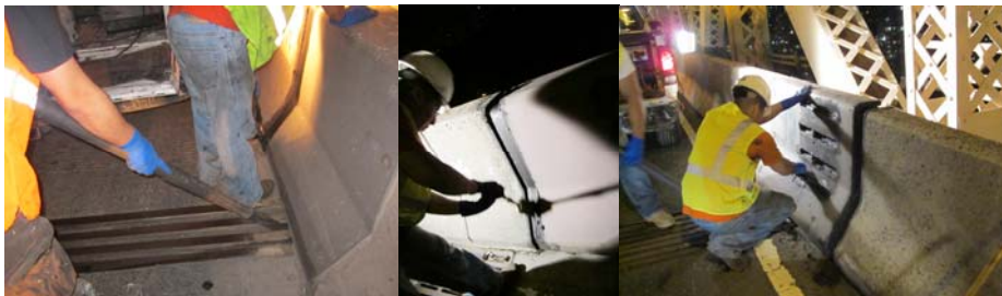
Expansion Joint Cleaning on the Williamsburg Bridge in September 2011. (Credit: Shaikh Islam)
