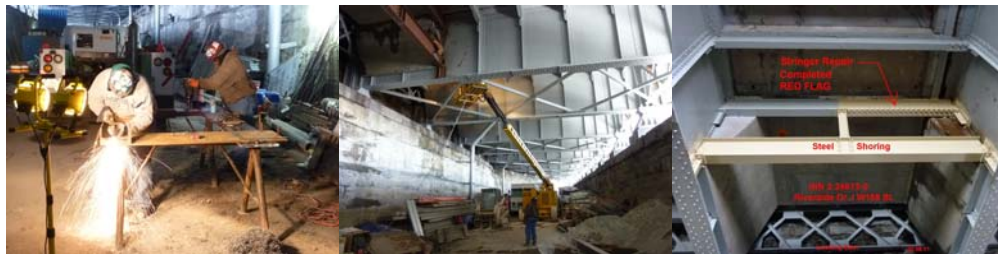
February 2011: Red Flag Stringer Repair at Riverside Drive Viaduct over West 158 th Street.
