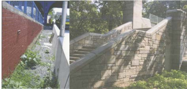
East Approach Cladding on the East 174 th Street Bridge. Abutment Wingwall Cladding on the West 173 rd Street Bridge.
