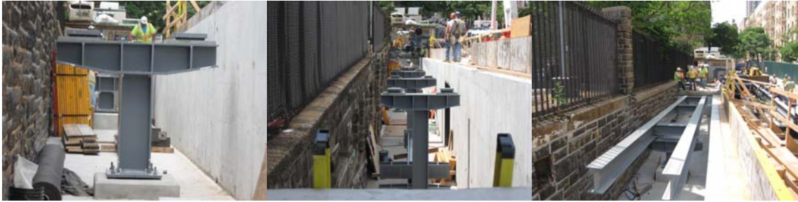
July 2011: Steel Erection for the West Side Ramp Along the North Side of John Jacobs Park.
