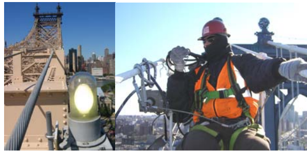
A Bulb of the Ed Koch Queensboro Bridge Necklace Lights. (Credit: Peter Basich) Repairing a Manhattan Bridge Necklace Light. (Credit: Hany Soliman)
