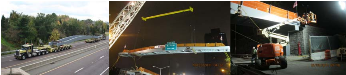
The New Bridge Span in Transit from Just North of Philadelphia to Jersey City. It was Then Loaded on the Barge and Brought up the East River to the Site. The Span Size was 26' x 135' and Weighed Approximately 80 Tons. New Main Span Steel Erection in October 2011.
