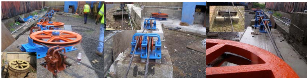
Carroll Street Bridge Pulling Cable System – Before and After. (Credit: Emily Colasacco)
