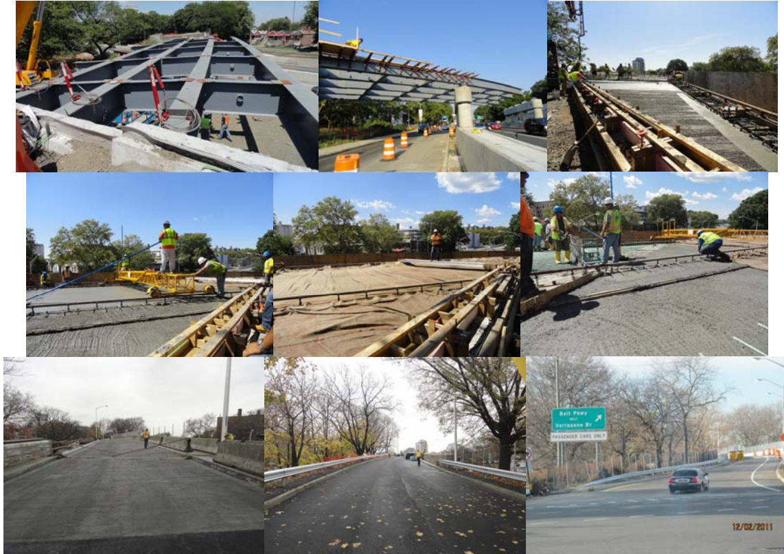
East 8 th Street Ramp in June 2011: Steel Installation for Span 1. July 2011: Installation of Steel Girders over the South Service Road and Eastbound Belt Parkway. August 2011: Concrete Deck Placement. November 2011: Completed North and South Approach Roadways. December 2, 2011: Bridge Open to Traffic.
