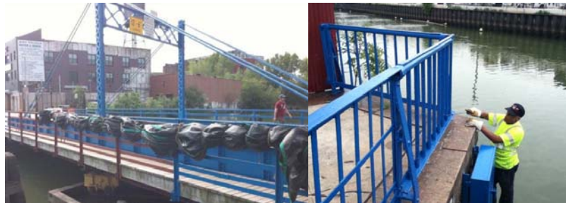
Painting of the Bridge in Progress. Bridge Painter Joao Silva Applying Top Coat to Hand Rails.
