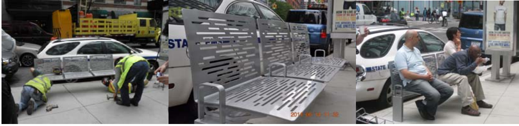
Bridge Repairer and Riveter Ignazio Trapani Drilling the Holes for the Concrete Anchor Bolts to Hold the Bench Securely in Place. Bridge Repairer and Riveters Ignazio Trapani, Fabian Del-Tongier and Salvatore Dimuro - Final Tightening of the Bolts and Installation of the Cover Plates to Hide the Connections. (Credit: Thomas Whitehouse) Bench Prototype and Testing by Citizens.
