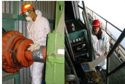
Division Staff Installing Strain Gauges in 2006 on the Greenpoint Avenue Bridge. Checking the Measurements. (Credit: Vera Ovetskaya)
