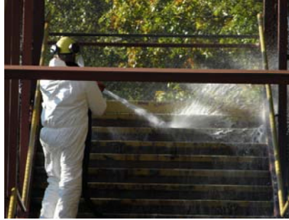
Highway Repairer Ruben Sanchez Washing the Staircase at the PS-5 Pedestrian Bridge over 10 th Avenue in Manhattan in November 2011. (Credit: Joseph Flood)
