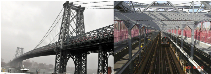
Williamsburg Bridge in February 2010. (Credit: Samuel Teaw). Looking West at the Overhead Trusses in November 2010. (Credit: NYSDOT)
