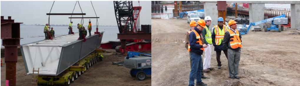
First Major Steel Erection at the Paerdegat Basin Bridge in April 2011. Observing the Placement of the Tub Girder Sections: Administrative Engineer Daniel Hom, Civil Engineer Edvard Jeamgocian (Obscured), Consultant Project Manager Bill Ferdinandsen, and Civil Engineers Ferdinand John and Jagdish Patel.
