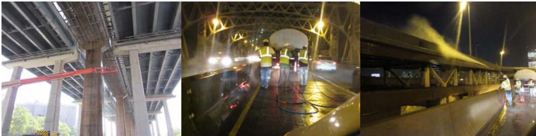
Washing the Williamsburg Bridge in July 2011 and the Ed Koch Queensboro Bridge in August 2011.
