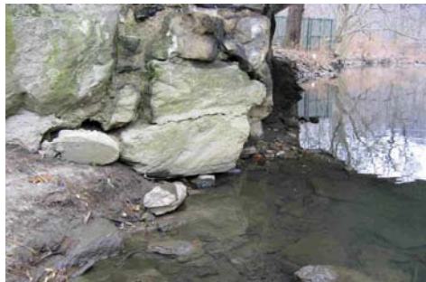
Scour on Pier 2 End Face of Mosholu Parkway Bridge Over Bronx River in 2008. (Credit: NYSDOT)
