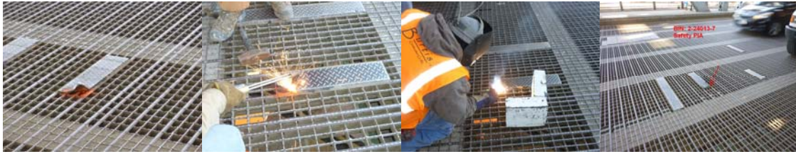
Addressing a PIA Flag on the Broadway Bridge in February 2011.
