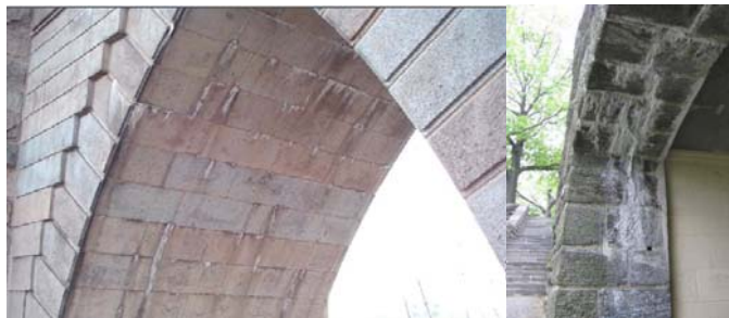
Moderate Efflorescence on the Brooklyn Bridge Brooklyn Tower North Gothic Arch in 2004. (Credit: NYSDOT) Efflorescence on the Underside of the Masonry Stones on the End Abutment of the Margaret Corbin Drive Bridge over Pedestrian Path Near Café.
