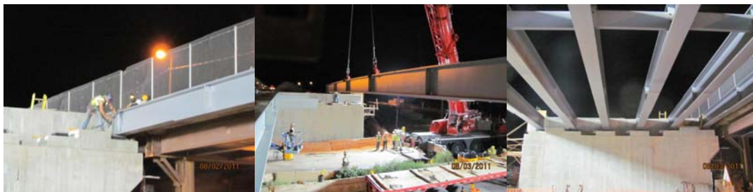
Completing the Steel Erection for the Northern Section in August 2011. (Credit: Daniel Hom)
