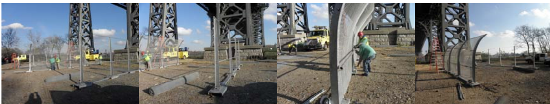
Assembling Three Pedestrian Prototype Fence Sections (Curved, Angled, and Straight), That Were Installed Underneath the Williamsburg Bridge in East River Park In December 2011. (Credit: Thomas Whitehouse)
