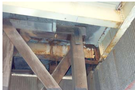
Timber Shoring Supporting a Failing Steel Beam – a Potential Winter Hazard.
