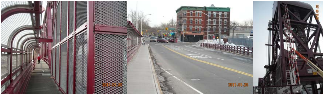
January 2011: North Sidewalk With New Pedestrian Fence. Vernon Boulevard and 36 th Avenue Intersection With New Turn Lane. Recently Painted Bridge With New Traffic Control Equipment.
