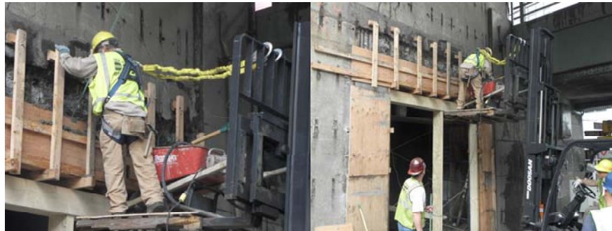
Performing Structural Repairs of the Entrance to the Cellular Structure at Joralemon Street Under the Brooklyn-Queens Expressway Triple Cantilever in June 2011. Loose Concrete was Removed and Replaced, and Rebar was Cleaned and/or Replaced. Cement Mason Victor Porowski Placing Concrete in the Forms While Standing on a Wooden Platform Raised by a Hi-Lo. He is Wearing the Appropriate Fall Protection Gear. Bridge Repairer and Riveter Brook Budd, Cement Masons Victor Porowski on Raised Platform and Lawrence Marks Operating the Hi Lo, and Carpenter Stephen Buckley. (Credit: Thomas Whitehouse)
