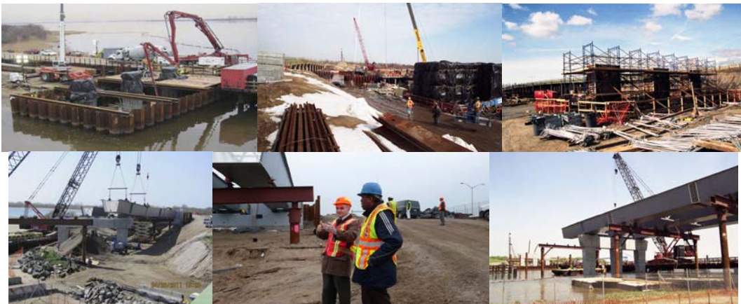
February 2011: Pumping Concrete at Paerdegat Basin Cofferdam for Pier No.3. February 2011. March 2011. April 2011: Setting Tub Girder Sections at Eastbound Bridge Between West Abutment and Pier No. 1. Civil Engineers Edvard Jeamgocian and Ferdinand John Observing the Operation. May 2011: Eastbound Bridge – New Concrete Pier No. 2 and Temporary Supports for Tub Girders.
