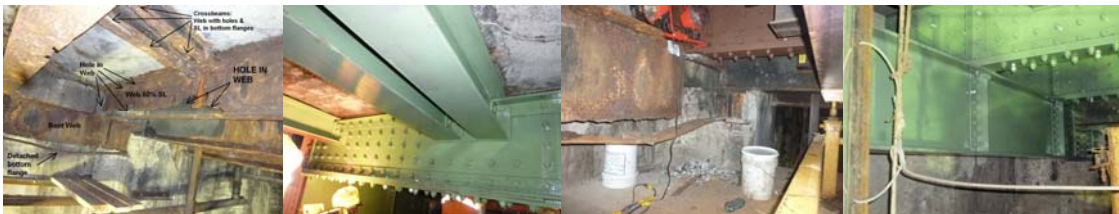
73 rd Street Pedestrian Bridge Over Amtrak – Red Flag Repair of the Steel Beam Grid. Span 5 – Stringer S3 Exhibited Severe Corrosion With Holes. After Repair with Bolted Web Plates. Span 5 – Floorbeam exhibited Severe Deterioration on Web and Bottom Flanges. Span 5 - New Floorbeam Under Stringers S2 & S3. (Credit: Artemio Angeles)
