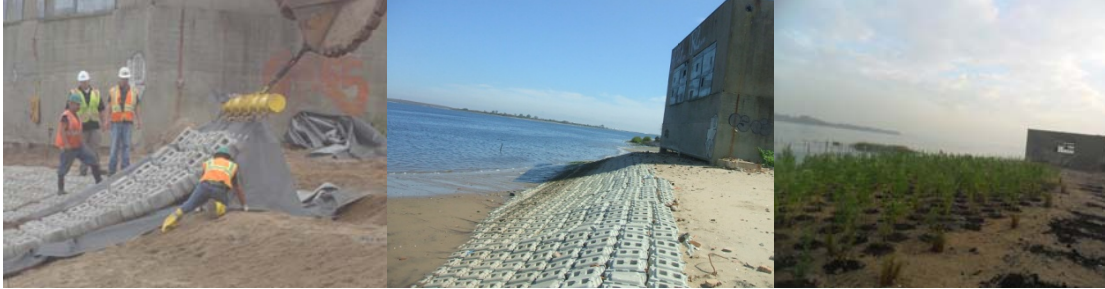
Summer and Fall 2011: Installing the Revetment. An Articulating Concrete Block Revetment System is Used as Slope Protection in Front of the Existing One Story Warehouse Building. Planting Bayberry; Groudsell Trees; Beach Plum Plants, and SwitchGrass.
