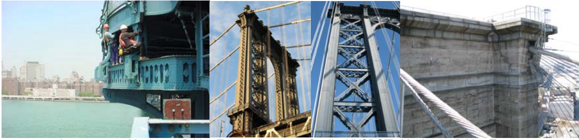
Inspectors on Manhattan Bridge Tower. (Inspector Credit: NYSDOT) Manhattan Bridge Tower. (Credit: Michele N. Vulcan) Manhattan Bridge Tower Detail. (Credit: Russell Holcomb) Brooklyn Bridge Brooklyn Side Tower Detail. (Credit: Jagtar Khinda)
