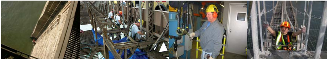
Repairing the Brooklyn Bridge Standpipe System, 130 Feet Below the Roadway. Maintenance Crew Conducting the Annual Cleaning and Lubrication of the Solid Rod Suspenders Spherical Bearings on the Brooklyn Bridge. (Credit: Anatoly Orlov) Oiler T. McAuliffe at the 9 th Street Bridge. Assistant Mechanical Engineer Vera Ovetskaya Climbing to the Brooklyn Bridge Tower in 2008. (Credit: Gennadiy Kaplun)
