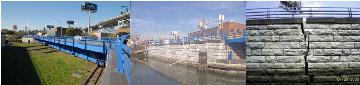
Borden Avenue Bridge. (Credit: Peter Basich) General and Close Up View of the Crack in the Wingwall. (2 nd View Credit: NYSDOT)
