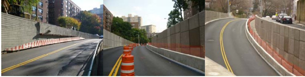
Kappock Street Retaining Wall in Riverdale, Before and After Repairs. The Existing 300-Foot Long Parallel Concrete Roadway Retaining Walls on Both Sides of Kappock Street Were Deteriorated and Leaning, and Were Replaced with New Modular Retaining Walls in the Summer of 2009.
