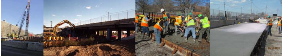
Rockaway Parkway Bridge in February 2011: Driving Steel Pile for Cast in Place Concrete Piles at East Abutment. March and April 2011.
