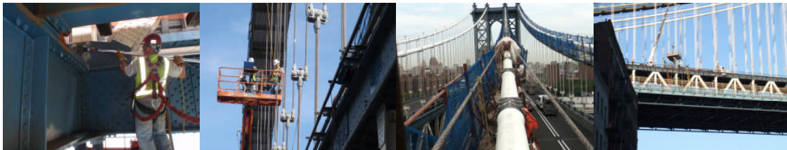
August 2011: Repairing Gusset Plates, Checking Bolt Tension. Checking Suspender Loads With an Accelerometer. Installing Containment on Cable D. October 2011: Installation of Transit Platforms.
