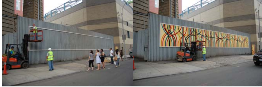
Bridge Repairer and Riverter Yiu Liu, Supervisor Carpenter Joseph Vaccaro, and Carpenters Stephen Buckley and Joseph Moschella Installing the Mural. (Credit: Doneliza Joaquin for DUMBO NYC)
