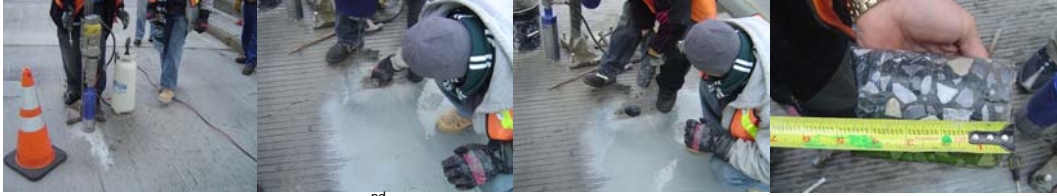
Removing a Core From 252 nd Street Bridge over Henry Hudson Parkway in January 2009. (Credit: Masroor Mahmood)
