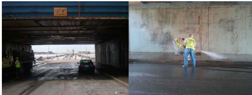
Bridge Painters Nicholas Krevatas and Branko Grzancic Removing Graffiti. (Credit: Earlene Powell)
