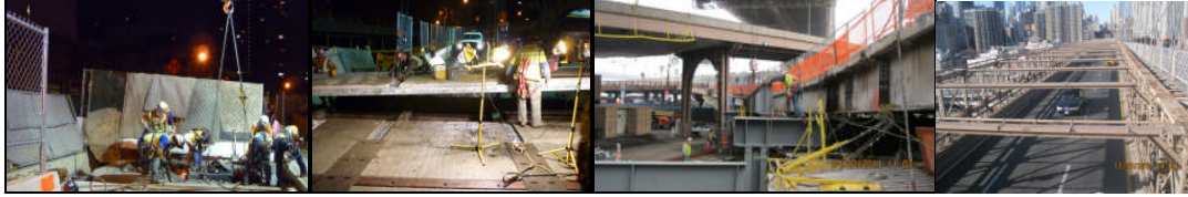
May 2011: Sound Dampening Fence Used as Sections of Roadway Around the Manhattan Approach Outside Pace University Are Saw Cut and Removed. Brooklyn Bridge Manhattan Approach Deck Replacement. Southbound FDR Drive Ramp - April 2011 Steel Erection. December 2011: Painted Top Struts of the Brooklyn-Bound Manhattan Side Span.
