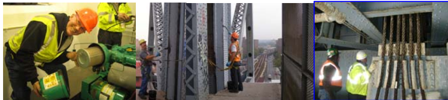
Oiler Tom Strommen Maintaining the Hydraulic Power Unit at the Hamilton Avenue Bridge in February 2010. (Credit: Vera Ovetskaya) Cleaning and Lubricating the Broadway Bridge. (Credit: Reza Taheri) Executive Director of Bridge Preventive Maintenance and Repair Thomas Whitehouse (Wearing Yellow Jacket) Inspecting the Broadway Bridge Machinery Room and Instructing the Contractor. (Credit: Albert Hong)
