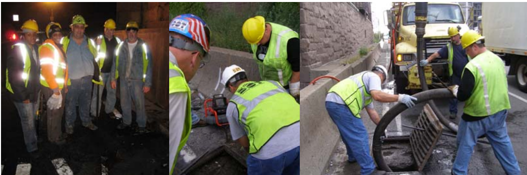
Drain Crew After Hand-Tool Cleaning the Clogged Catch Basins at Night on the Eastbound Brooklyn-Queens Expressway in April 2011: Highway Repairers Linda Rose and Sharon Britt, Supervisor Highway Repairer Joseph Turchiano, and Highway Repairers John Latona and Alfred Black. (Credit: Russell Holcomb) The "SnakeCam" is a Camera that is Fed Into a Drain/Sewer to Show the Crew What is Occurring. Executive Director of Bridge Preventive Maintenance and Repair Thomas Whitehouse, Supervisor Highway Repairer Anthony Irizarry, and Assistant City Highway Repairer John Tammaro Using the Camera on a Drain on the Eastbound Brooklyn-Queens Expressway in September 2011. Supervisor Highway Repairer Anthony Irizarry, Highway Repairer Michael Cunningham, and Assistant City Highway Repairer John Tammaro Using the Scupper Truck to Clean the Drain. (Credit: Paul Schwartz)
