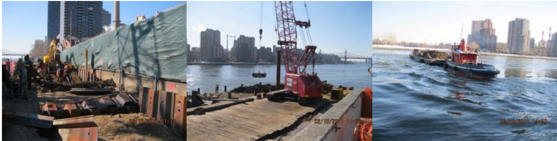
February 2011 at the East Ramp Area: Installing Interim Steel Sheetting on East Side, at Pier Footings # 10 and 11. Debris Loaded out Onto Barge and Removed by Tugboat.
