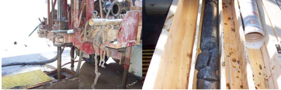
Conducting Soil Borings in 2008 as Part of the Seismic Retrofit Design of the Manhattan Bridge. Drilling to a Depth of Approximately 210 Feet to Obtain an 8-foot Long Hard Rock Sample. A 2 1/2 –Foot Long Hard Rock Sample Taken From a Depth of Between 202 and 204 ½ Feet.
