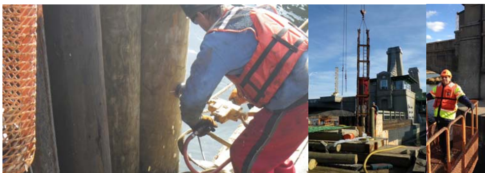
Working on the Shore Road Bridge in December 2011. (Credit: Artemio Angeles) When and Where Contract Unit Director Sudhir Jariwala at the Shore Road Site to Inspect the Fender System Repairs as well as the Safety Flags Repair Under the Arch Spans.
