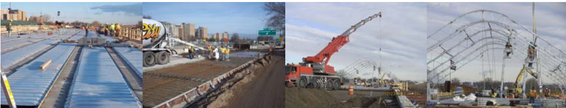
December 2011: Preparing the Decking for the Concrete Pour. Concrete Pours for Southeast and Northeast Roadways. Commenced Installation of Winter Tent Enclosure for Stage IIB Concrete Bridge Deck Placement. (Tent Credits: Daniel Hom)
