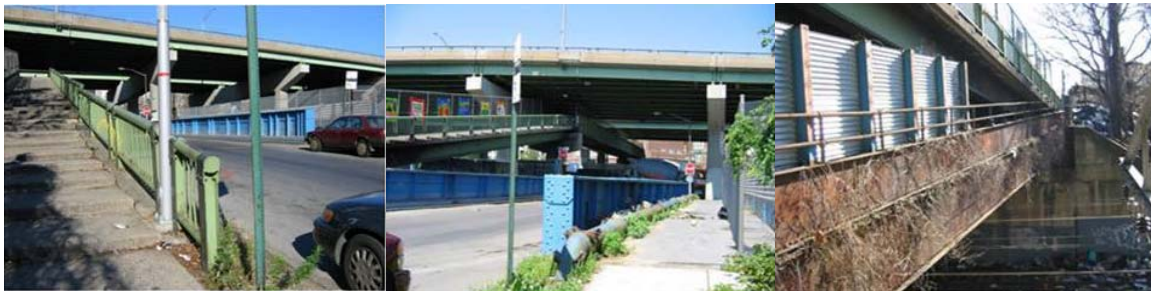
Bryant Avenue Bridge Looking North Towards the North Sidewalk. Looking South Towards the Pedestrian Overpass. Looking East Along the South Fascia of the Bridge.
