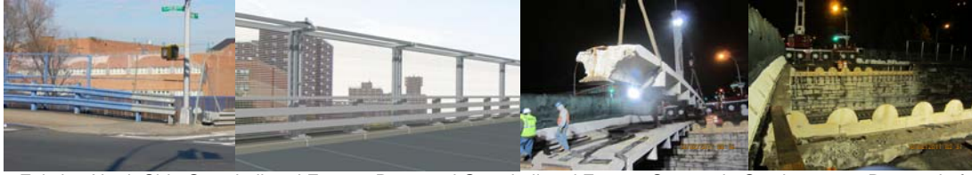
Existing North Side Guardrail and Fence. Proposed Guardrail and Fence. Stage 1 in October 2011: Removal of the Existing Bridge Girders.
