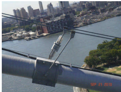
Necklace Light on Williamsburg Bridge Main Cable in September 2010. (Credit: NYSDOT)
