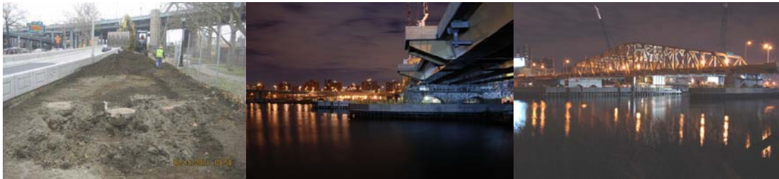
March 2011: Began Landscaping the Area Between the A Ramp Approach and the River. Bridge in November 2011. (November Credit: Hardesty and Hanover)
