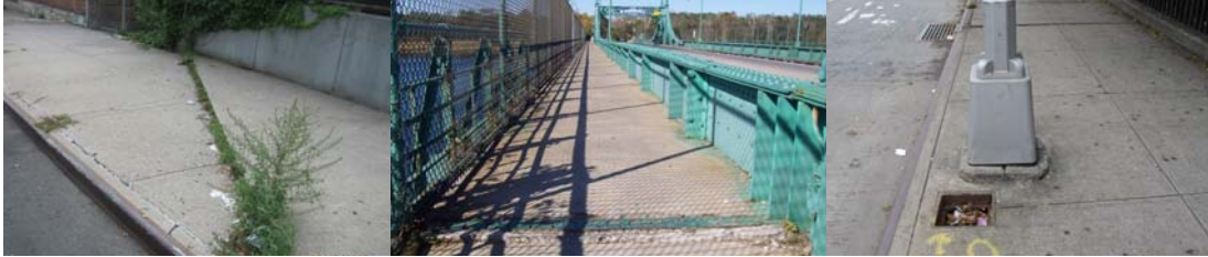
August, October, and November 2008: Examples of Tripping Hazards.
