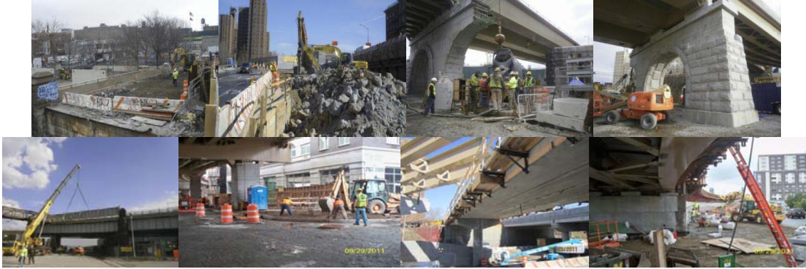
March 2011: Completed Excavation and Disposal of Existing Approach Slab and Roadway Pavements at B Ramp, Stage III. . Completed Excavation and Disposal of Existing Willis Avenue Abutment Footing and North Retaining Footing for Stage 5B Construction. Stage III Caisson Concrete Placement at Caisson #2 at Pier 11. Setting Granite Stone Facing at Pier 11. Finished Stage VB Removal of Steel Girder at South Bay at Existing Span 15. September 2011: Construction of Sidewalk at Bruckner Boulevard. February 2011: Pedestrian/Bicycle Bridge and Ramp to Major Deegan Expressway. September 2011: Granite Installation for Approach to Connector Ramp.
