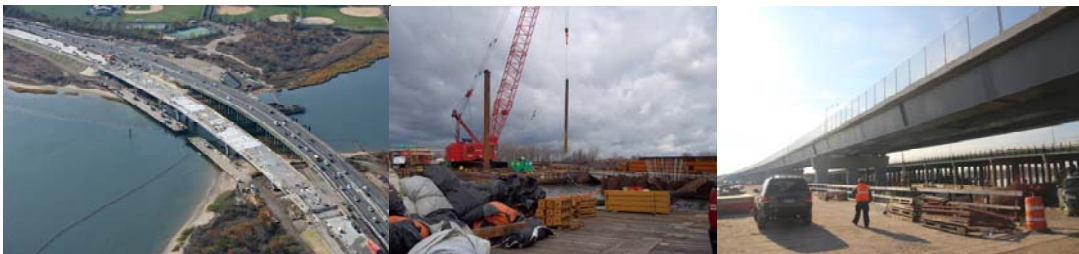
November Aerial View. December 2011: Working Inside the Northern Cofferdam. New Eastbound Bridge.
