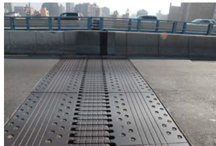
Manhattan Bridge Finger Dam. (Credit: Jagtar Khinda)
