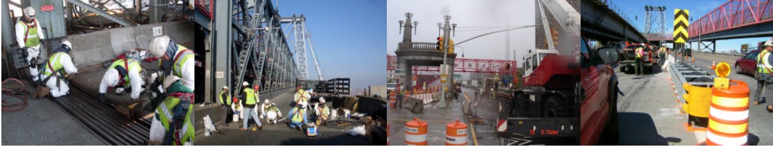
February 2011: Looking North at the Replacement of Existing Modular Joint Seals on the South Inner Roadway. April 2011: Looking North at the Replacement of Existing Modular Joint Seals on the North Outer Roadway. May 2011: Looking North at the Placement of a Temporary Barrier at the Manhattan Plaza in Preparation for the Clinton Street Traffic Signal Relocation Work. September 2011: Looking West at the Installation of the Brooklyn Approach Precast Median Barrier and Attenuator.
