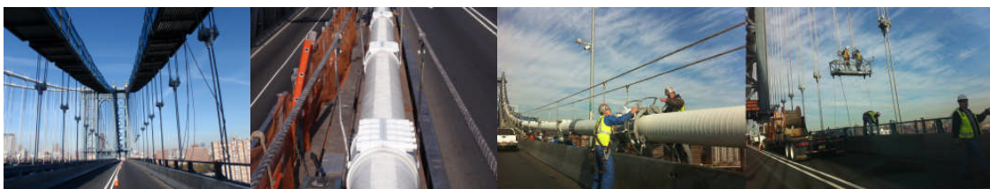
November 2011: New Suspender Assemblies Along 'C' and 'D' Trusses (Temporary Platforms Shown Above). Main Cable Wrapped With Walking Surface. Power Tool Cleaning Cable Circumferences and Grooves.
