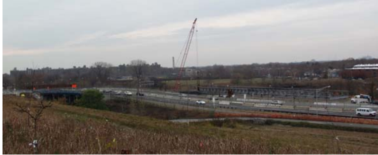
Fresh Creek Bridge in November 2010: Overview of the Existing Bridge and the Installation of the Temporary Bridge and Approaches North of the Existing Roadway. (Credit: Eric Callender)
