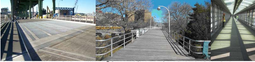
Hamilton Avenue Bridge, and West 8 th Street and Chambers Street Pedestrian Bridge Decks. (Hamilton Credit: NYSDOT)
