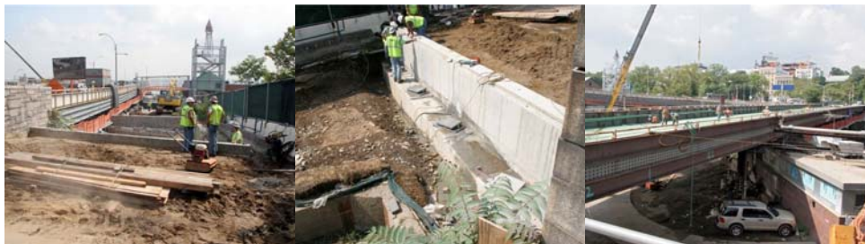
August 2011: Ramp A Looking East. Ramp A West Abutment Pedestals. Ramp D Looking Southwest.
