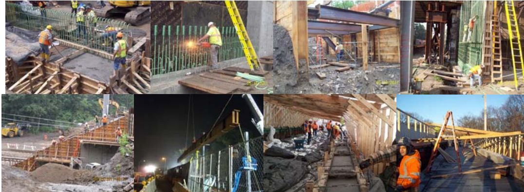
Shore Road Circle Bridge in April 2011 – July 2011. September 2011: Steel Installation. November and December 2011: Concrete Parapet and Deck Placement.
