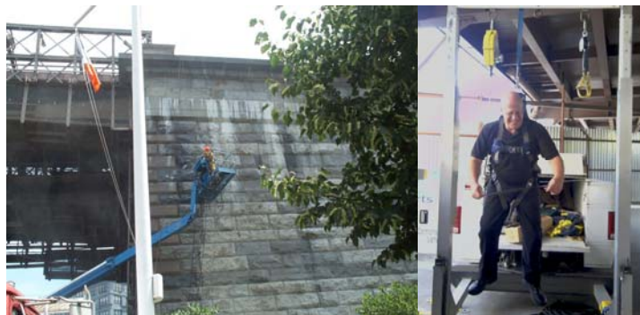
Cleaning the Brooklyn Bridge Brooklyn Anchorage in July 2007. (Credit: Serag Saad) During Fall Protection Training in August 2010, Executive Director of Bridge Preventive Maintenance and Repair Thomas Whitehouse Was Hoisted in the Air While Wearing a Full Body Harness - Demonstrating How to Deploy and Use the Foot Stand to Prevent Orthostatic Intolerance (Commonly Referred to as Suspension Trauma), Which Can be Fatal if Not Prevented. (Credit: Gean Pilipiak)
