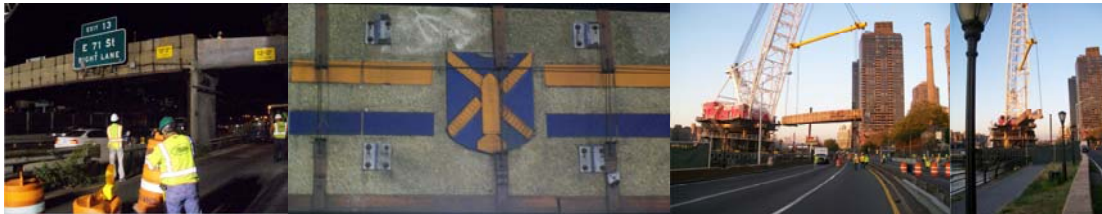
East 78 th Street Bridge Before Demolition. Original Tile Signage. Moving the Bridge to the Barge.
