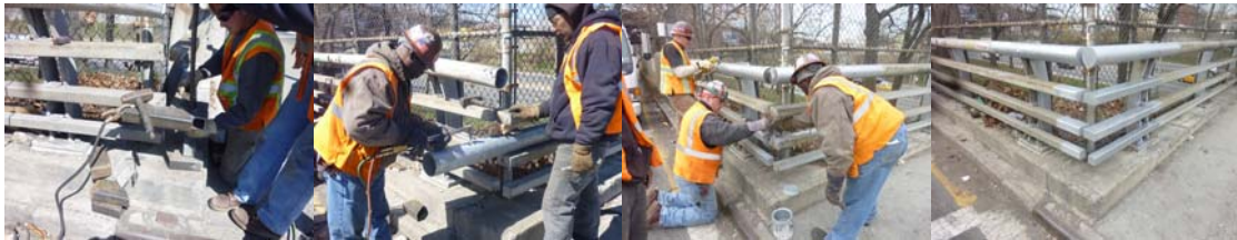
Working on the 44 th Street Bridge over Grand Central Parkway in March 2011. (Credit: Artemio Angeles)
