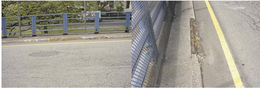
Spalled Section of Curb on the East 8 th Street Bridge in 2006. (Credit: NYSDOT)
