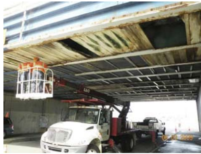
2009 Inspection: The Entire Underside of the Bay Ridge Avenue Bridge Deck is Shielded With Timber Planking and Steel Wire Mesh Netting. The Shielding was Temporary Removed to Perform the Inspection of the Deck. Shielding was Replaced After the Inspection. (Credit: NYSDOT)
