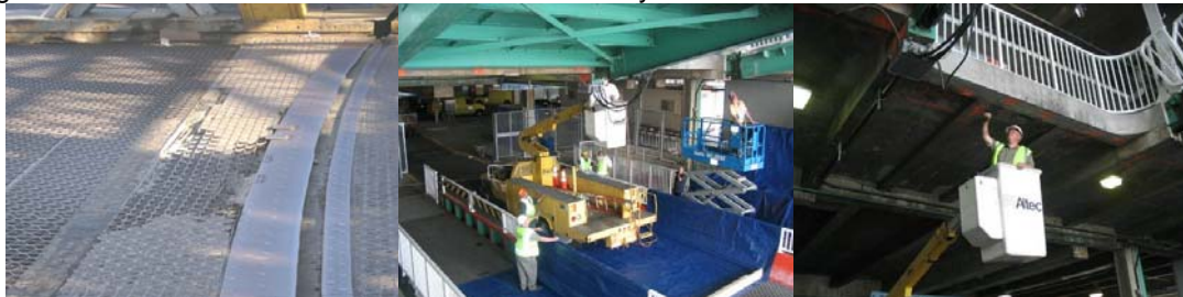
Example of PIA Safety Flag: Broken Grating. Executive Director of Bridge Preventive Maintenance and Repair Tom Whitehouse (White Hardhat) Ensuring the Proper Setup of Containment Procedures at the St. George Ferry Terminal Landing Slips Before the Masons Address A PIA Flag (Falling Concrete). Inspecting the Flagged Condition.
