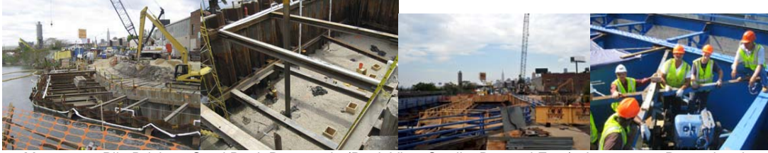
May 2010: Pile Driving. Steel Deck Removed. (Deck View Credit: Bernard Ente) June 2010: Removing the Motor for Replacement and the Main Machinery Shaft for Rehabilitation. Oiler Carl Wharton, Mechanical Engineer Ibrahim Ibrahim, Oilers Tom Strommen and Richard Morreale, and Construction Project Manager Ali Mozaffari. (Credit: Vera Ovetskaya)
