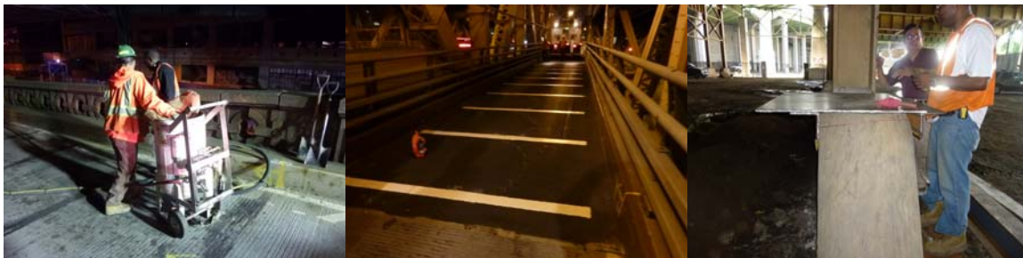
Working on the Ed Koch Queensboro Bridge in September and October 2011. When and Where Contract Unit Director Sudhir Jariwala (Background) Inspecting Repair Materials at the Henry Hudson Viaduct in September 2011.
