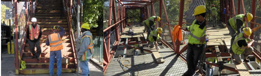
Repairing the PS-5 Bridge: Director of Bridge Repair Pinakin Patel and Highway Repairers Joseph Davis and George Lee. Carpenters John Horgan and Ruben Urena, and Assistant Civil Engineer Fouad Althaibani. Carpenters Adam Muhleisen, John Horgan, and Ruben Urena. Electrician Angelo Tubiolo. (Credit: Thomas Whitehouse)
