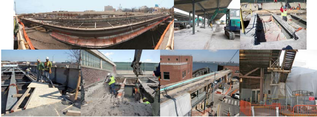
January 2011: Panoramic View. February 2011: Sidewalk and Decking Demolition at Bus Station North. March 2011: Ramp D South Side Fascia Repair. Kiosk Wall Demolition. Breezeway Containment and Abatement.
