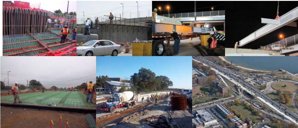
May 2011: Preparing Rebar for Northeast Abutment Footing. June 2011: New Footing and Wing Walls at Northeast Side. July 2011: Constructing East Abutment, North Side of Belt Parkway. Completing the Steel Erection for the Northern Section in August 2011. (Credit: Daniel Hom) September 2011: Installing Reinforcement Steel for Stage 2 Westbound Lane Decking. October 2011: Pouring Concrete for Northeast Approach. Aerial View in November 2011.
