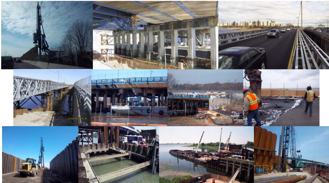
Fresh Creek Bridge in January 2011: Installing Metal Shielding Along Westbound Lane of Belt Parkway. February 2011: Placing Under Deck Protective Shielding. March 2011: Westbound Belt Parkway Traffic Detoured onto the Temporary Bridge. Westbound Temporary Bridge at Left, Existing Bridge at Right. Removing Lead Based Paint From Steel Cut Line Locations. Westbound Lane Demolition. On March 4, 2011, Westbound Traffic was Detoured on to a Temporary Bridge over Fresh Creek Basin, and Eastbound Traffic was Detoured on to the Westbound Belt Parkway Roadway Within the Contract Limits. Demolition of the South Side of the Bridge started on March 22 and Continued into June 2011. On April 7, Demolition Work of the Deck and Stringers of the East Bound Side of the Bridge was Completed. April 2011: Installing Metal Shielding Along Belt Parkway Median. June 2011: Cofferdam on South Side of Existing Bridge Pier No. 1. Driving Piles for the Southeast Abutment.
