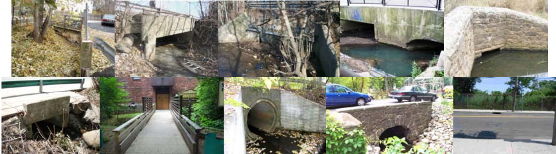
Galloway Avenue over Marianne Street, Forest Avenue over Crystal Avenue. Naughton Avenue over Patterson Avenue, Midland Avenue over Hylan Boulevard. Rockland Avenue over Brielle Avenue, Forest Avenue over Randall Avenue. Gregg Place over Randall Avenue, Arthur Kill Road over Muldoon Avenue. Richmond Hill Road over Richmond Road, Arthur Kill Road over Ridgewood Avenue.
