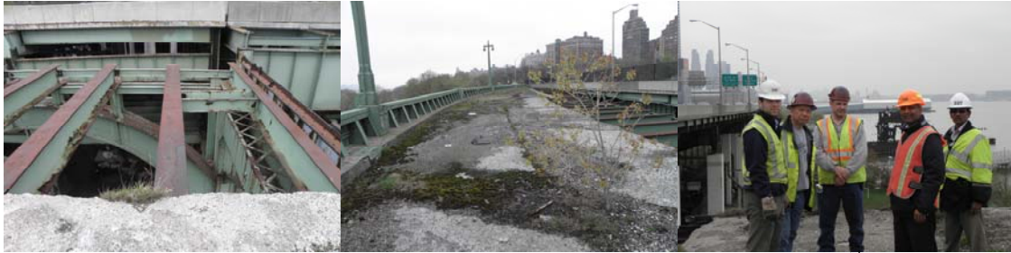
Inspecting a Loose Concrete Safety Flag at the Abandoned West Side Highway Ramp at 72 nd Street and Riverside Park in May 2011: Interim Director of Bridge Preventive Maintenance Paul Schwartz, Bridge Repairer and Riveter Liu Yiu, Supervisor Bridge Repairer and Riveter Gean Pilipiak, Director of Bridge Repair Pinakin Patel, and Engineer-in-Charge Bala Nair. (Credit: Thomas Whitehouse)
