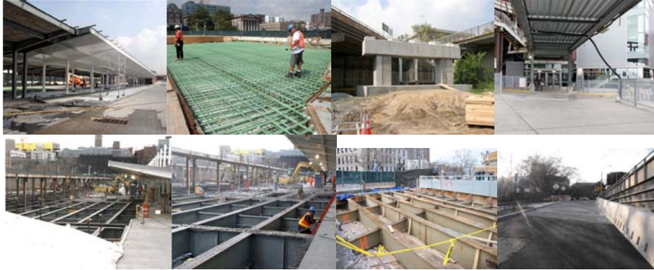
August 2011: Bus Ramp A Canopy. Span 1 – Looking North. North Ramp Center Pier. December 2011: Breezeway. Bus Ramp D. Taxi Ramp. Stage II Demolition. Ramp A Open to Traffic.
