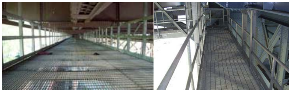
Ed Koch Queensboro Bridge Lower Level Flooring System Catwalk under Lower Level Queens Approach. Manhattan Bridge Brooklyn Tower Catwalk. (Credit: NYSDOT)
