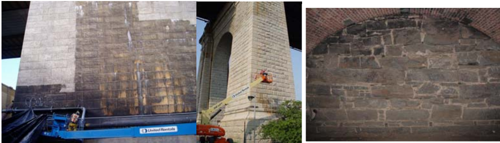
Cleaning the Masonry of the North Face of the Manhattan Bridge's Brooklyn Anchorage and of the North and East Faces of the Roosevelt Island Pier of the Ed Koch Queensboro Bridge. Masonry of the East Drive Bridge Over Eastwood Arch.
