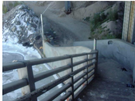
Stairs at end of pathway - closed off
