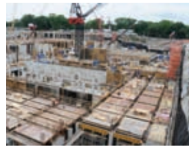
Croton Water Filtration Plant
