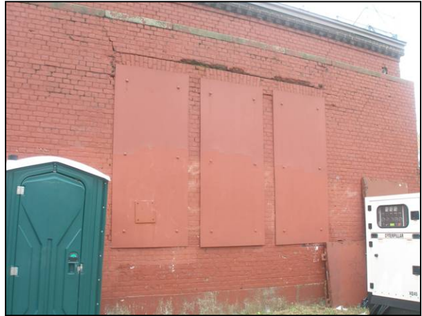
McCarren Play Center filter house: north façade of northern filter house building, looking southwest.
