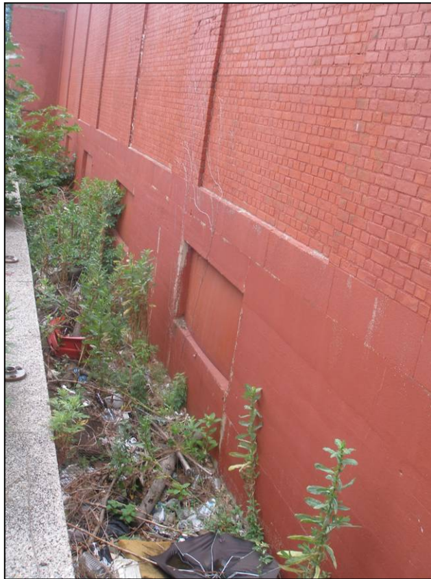
McCarren Play Center filter house and bleacher area: east facade and exposed basement wall of filter house, looking south. Photo: Kathryn Horak, 2007
