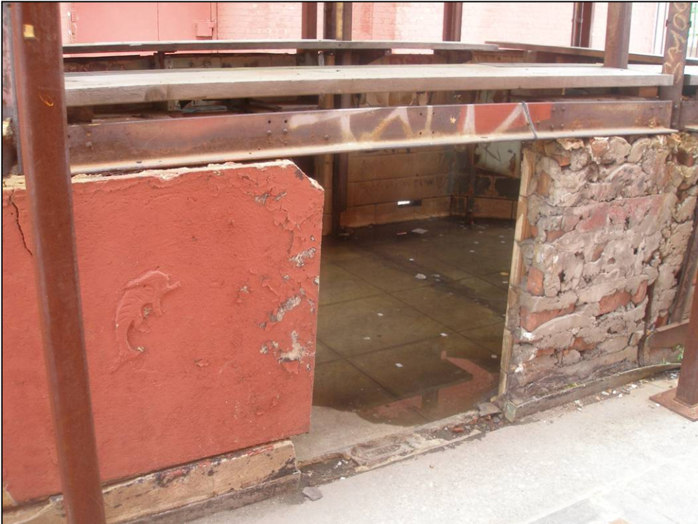
McCarren Play Center bath house: ticket booth detail, north elevation. Photo: Kathryn Horak, 2007
