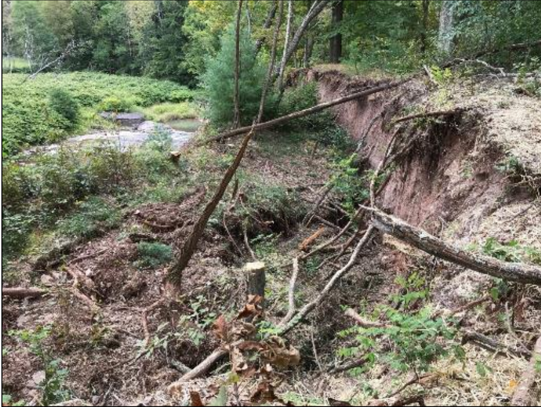
Figure 5. Rotational slide in process with the massive section of earth slowly sliding down the slope towards the Batavia Kill within the 2021 Project 2 reach.
